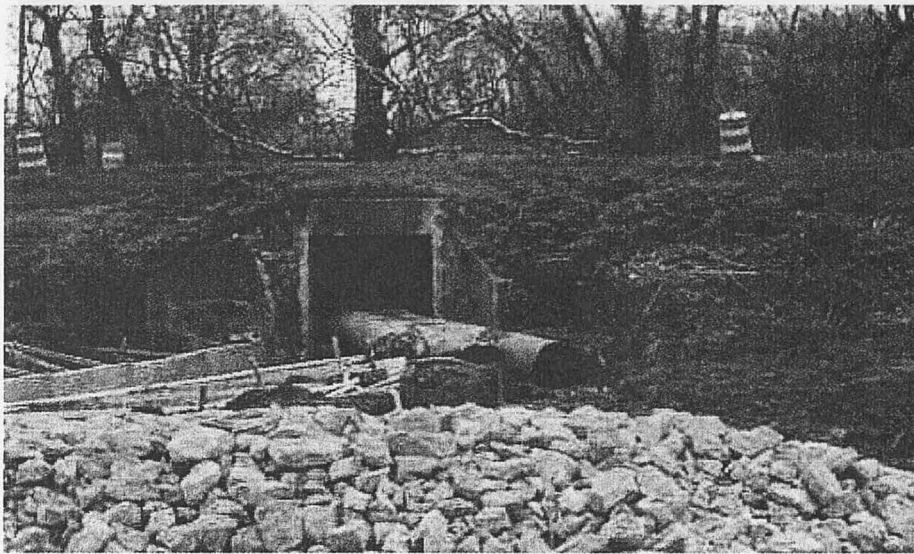
A water channel change combining multiple water channels performed to allow for a single culvert installation to minimize and control erosion
