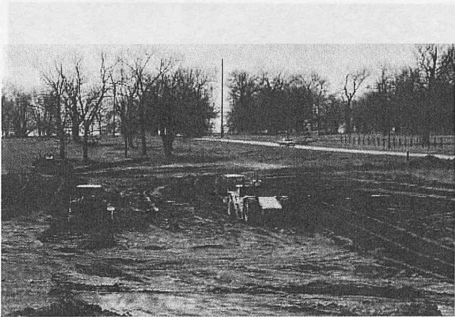
The original topsoil, Marnie silt loam, was stripped, stockpiled and returned to the original 1 to 1½ foot thickness
