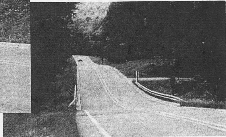
Discontinuous curb and gutter and guard rail section on Route 215.
