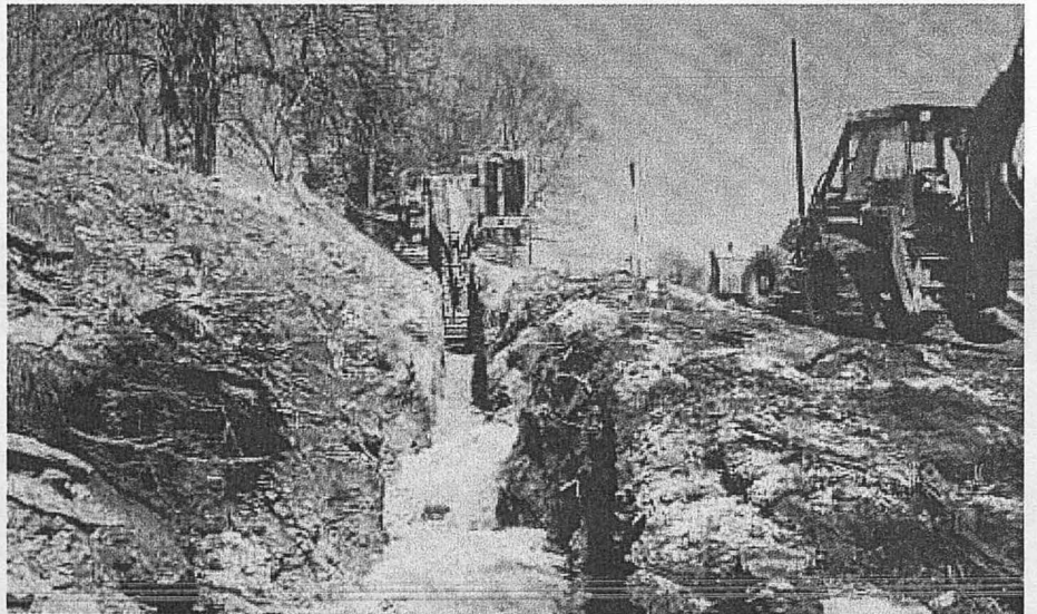
Utility easement modifications were coordinated to lessen impact on trees and overall aesthetics of the countryside
