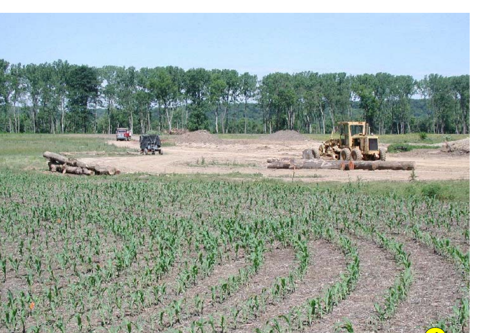
New subdivision construction near the Ohio River along Ky. 322 is indicative of the tremendous population growth in Oldham County. Farmland and pasture land is rapidly succumbing to residential development. Photo by Stephen Greb, Kentucky Geological Survey.
