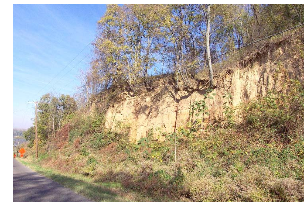
Landslides and slumps are associated with tall bluffs during strong earthquakes. The bluff pictured above is located just south of Columbus-Belmont State Park on Ky. 58. The bluff is capped by approximately 30 feet of loess (windblown material). Photo by Glynn Beck, Kentucky Geological Survey.
