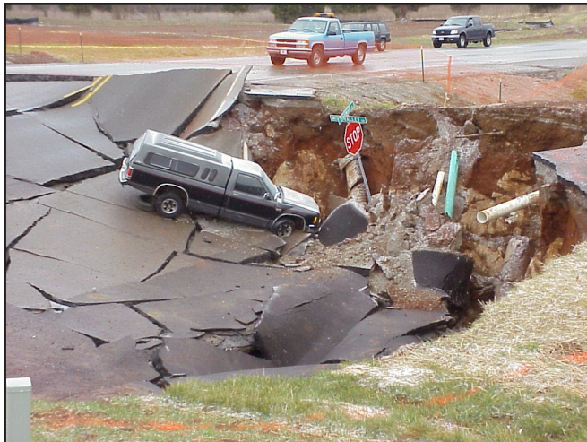
Figure 3. By chance, the collapse at Dishman Lane in Bowling Green did not cause any fatalities.
