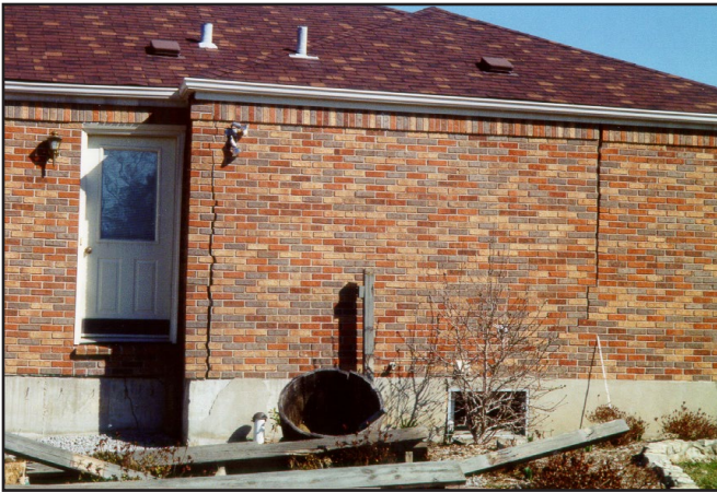
Figure 2. A cover-collapse sinkhole caused more than $40,000 in damage to a home near Louisville in April 2001.
