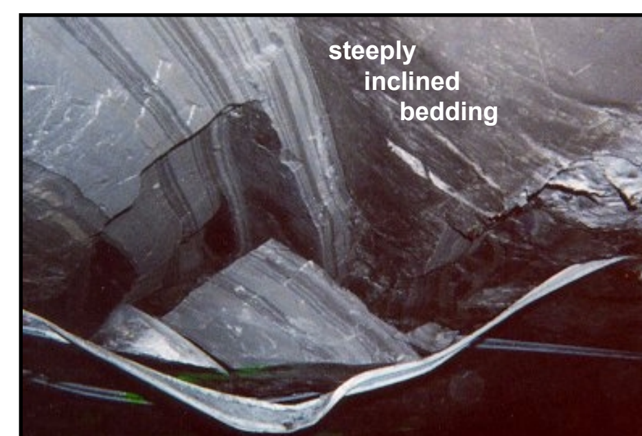
Figure 14. Roof fall exposes steeply dipping beds.
