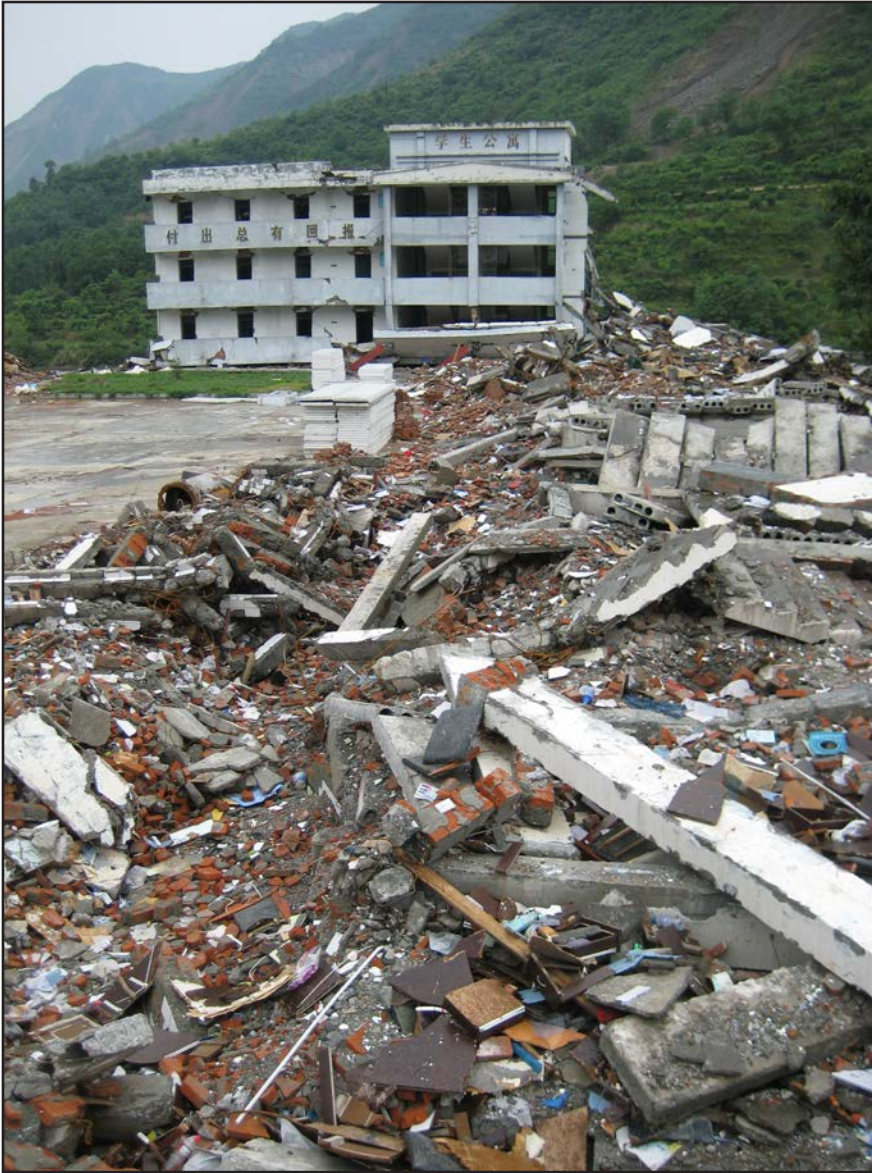
Figure 1. Strong ground motion from the Wenchuan earthquake caused a classroom building to collapse and killed many students.
