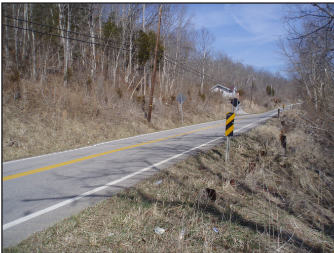
Figure 11. An old I-beam pier retaining wall in the grass suggests previous slope failure, and a leaning telephone pole suggests the slope is actively creeping.
