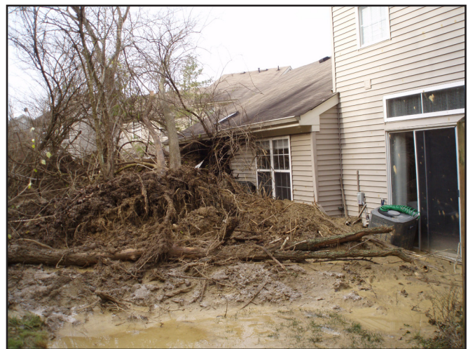
Figure 19. A large translational slide in December 2011 brought debris downslope into two condominiums. The greater slope area was predicted by LiDAR beforehand.
