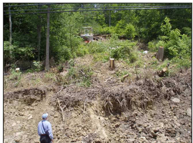
Figure 4. Landslide along Ky. 3187. Thick colluvium is shown at the bottom of the photo and a threatened home toward the top.
