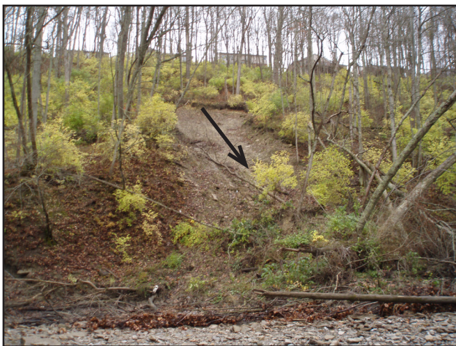
Figure 18. A small translational slide in November 2011 is indicated by debris and leaning trees at the toe and the neighborhood above the scarp. The greater slope area was predicted using LiDAR beforehand.
