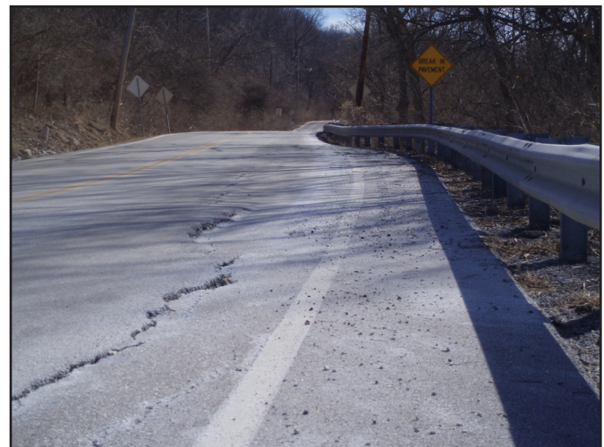
Figure 12. Evidence of landslide activity: The road is benched into the middle of the slope and the landslide stretches above and below the road. There is significant offset in the pavement.
