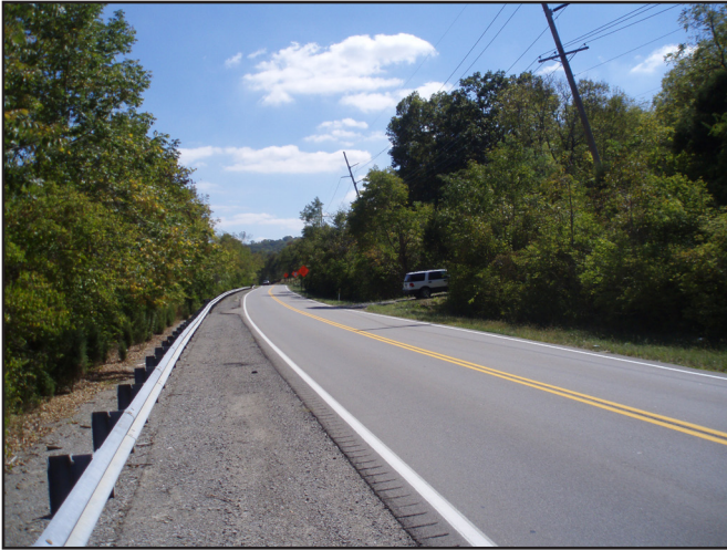
Figure 13. Recently repaired I-beam piers and leaning telephone poles along Ky. 8 are evidence of landslide activity. Ky. 8 is in constant need of repair because of landslide damage.
