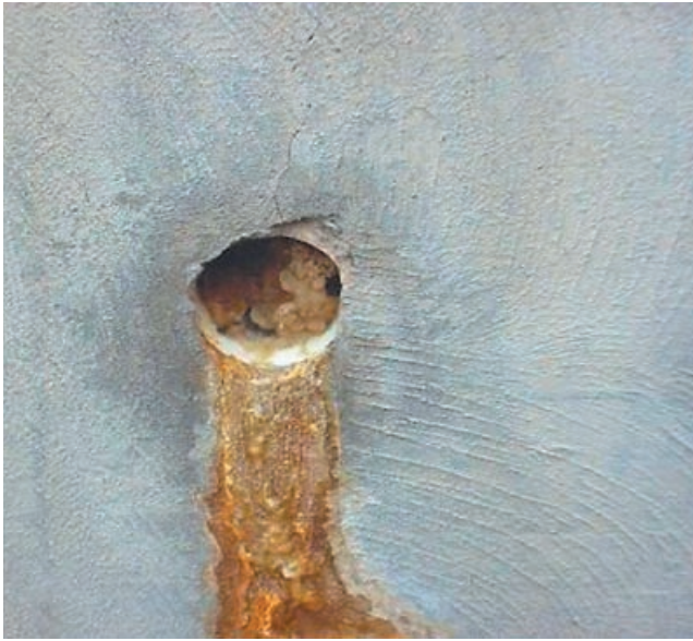
Figure 20. Drain-pipe precipitates (sulfates).
