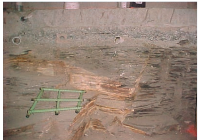
Figure 16. Multidirectional cleat fractures coated with secondary sulfate precipitates such as jarosite, copiapite, and melanterite in the Chattanooga Shale beneath flooring at the middle school. The sewer drain tile was broken by heaving floor slabs, and subsequently was removed. Rebar is being inserted into reinforced concrete columns.
