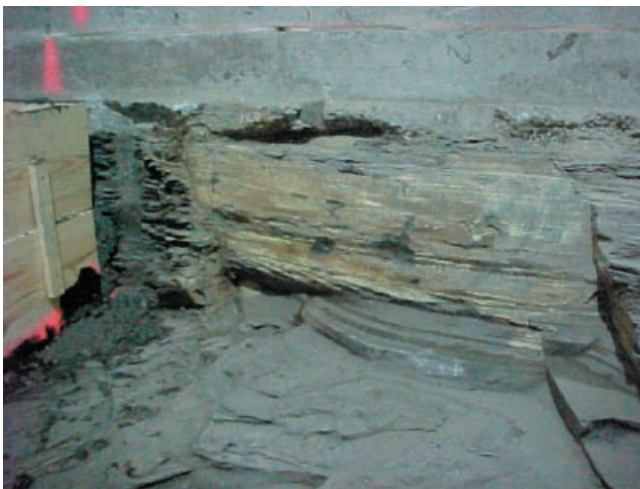
Figure 18. Cleats with sulfate precipitation in shale subcrop beneath the middle school, along with forms for construction of new concrete columns.
