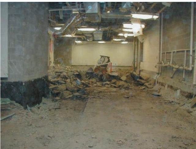
Figure 14. Repair of heaving floors in middle school gymnasium. The original foundation and fill had to be removed and sealed with a resin to prevent further oxidation and heaving of the shale. Photograph by John F. Stickney, Kentucky Rural Water Association.
