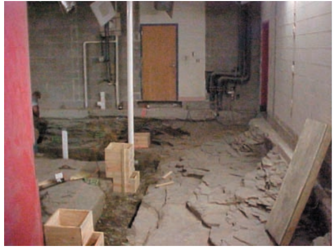
Figure 15. New trench constructed in shale subcrop beneath the middle school. The sulfate mineral copiapite has formed in cleats. Note that load-bearing walls on the right side of the photograph and in the background do not show any signs of failure.
