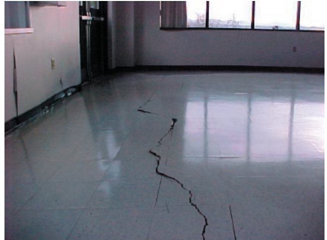
Figure 21. Substantial floor cracks in Carhartt break room.
