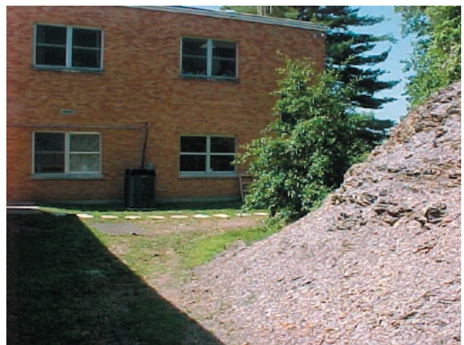
Figure 25. Exterior of the Marcum and Wallace Hospital office wing and outcrop of the Cleveland Member of the Chattanooga Shale. Note the absence of cracks or offsets in exterior brickwork near windows, even though behind these windows, interior floor heaving was extensive.
