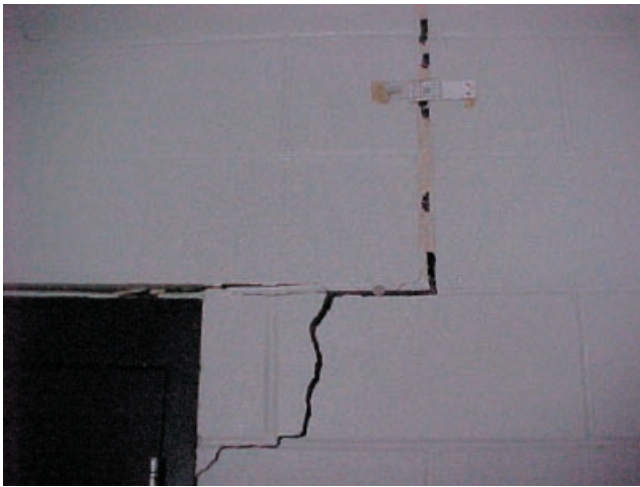
Figure 22. Large cracks (1 in.) in concrete block adjacent to doorway at Carhartt factory.
