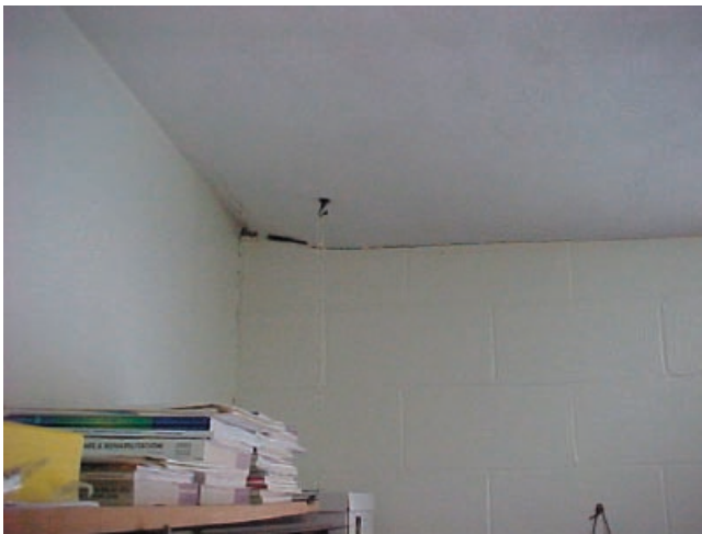
Figure 27. Displacement of ceiling wallboard at hospital along nonload-bearing walls caused by floor heaving.
