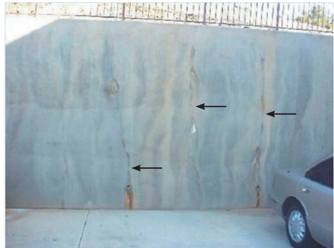
Figure 19. Tension fractures (arrows) along exterior retaining wall and iron-stained drainholes.
