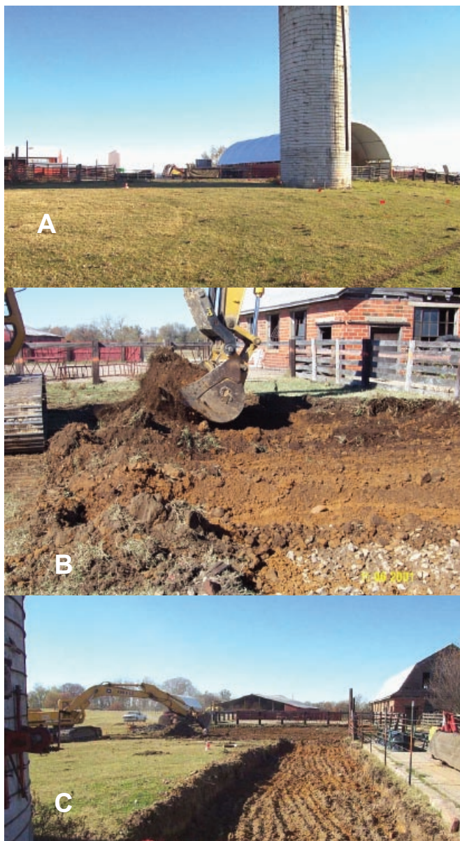
Figure 4. (A) The abandoned feedlot before excavation began, looking northeast. (B-C) During excavation, both looking west. (B) shows the area where the soil was excavated to 1 ft below land surface. The foreground area in (C) was excavated to 3 ft below land surface.
