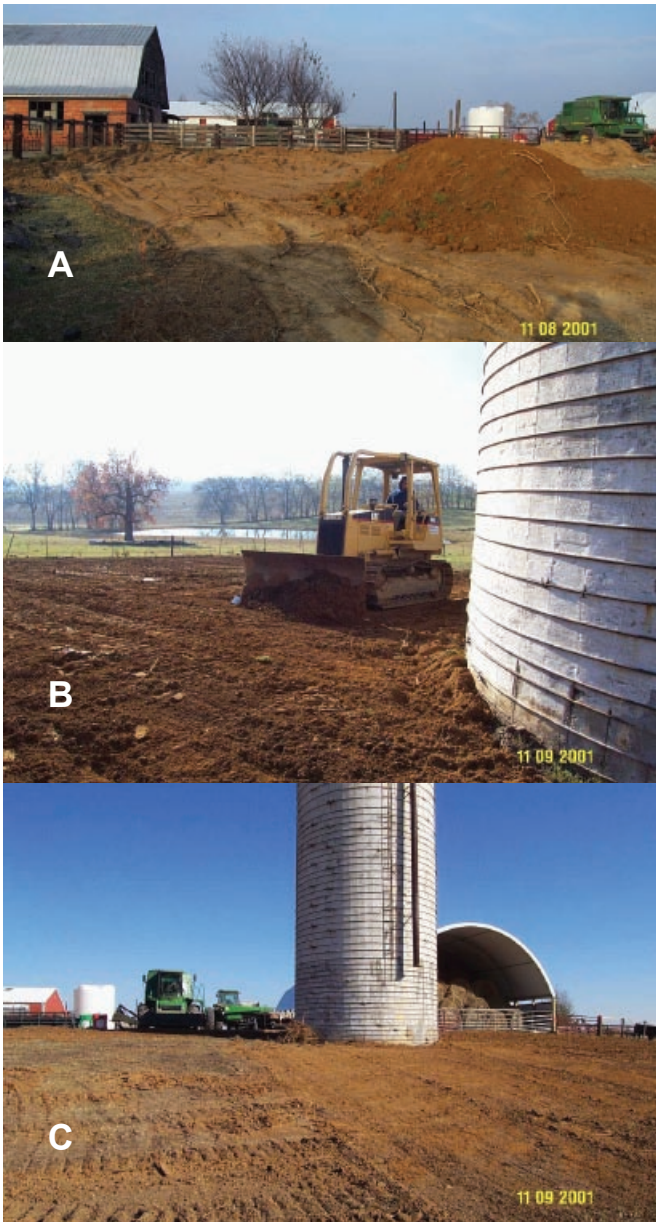
Figure 6. (A) The excavated feedlot being filled with native soil, looking north. (B) Soil being spread back to original grade (looking southwest). (C) After remediation was completed, looking northeast.
