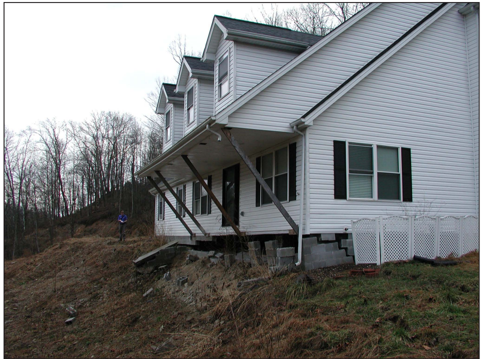
Figure 6. Landslide-damaged home, Lawrence County.
