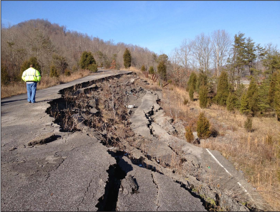
Figure 1. Landslide damage along the now abandoned Ky. 10, Lewis County.
