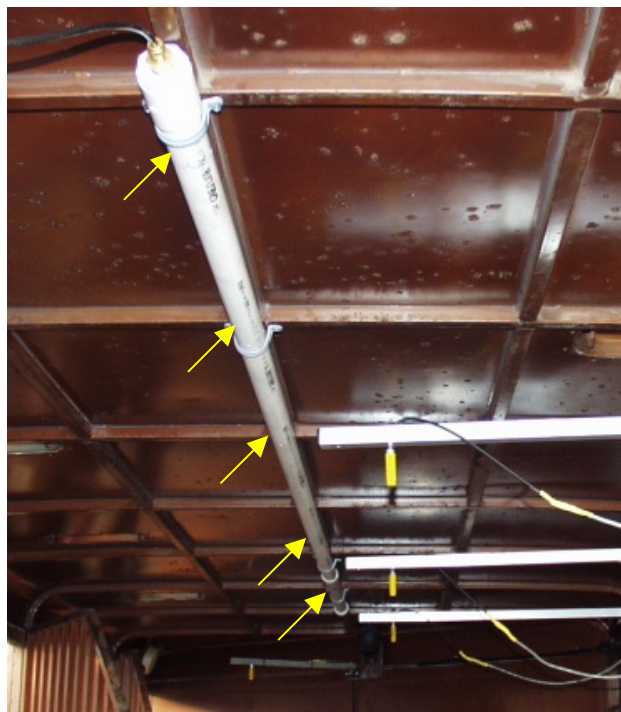
Figure 3. PVC diffuser for injection of tracer gas. Arrows indicate approximate locations of outlet holes.
