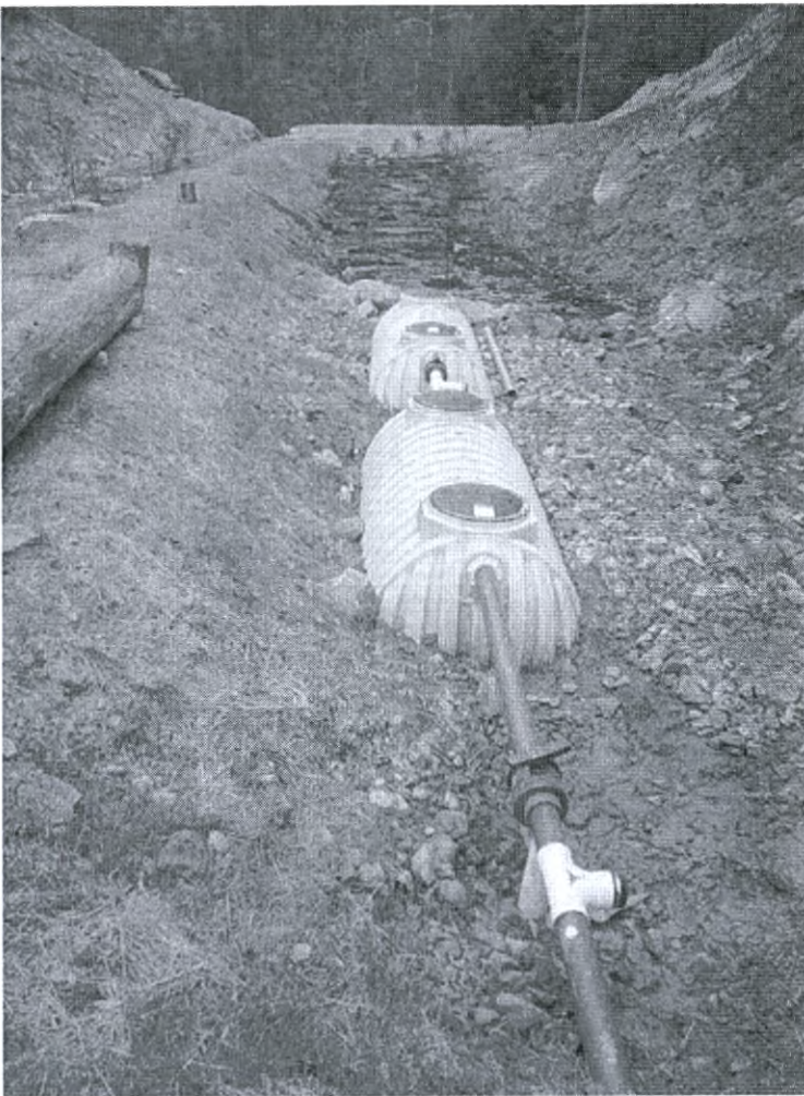
Figure 4. Picture of the bioreactors installed at Guy Cove. The picture shows the progression of the seepage through the bioreactors and to the wetland.
