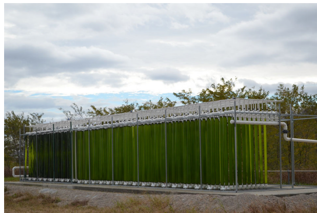
Fig. 4 Photobioreactor installed at East Bend Station
