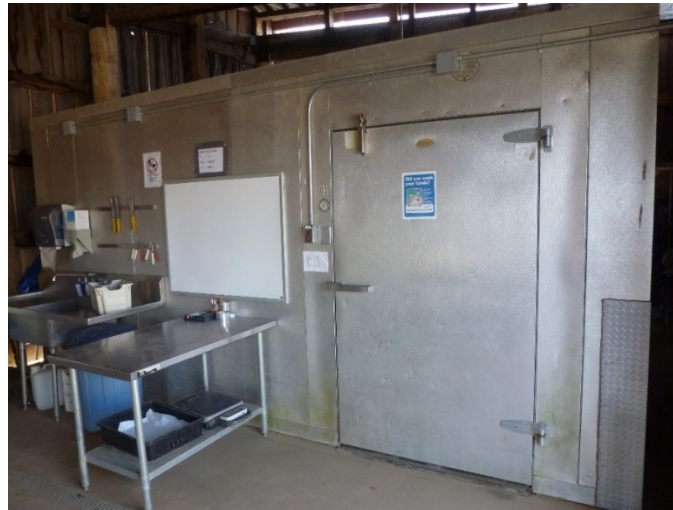
Figure 5-3 CSA walk in cooler
