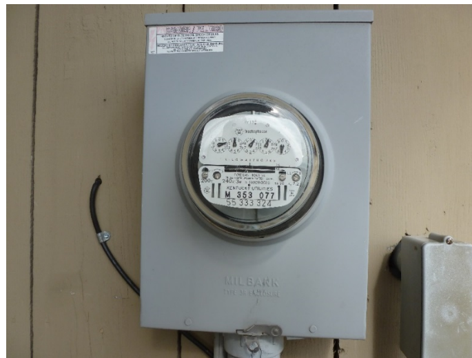
Figure 5-2 CSA conventional electric meter
