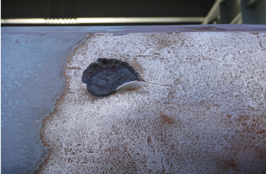
Figure 2 Scab in steel plate on bridge tie chord
