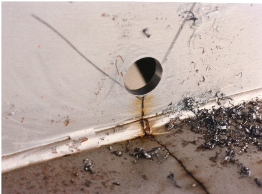
Figure 59 A check hole used to stop further fatigue crack growth in a fascia girder
