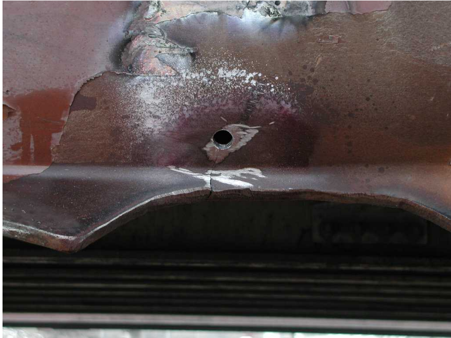
Figure 5 Crack caused by vehicle impact (Asfour, S., Emergency Bridge Repairs, Presentation at the Midwest Bridge Working Group Meeting, Evanston, IL, 2005)
