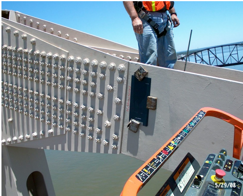
Figure 25 RT film pack mounted on outer face of inboard flange for radiograph of flange-to-web fillet weld and flange at 5-1/16" crack terminus
