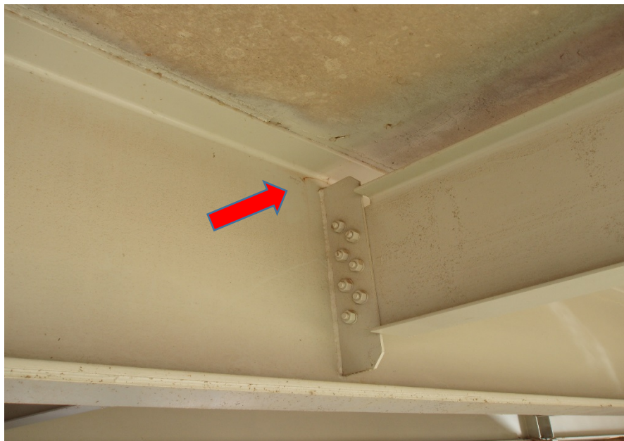
Figure 10 Distortion-induced fatigue crack in bridge beam
