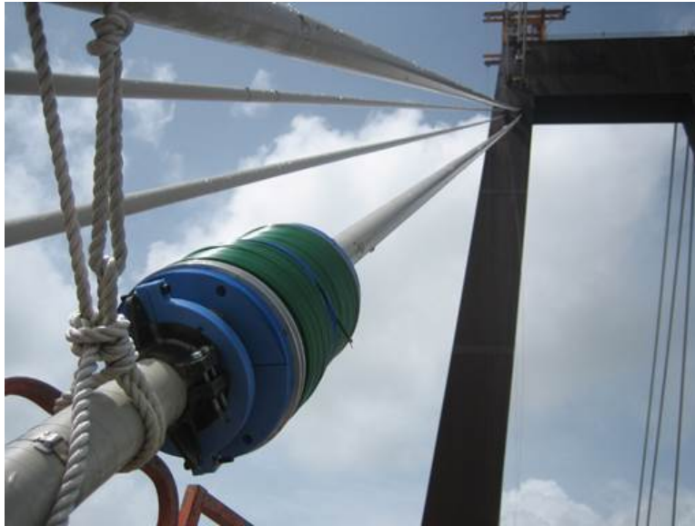
Figure 48 Magnetic flux testing of a stay cable on the I-310 Hale Boggs Bridge near Luling, Louisiana
