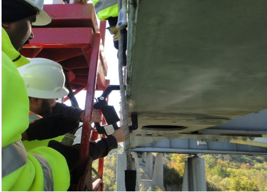
Figure 18 Use of AC yoke for magnetic particle inspection of web-to-flange fillet weld on tie-chord. The yoke is aligned to detect a crack in the toe of a longitudinal web-to-flange fillet weld on the tie chord
