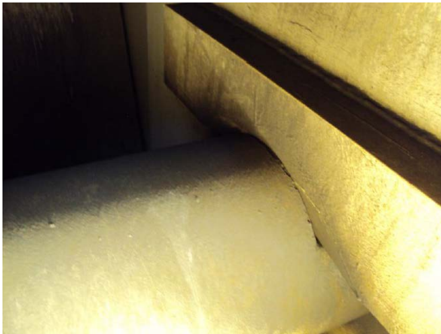
Figure 8 Top chord plate wearing groove into a top chord pin on the K-65 Kennedy Bridge over the Ohio River at Louisville
