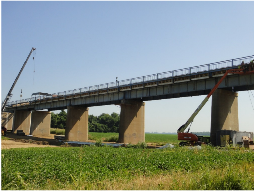
Figure 3 Simple span non-redundant deck girder approach spans that are fracture-critical
