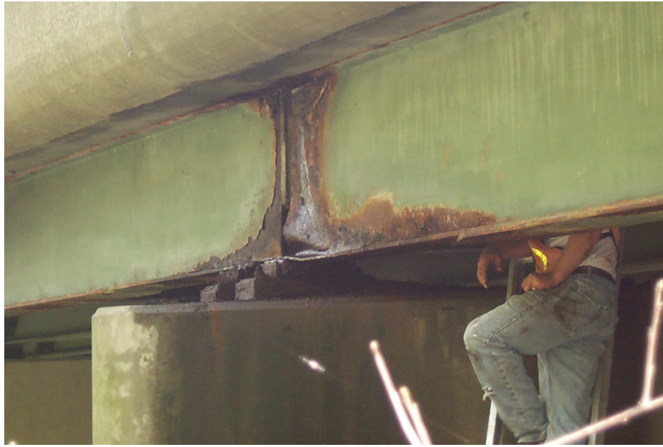
Figure 9 Web crippling of a corroded girder
