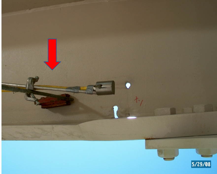
Figure 24 Upward view showing RT guide tube and collimator aimed at 5-1/16" crack in H-beam web for radiograph from underside of flange (arrow)
