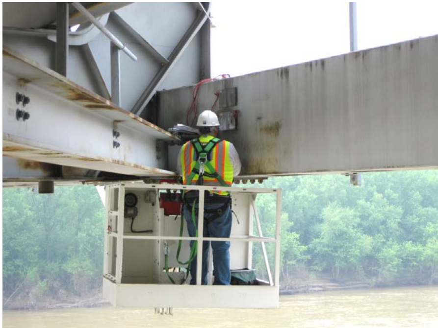
Figure 13 NDE operator being qualified using flawed plates attached to bridge tie-chord (Gorrill, G., “Sherman Minton Rehabilitation, Presentation to the Midwest Bridge Working Group, Schaumburg, IL, May 30, 2012)
