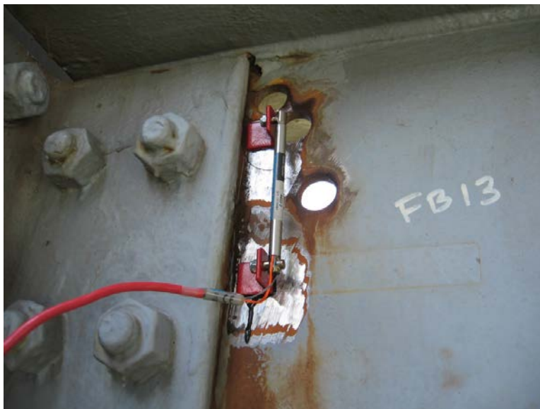
Figure 49 Crack gage mounted on bridge floorbeam
