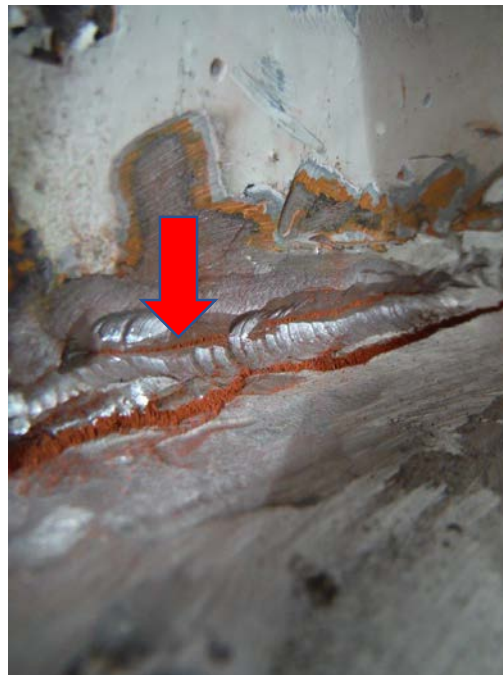
Figure 20 Possible MT crack indicated on in fillet weld subsequently evaluated by UT
