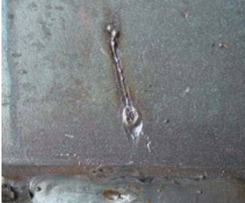
Figure 11 Welding arc strike on surface of steel plate (Heavy Engineering Research Association, Auckland, NZ.)
