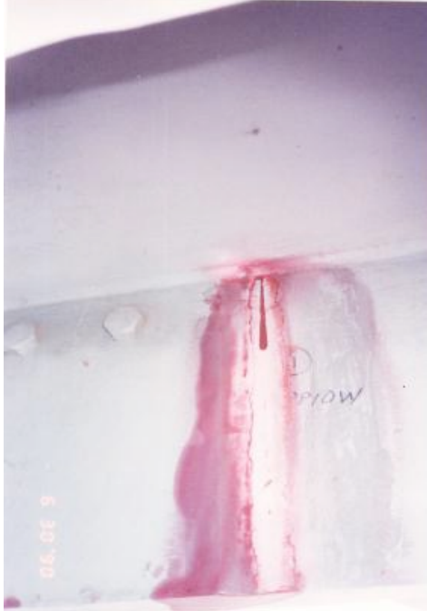
Figure 54 Crack in H-girder (high strength steel) on I-65 Kennedy Bridge 22-1/2 long x 3/8” deep (HNTB, “Bridge Inspection Report: I-65 BRIDGE over the Ohio River,” Report to the Commonwealth of Kentucky Transportation Cabinet, Department of Highways, Division of Maintenance, May 1991).
