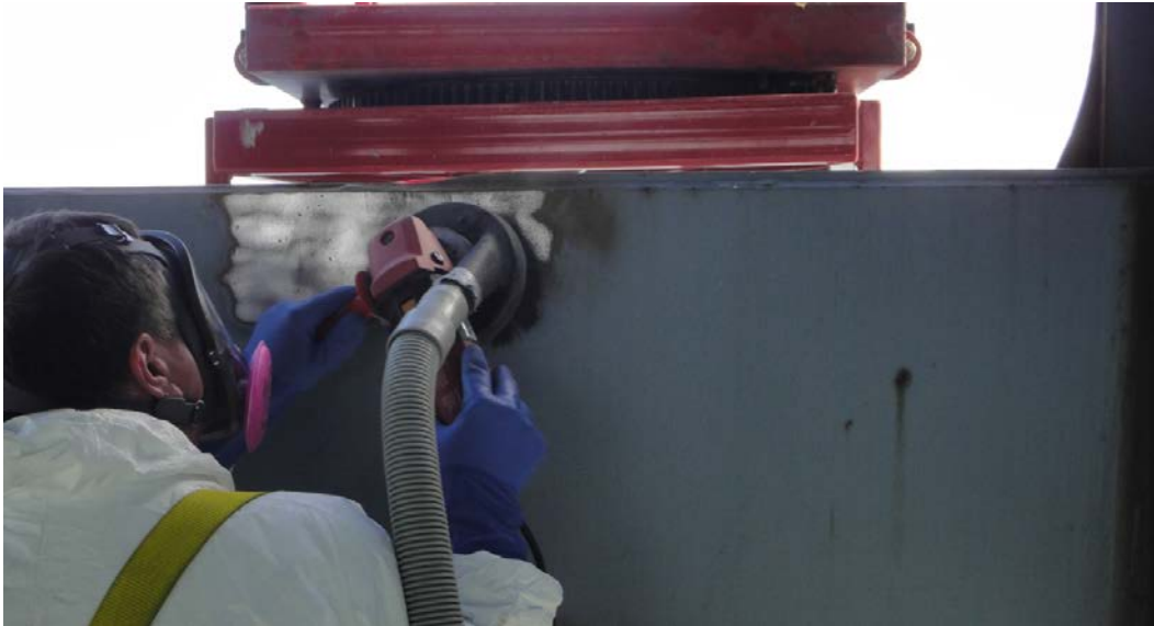
Figure 50 Technician removing lead-based painting using vacuum shrouded grinder with non-woven pad and wearing personal protection
