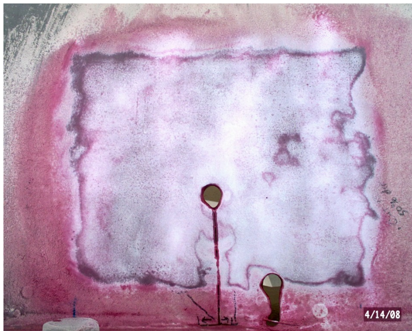
Figure 17 Dye penetrant test on cracked area on faulty weld repair of upper chord member
