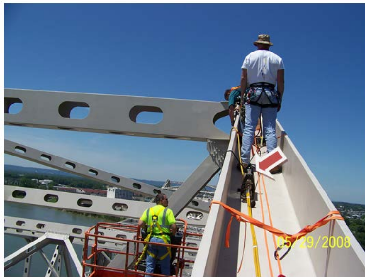
Figure 23 RT Projector (Arrow) mounted on H beam. Note yellow guide tube running from camera to location under the beam
