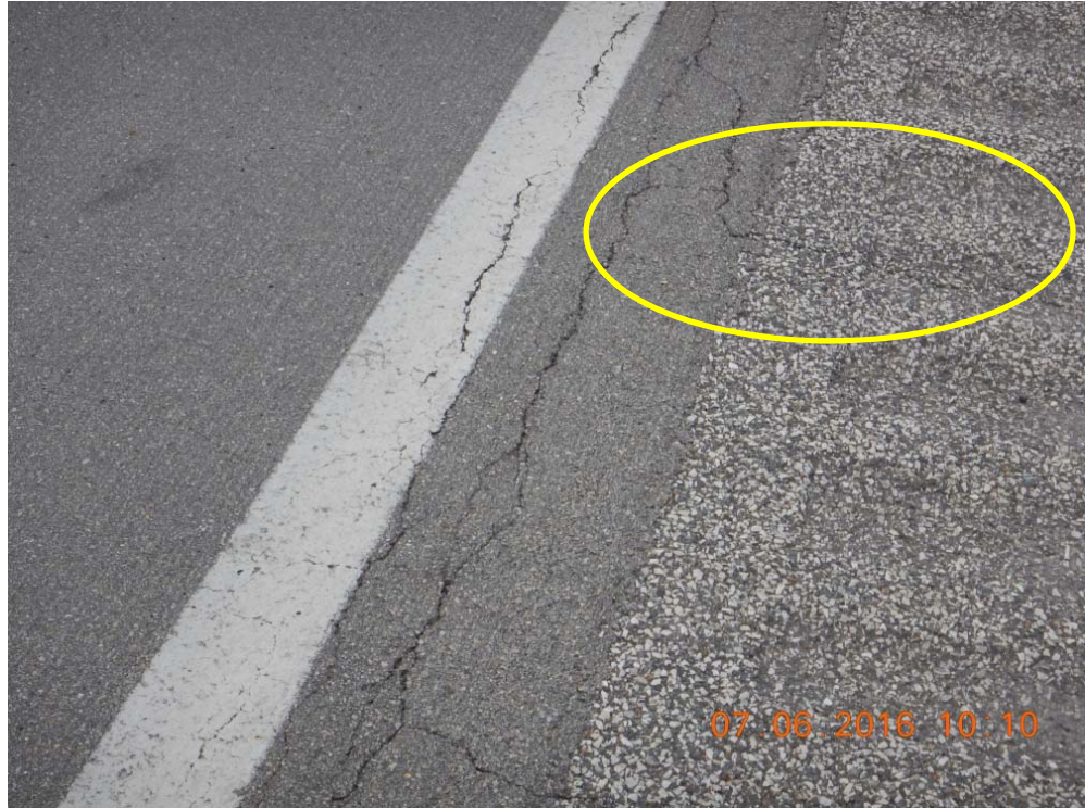
Figure 7.4: Greenup County, Reflective Crack/Edge Cracking, Microsurfacing
