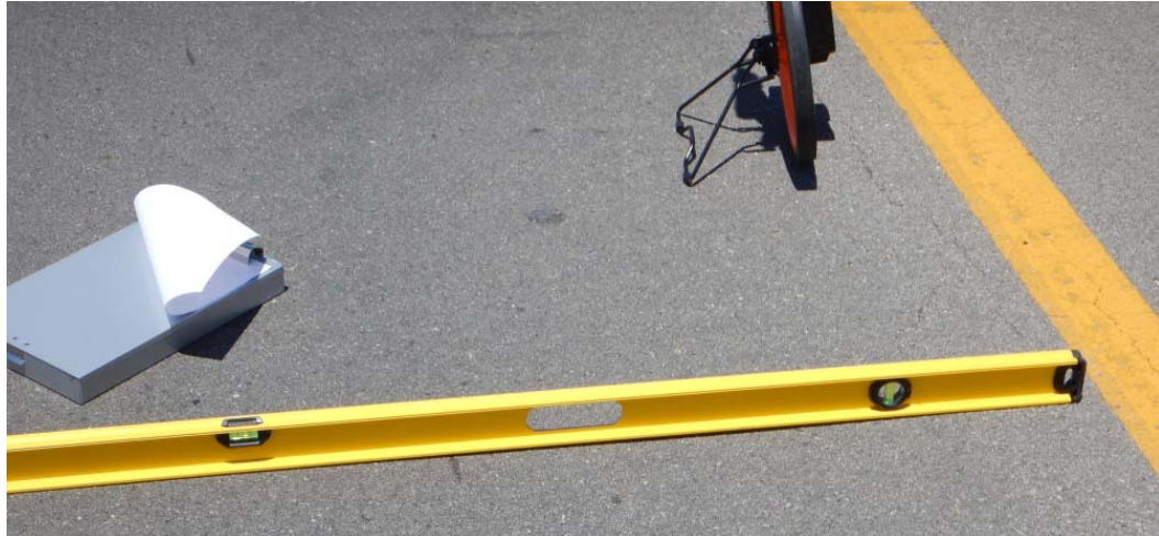
Figure 7.11: Nelson County, Rutting, Microsurfacing
