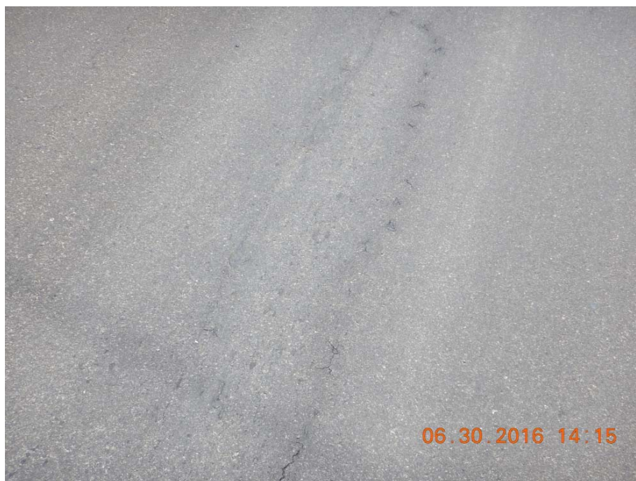
Figure 7.2: Morgan County, Bleeding Distress, Brand New Surface
