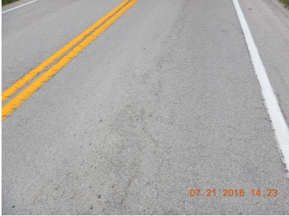
Figure 7.7: Wayne County, Alligator Cracking, Thinlay
