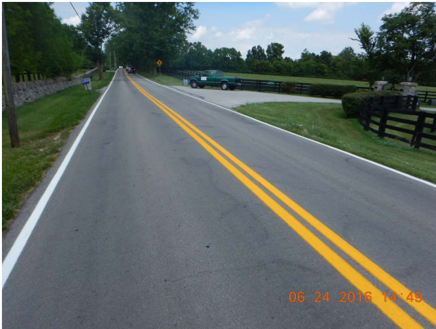
Figure 7.1: Fayette County, Bleeding Distress
