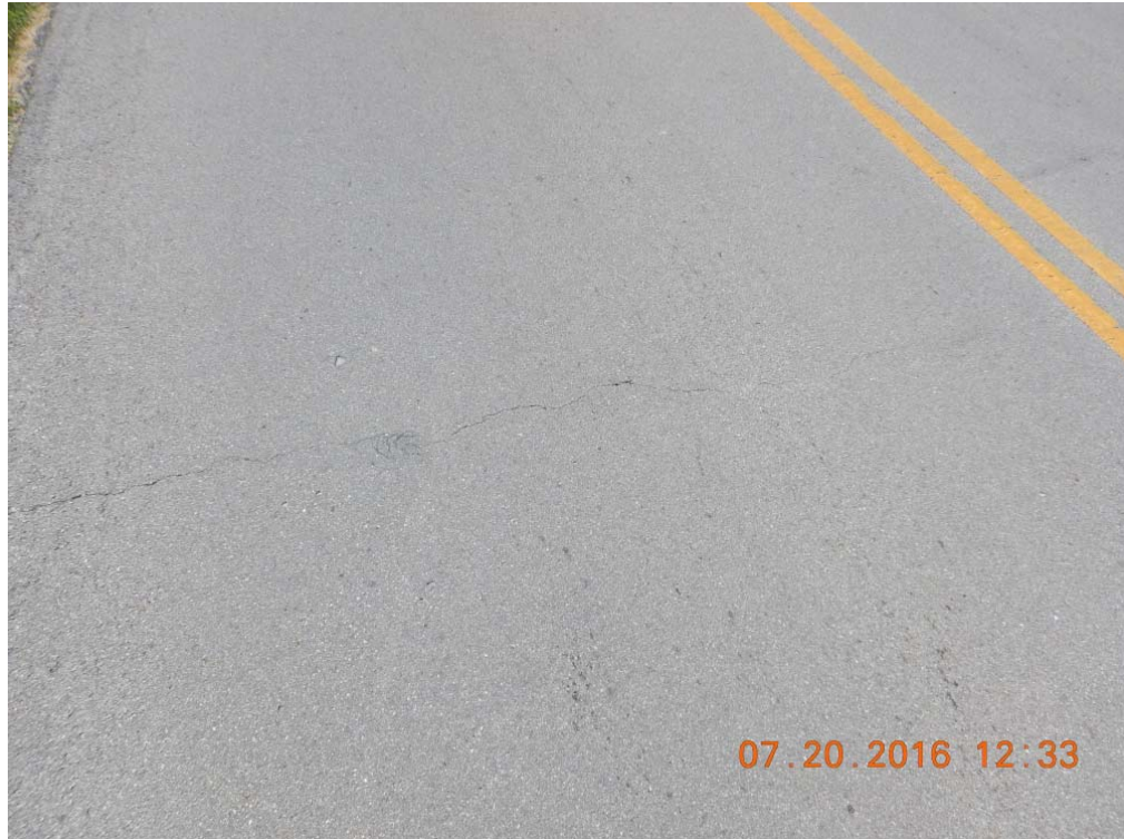
Figure 7.6: Laurel County, Transverse Cracking, Microsurfacing
