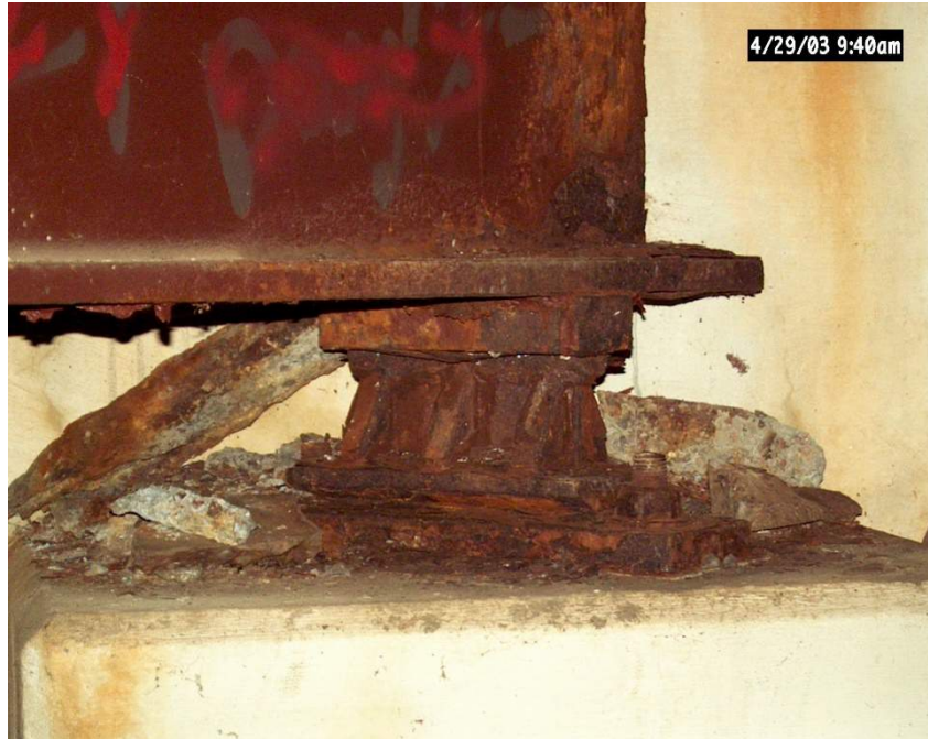
Figure 3. Corroded UWS Bearing Under Leaking Joint
