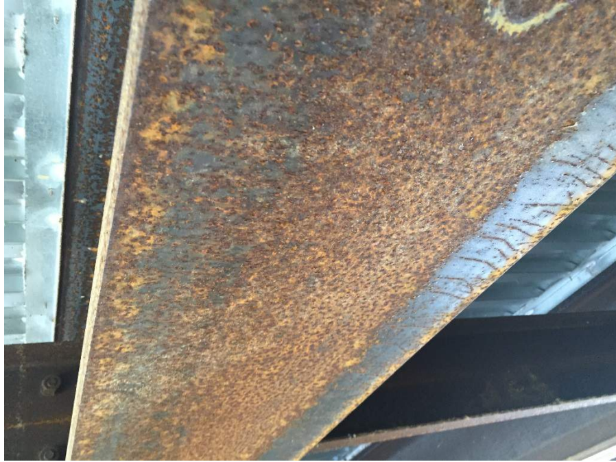
Figure 15. Pitting on Lower Flange of UWS Steel Beam Caused by Presence of Mill Scale on KY 6 Bridge
