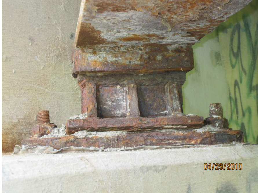
Figure 23. Rocker After Scaley Corrosion Product Removal on KY 1893 Bridge at Shawhan, KY
