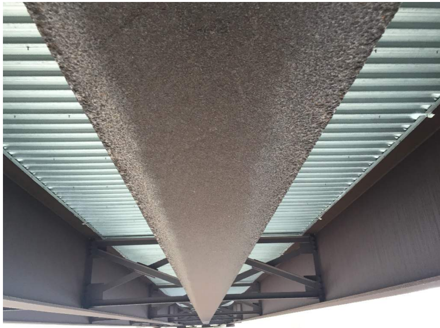
Figure 24. Scaley Corrosion on Bottom Face of Girder Flange of I-75 Overpass Bridge
