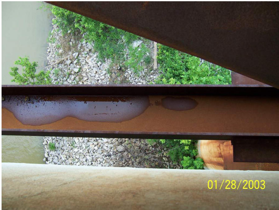
Figure 32. Water Ponding on Lower Chord of KY 81 Bridge
