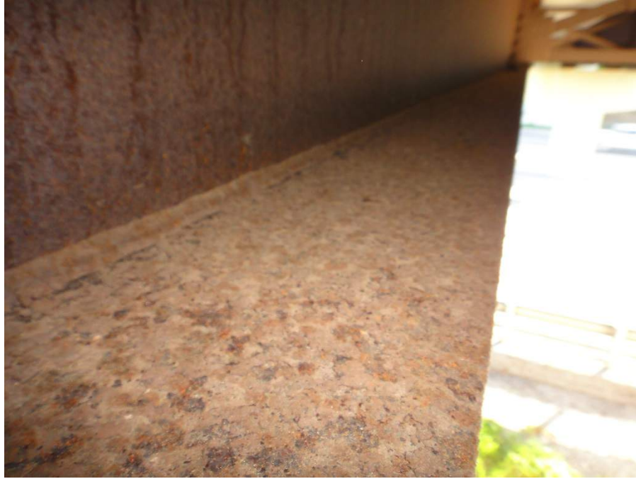
Figure 25. Scaly Corrosion on Upper Flange of Lower Flange on I-75 Overpass Bridge
