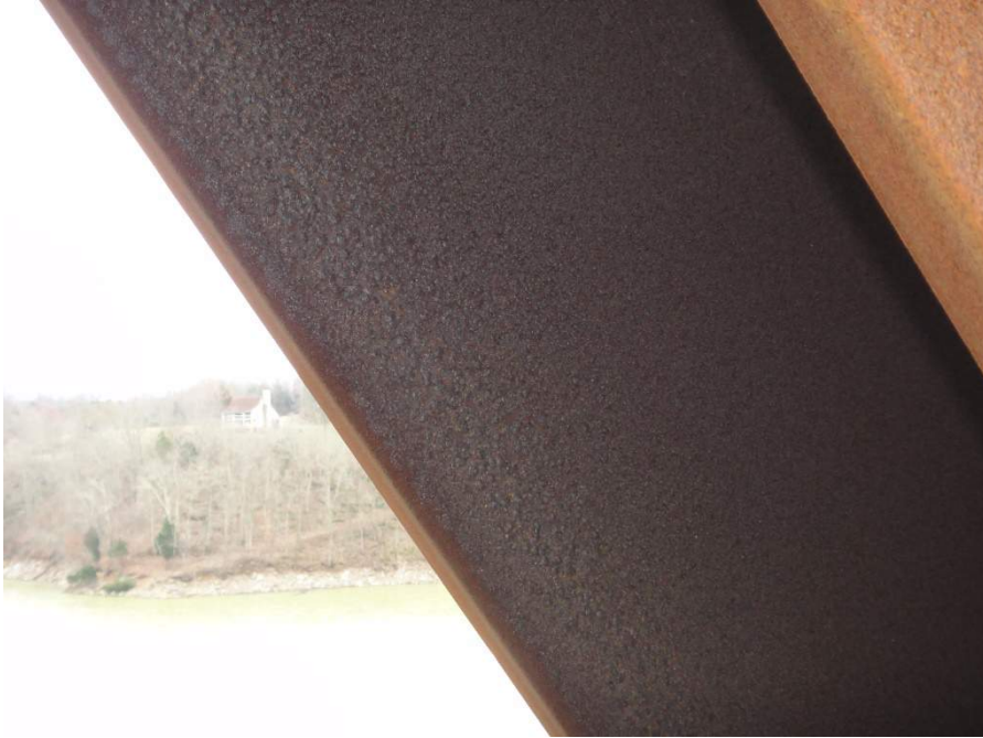
Figure 5. Underside of Truss Diagonal Showing Coarse Rust on KY 90 Bridge
