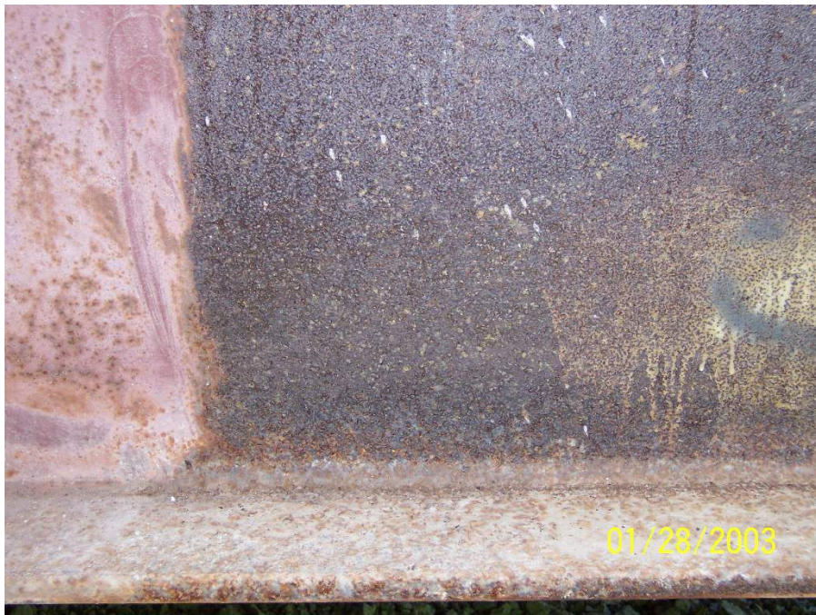
Figure 18. UWS Beam Showing Failed Coating at Beam End. Note the Severe Pitting in Coating and on Adjacent UWS.
