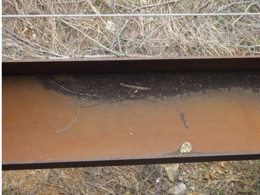
Figure 35. Debris Collected on the Lower Chord of the KY 90 Bridge
