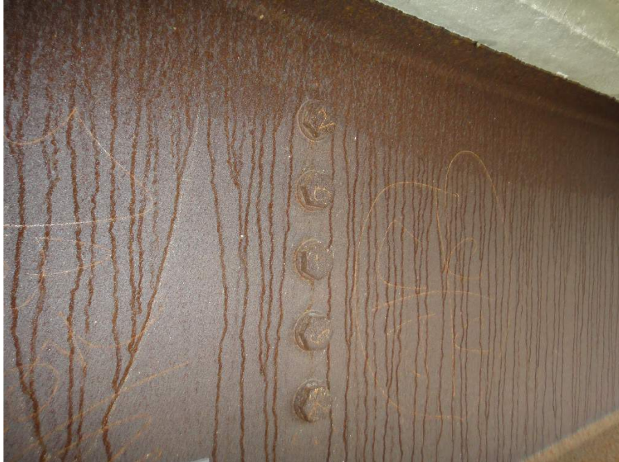
Figure 13. Condensation Drip Marks on Web of KY 90 Approach Span
