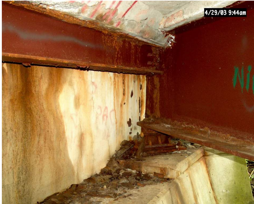
Figure 21. Corrosion under Deck Joint on KY 1893 Bridge at Shawhan, KY
