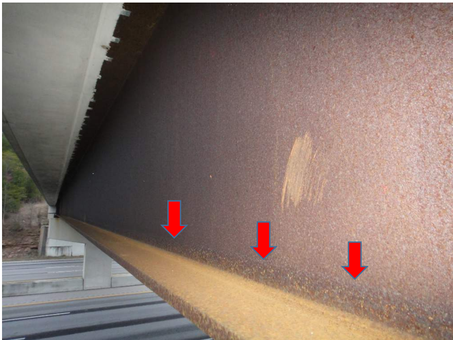
Figure 4. Fascia Beam of I-75 Overpass Bridge Showing Tight Rust in Middle of Web (Scrape Mark) and Scaly Corrosion and Rust Capillary Action on Lower Portion of Web (Arrows)
