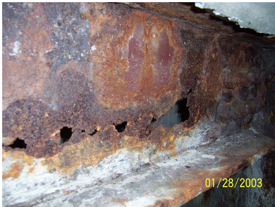
Figure 2. Severe Loss of Section on Web of Weathering Steel Diaphragm
