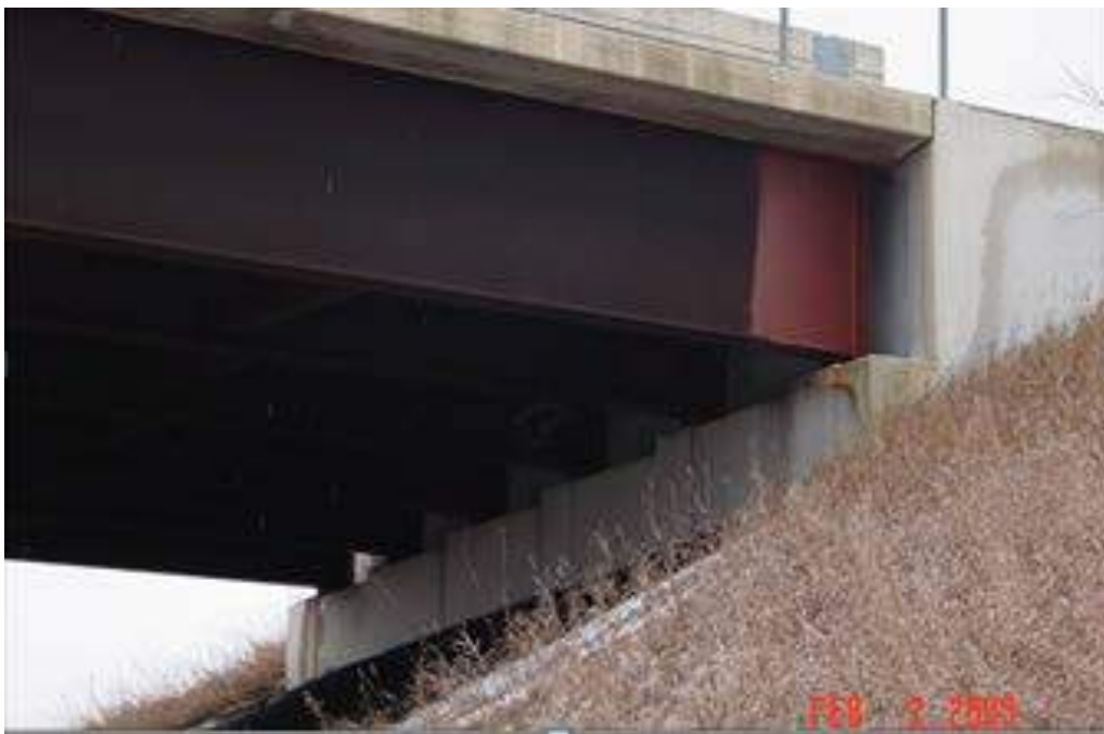
Figure 16. Minnesota DOT UWS Girder Painted about Two Feet from End
