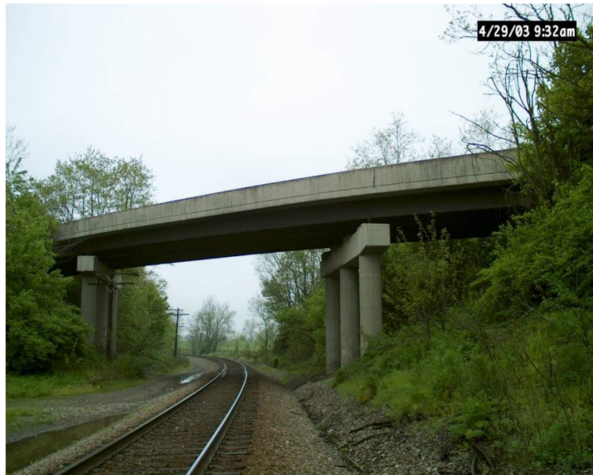
Figure 30. Vegetation Build-Up Around Abutments of KY 1893 Bridge
