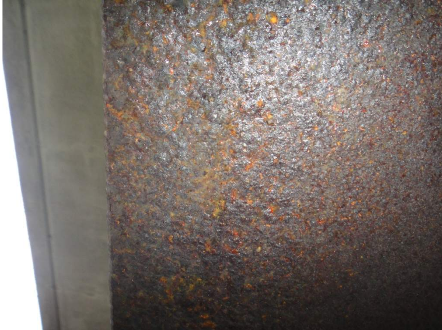
Figure 9. Coarse Patina on Lower Face of Lower Flange of I 75 Overpass Bridge
