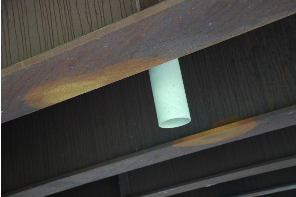
Figure 7. UWS Girder Bridge (Non-KYTC Bridge) Showing Effect of Inadequate Drain Pipe Clearance on Patina Formation
