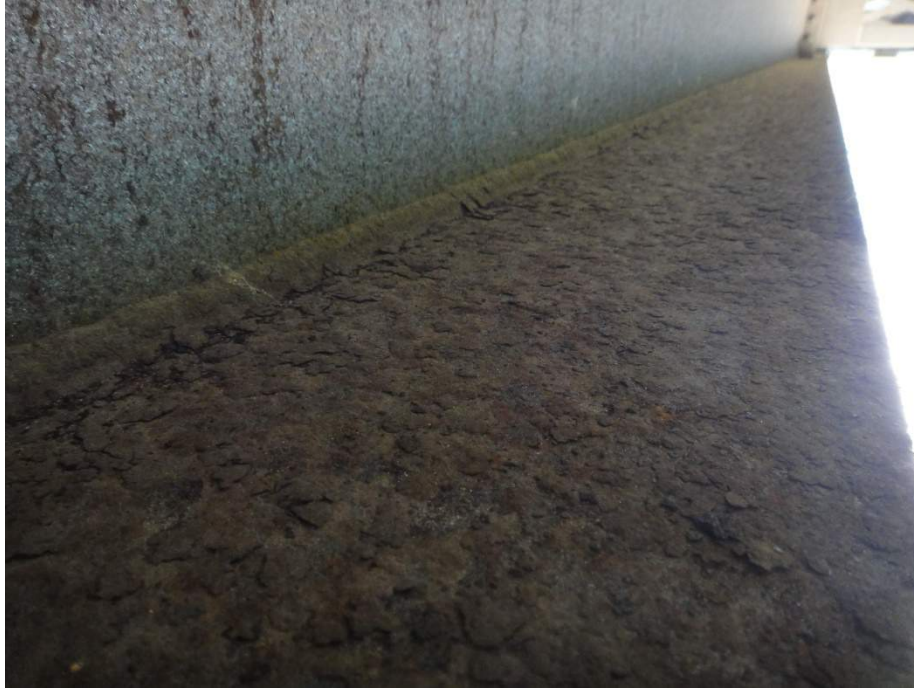
Figure 11. Unhindered Corrosion on Upper Face of UWS Girder on I 75 Overpass Bridge
