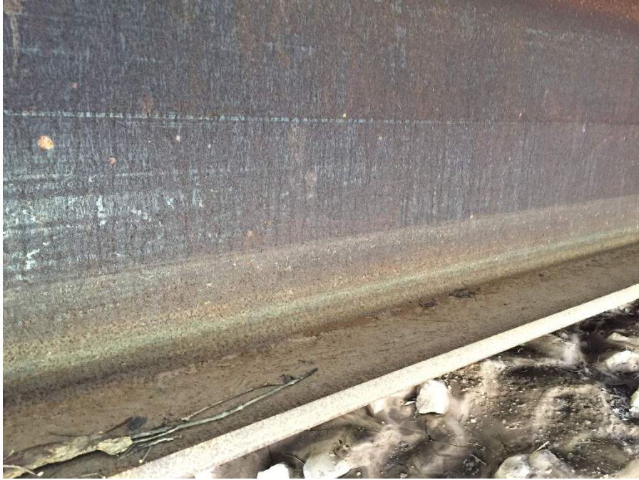
Figure 27. Tide Marks on the Web and Debris Deposits on the Flange of a UWS Beam of the KY 6 Bridge Indicative of High Water (Overtopping)
