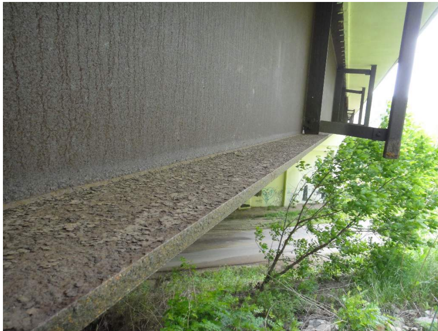
Figure 12. Deposit of Corrosion Debris on Upper Face on Girder Lower Flange of UWS Beam
