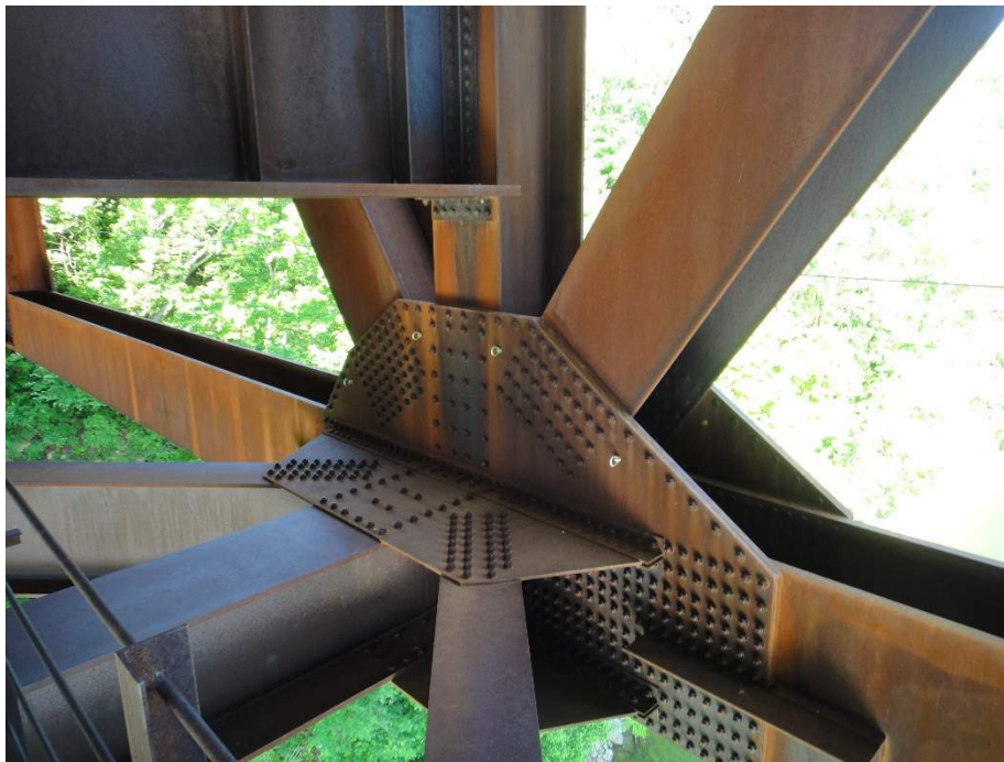
Figure 8. Lower Chord of UWS KY 90 Truss Bridge Showing Various Patina States
