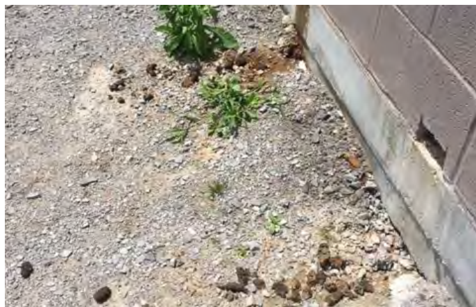
Example of inappropriate drainage from kennels onto dirt outside the shelter
