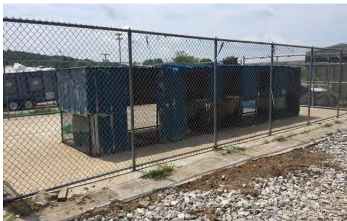
Dog holding area built with materials that cannot be disinfected; hot in summer and cold in winter
