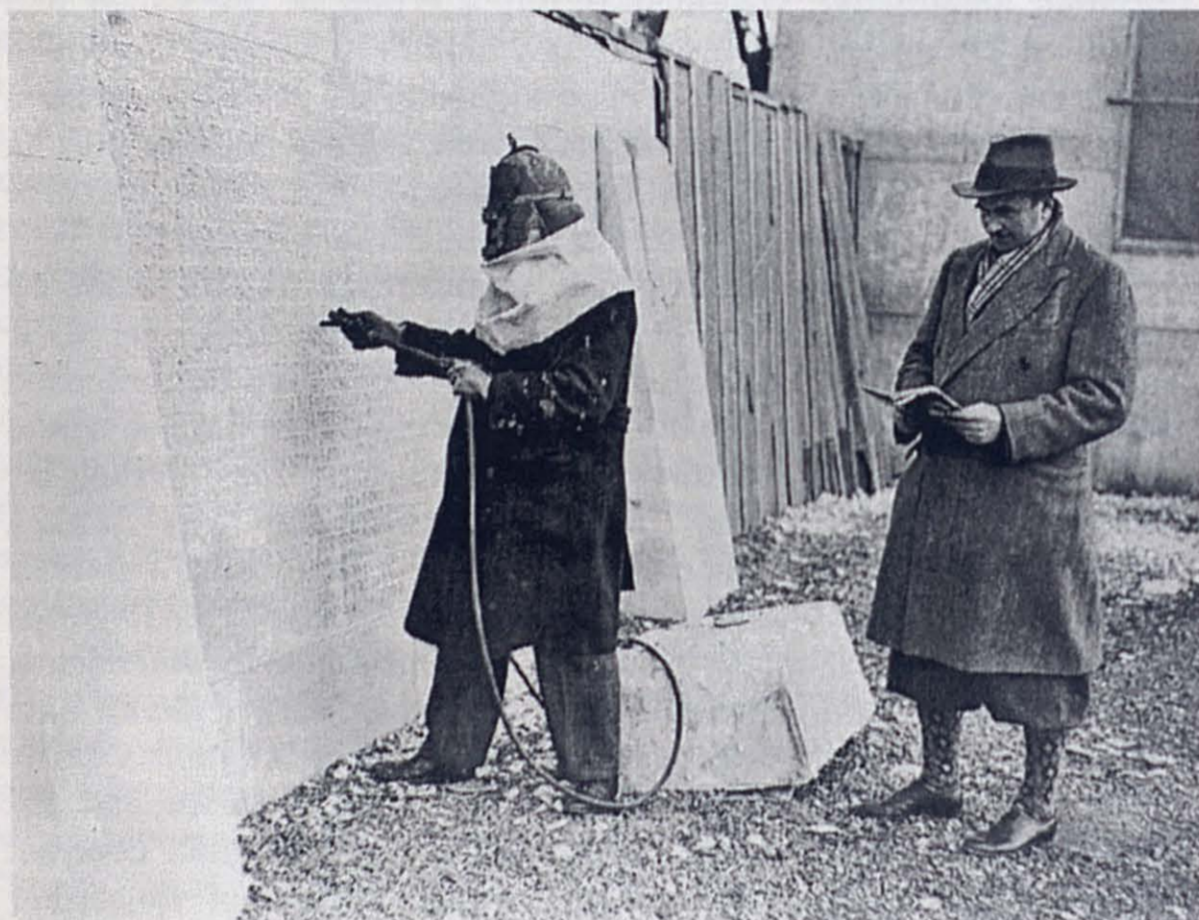
Figure 3: A sandblaster inscribes the names of the Missing on the Vimy memorial. Photo: Veterans' Affairs Canada.
