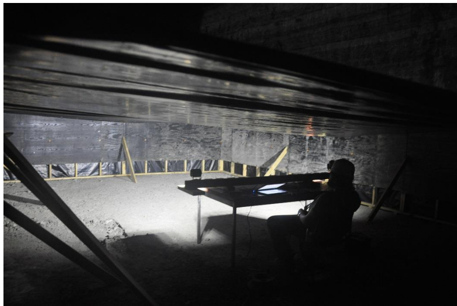
Figure 3.7: Example light setup (behind and left of roof bolt machine)
