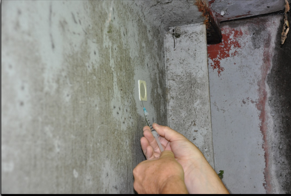
Figure 12. Extracting Initial Water Sample from Bresle Patch to Measure Surface Chloride Contamination Prior to Pressure Washing on KY 453 over P&L Railroad (B00045N).
