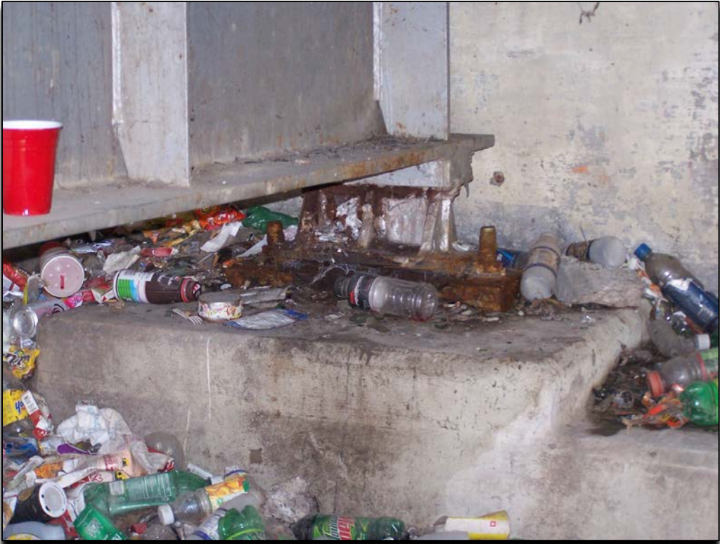
Figure 5. Trash and Roadway Debris Build-up on an Abutment. Note Corrosion on Bearing
