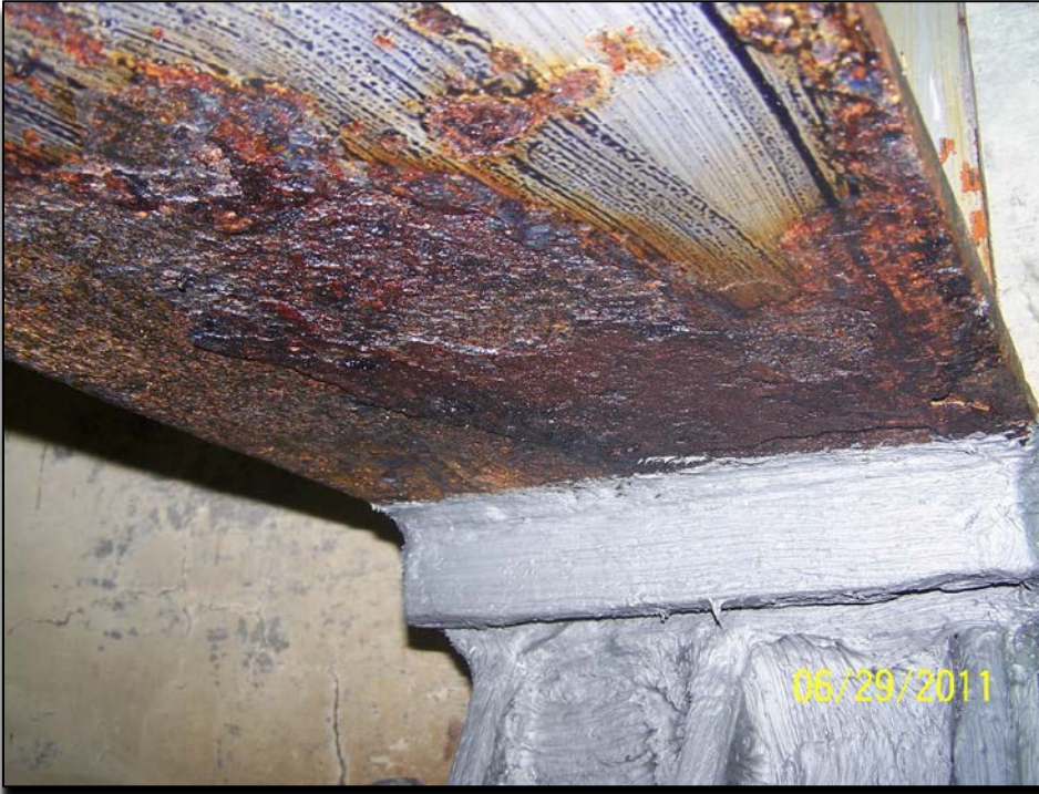
Figure 16. Conversion Coating Applied over Stratified Rust.
