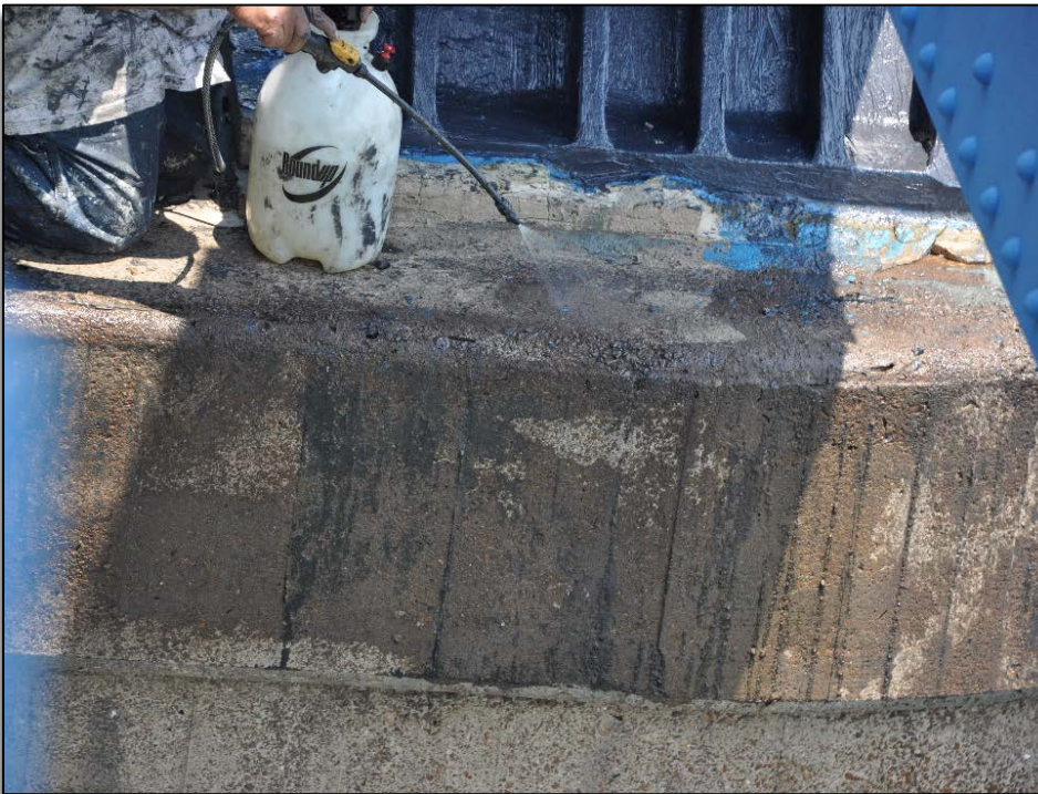
Figure 17. Sealer Application on Bridge Pier with Lack of Coverage.
