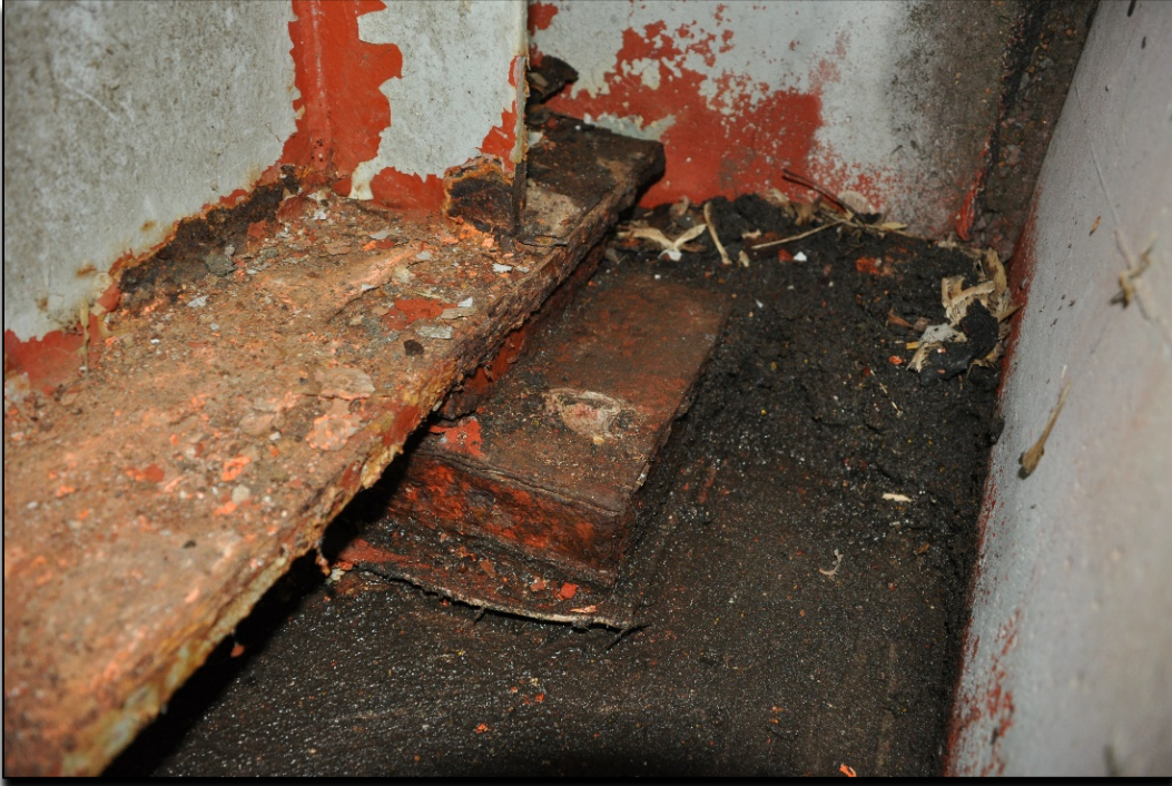
Figure 6. Debris Removal at an Abutment Revealing Corrosion of Bearing and Beam End
