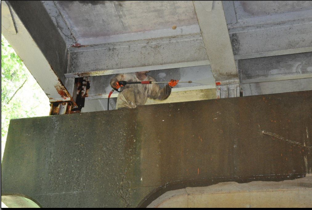
Figure 10. Washing a Superstructure and Substructure with Worker Standing on the Pier Cap. Note the Lack of a Safety Harness/Tie Off.
