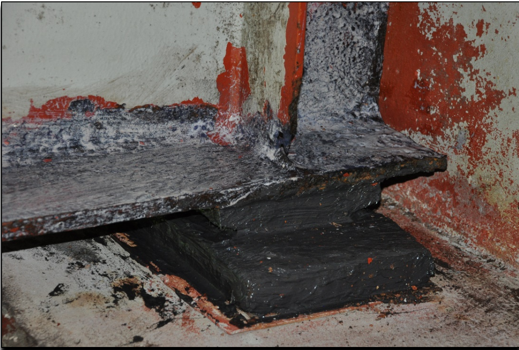
Figure 15. Conversion Coating Applied over Corroded Beam and Greased Bearing.
