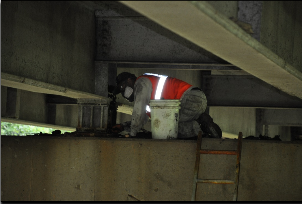
Figure 8. Worker Using a Hand Tool to Clean a Rocker Assembly. Note the Lack of a Safety Harness/Tie Off.
