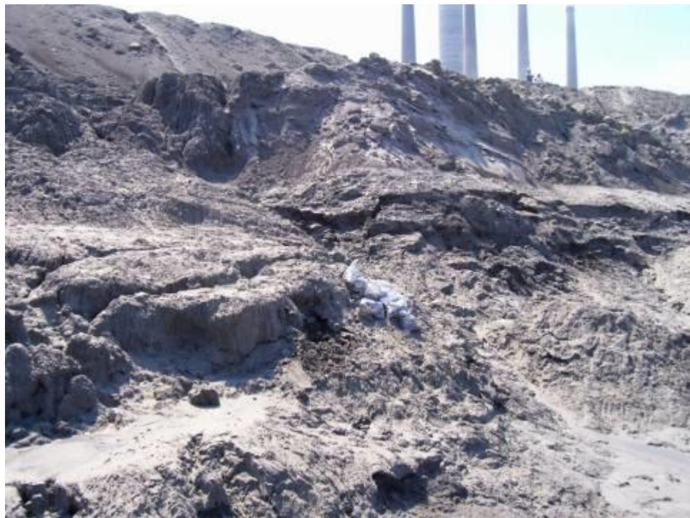
Figure 1.13: Slope failure occurred as a result of fly ash flow at the DPL Power Plant
