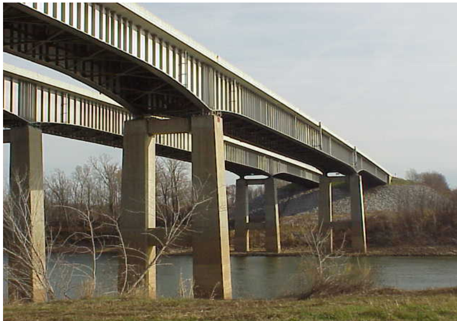
Fig. 11 Capacity of members and bearings of the main spans of the Cumberland River Bridges exceeds demand for projected 250-Year Seismic Event. [Consequently no retrofit is required]
