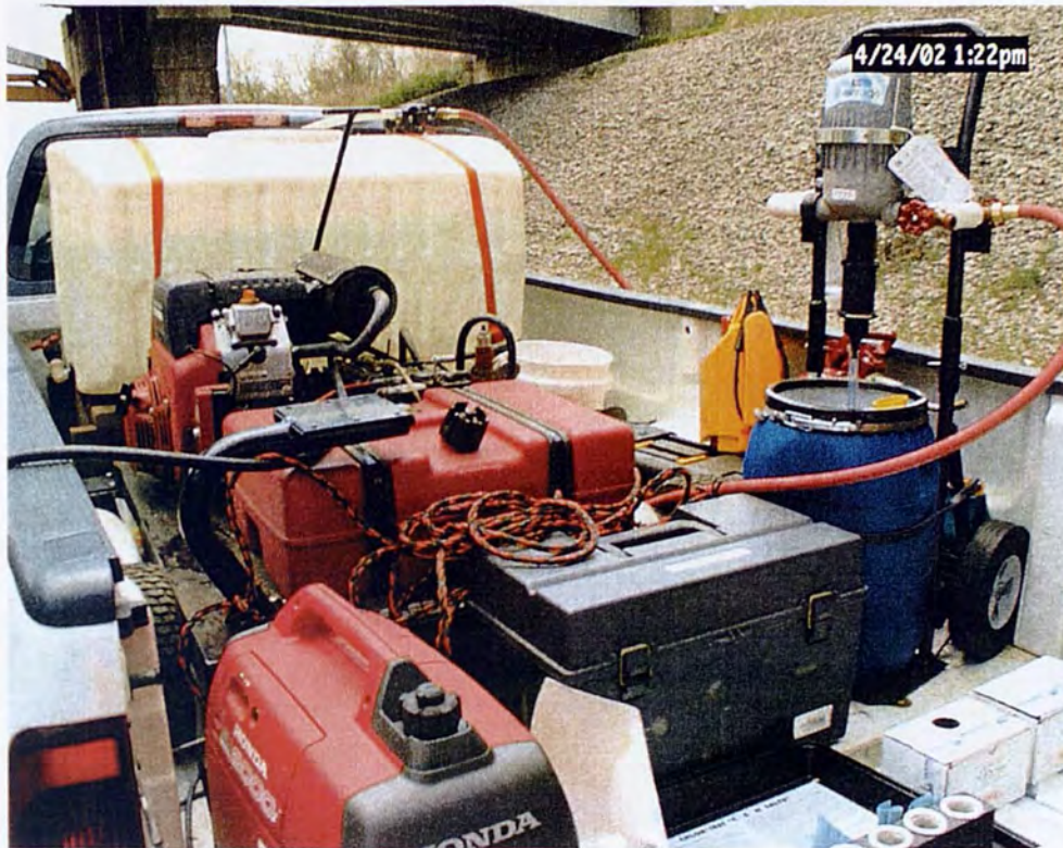
Figure 5 Equipment from CHLOR-RID that pumps the solution for removing invisible salts during pressure washing operation.
