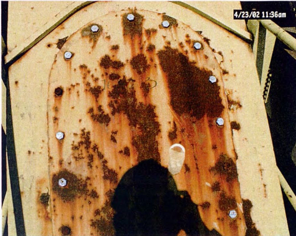
Figure 1 CHLOR*RID Test sleeve mounted on southbound arch flange (test area 3A).
