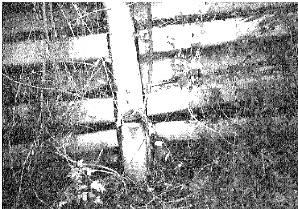
Figure 31: Failure in Vertical Member in Metal Bin Wall (Barbourville, KY)
