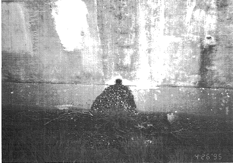
Figure 52: Migration of Backfill through Wall Drain (Knox County, 25E)
