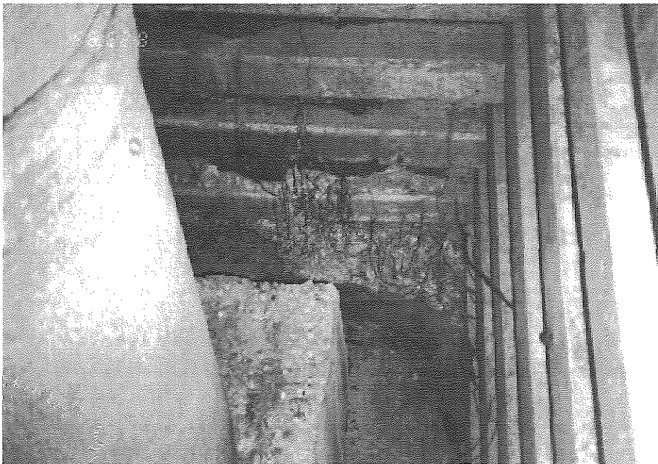
Figure 16: Wash out of Backfill Around Vertical Drain. (Kenton County, KY 8)
