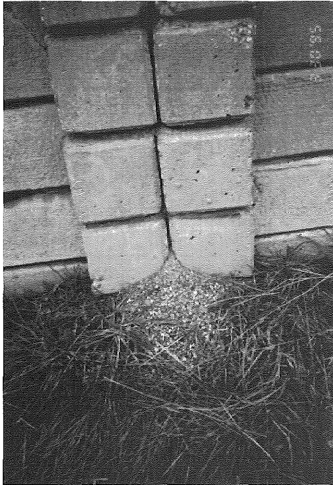
Figure 5: Migration of Backfill Through Vertical Joint in Crib Sections. (I-75 & I-71 Inter.)
