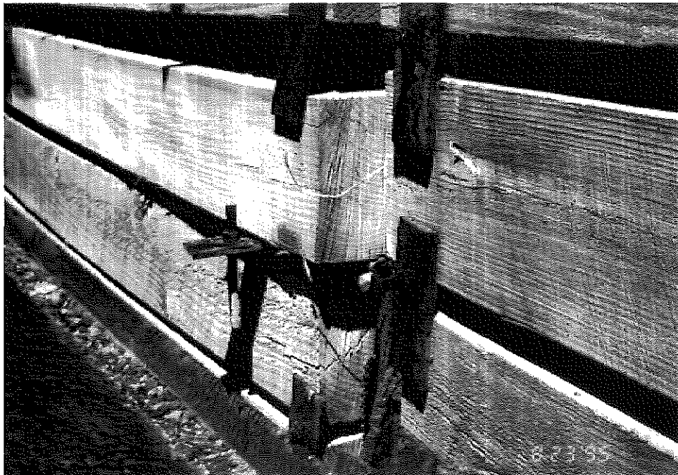
Figure 70: Broken Lagging Ties (Carroll County, KY 227)
