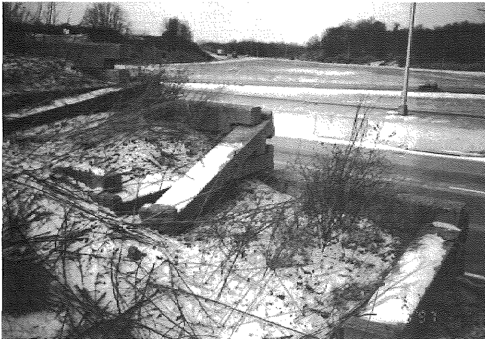
Figure 11: Sluffing of Unanchored Ends. (I-75 & I-75 Interchange)
