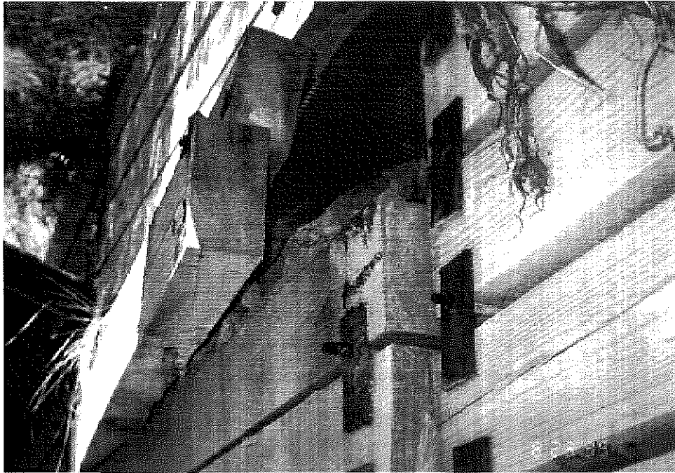
Figure 69: Displaced Timber Lagging Ties (Carroll County, KY 227)
