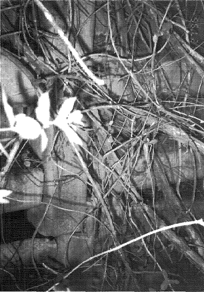
Figure 32: Failure in Vertical Member with some Lateral Displacement
