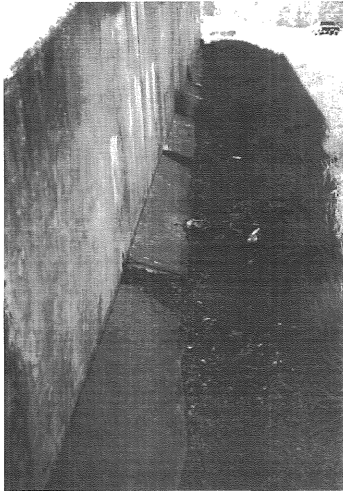
Figure 51: Migration of Backfill through Wall Drains (Knox County, 25E)
