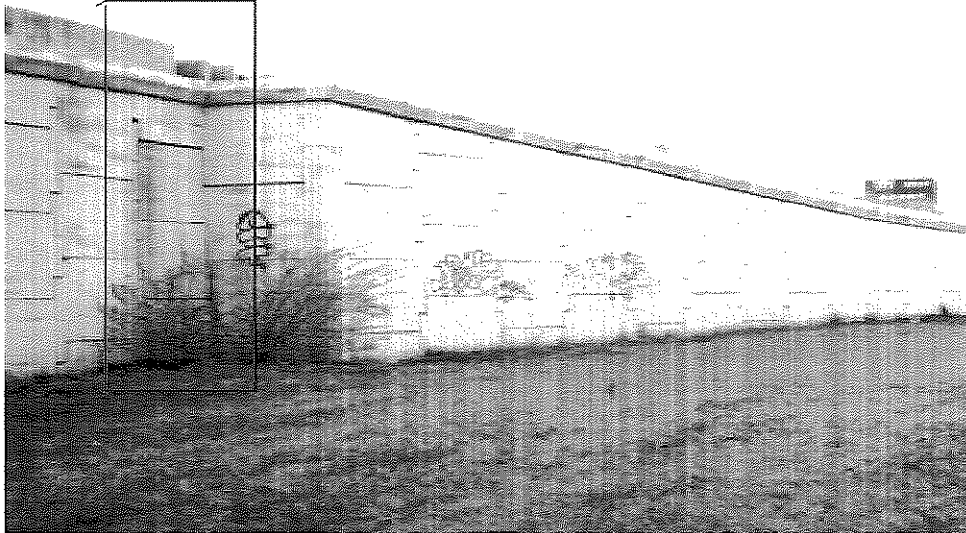
Figure 95a: Distressed Area on M.S.E. Wall (Kenton County, Wall # 3)
