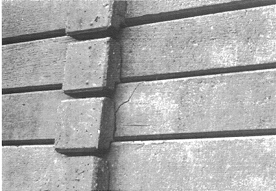
Figure 8: Cracking of Horizontal Crib Member at Connection. (I-75 & I-71 Interchange)
