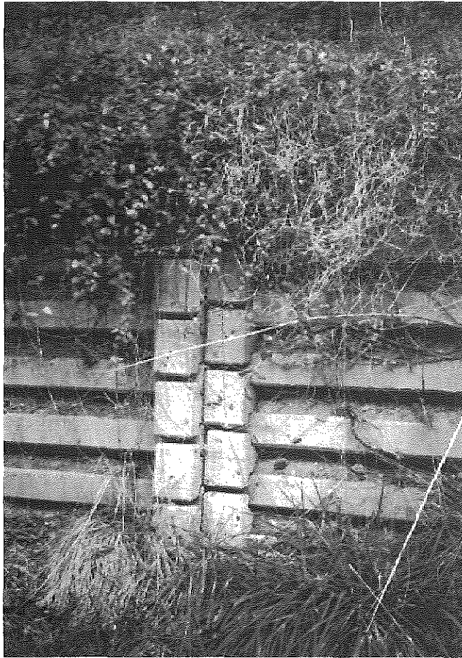
Figure 10: Possible Post Tilting of Crib Section. (Lee County, US 52)
