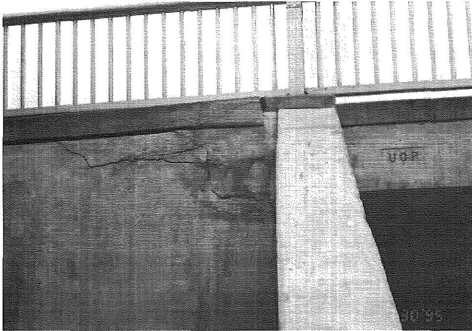
Figure 56: Moderate Cracking in Approach Fill Retaining Wall. (Kenton County, 2nd. Street)
