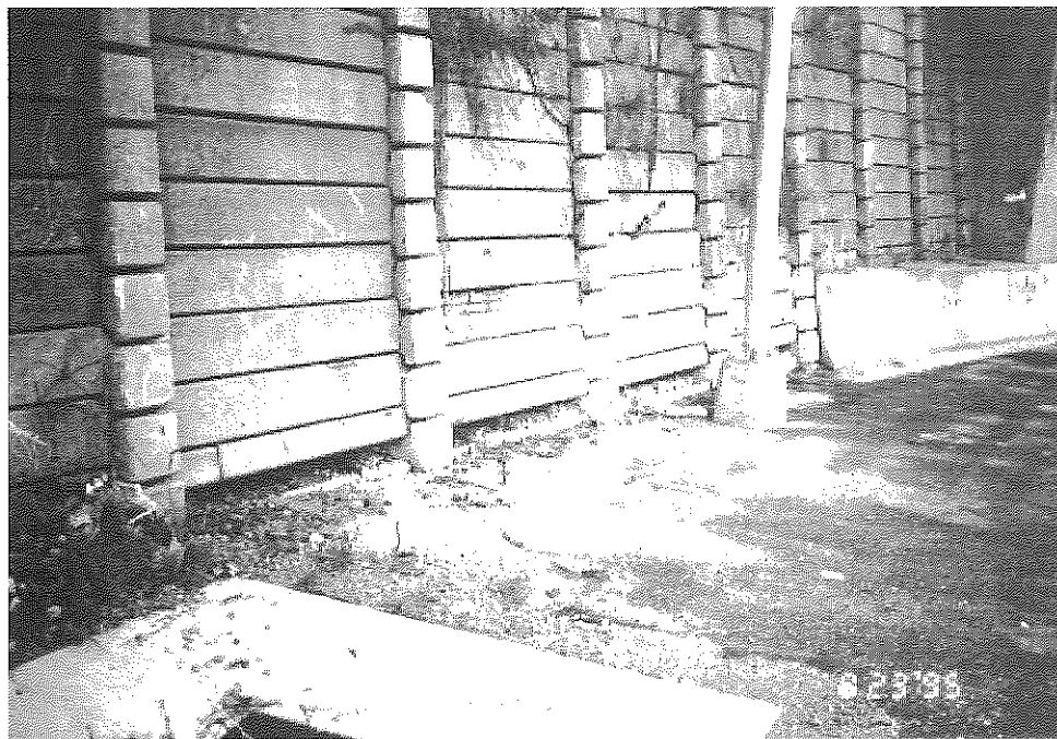
Figure 9: Spalling of Concrete on Face of Cribbing. (Kenton County, KY 8)
