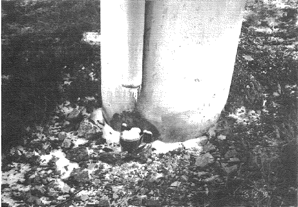
Figure 13: Separation in Outlet Pipe for I-71 Bridge Deck Drain. (I-75 & I-71 Interchange)
