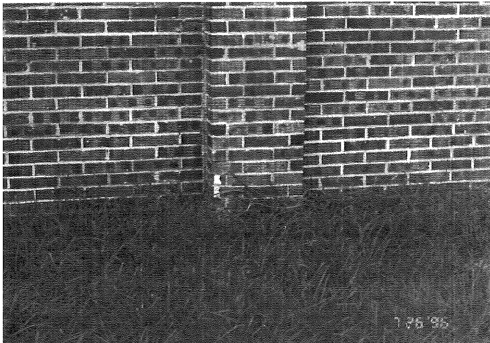
Figure 106: Chipped Bricks on Sound Wall Caused by Mower (Jefferson County, I-264)
