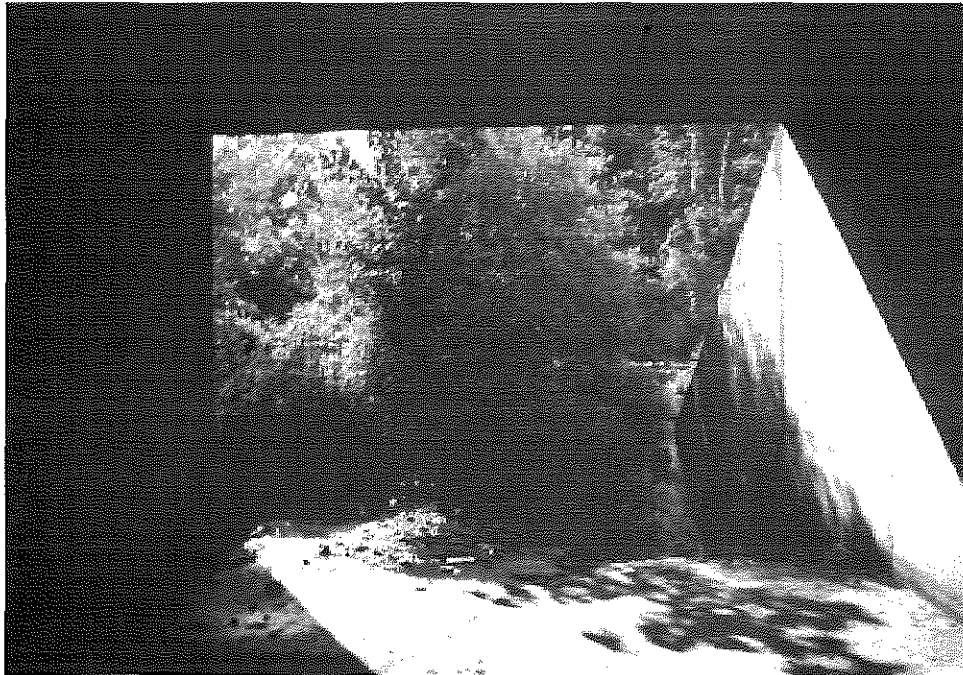
Figure 26: Vegetation in Culvert Outlet. (Lewis County, KY 9, Milepost 25)
