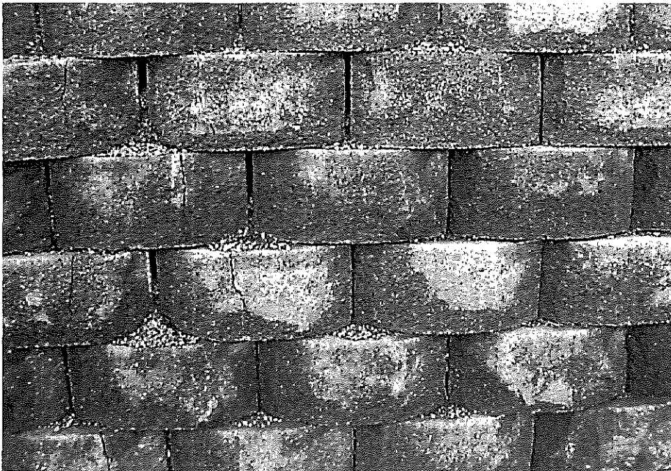
Figure 66: Migration of Backfill between Blocks
