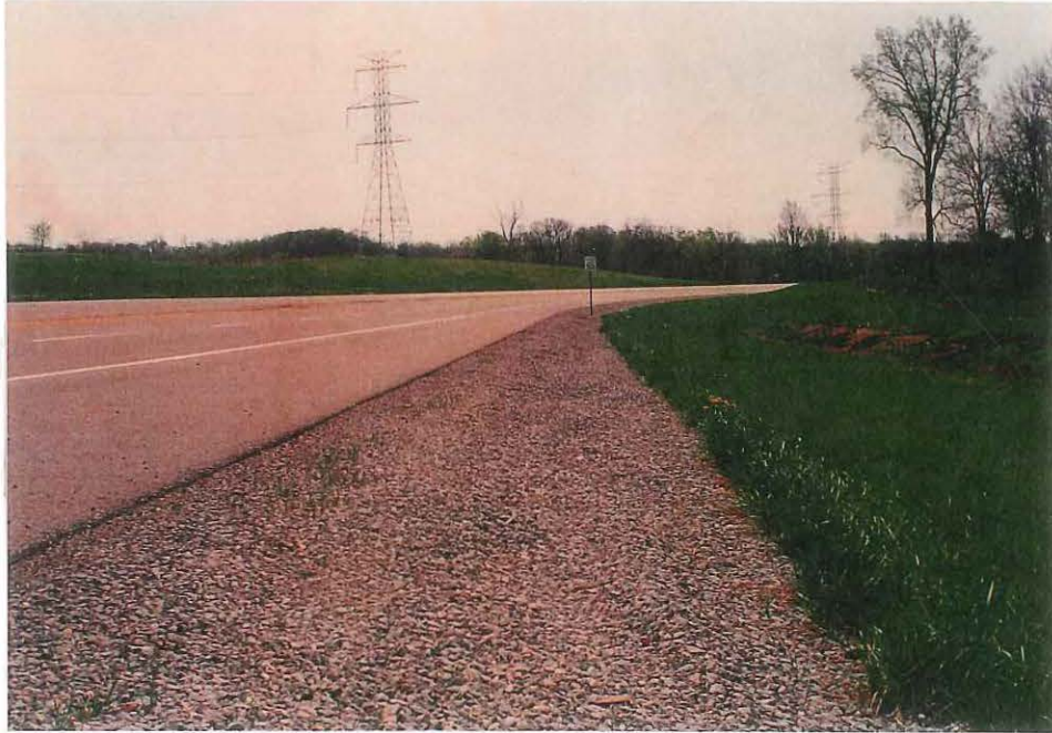
Figure 23. Daylighted, Untreated Drainage Blanket at AA Highway. Little Vegetation after Seven Years.
