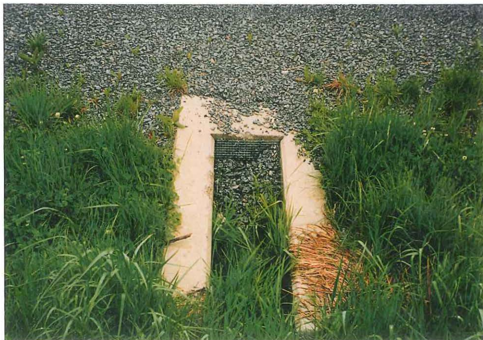
Figure 30. Drainage System Outlet Plugged with Debris and Vegetation.
