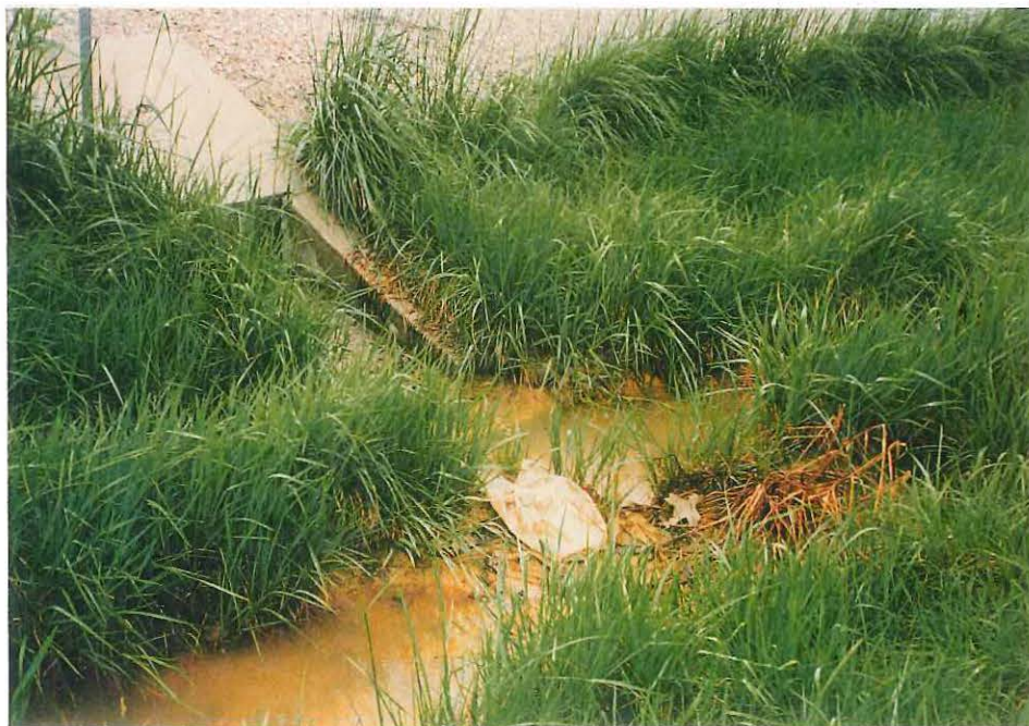
Figure 32. Drainage System Outlet Located Lower than the Ditch Line.
