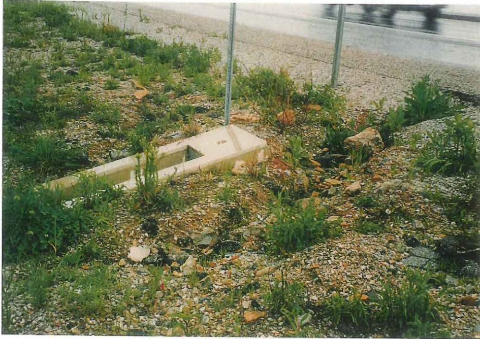
Figure 31. Drainage System Outlet Pipe Severed above the Headwall.
