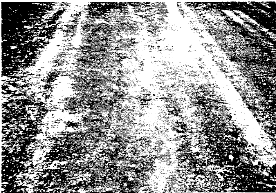
Figure 8. Longitudinal centerline cracking of the AFBC concrete base near STA 45+50 approximately two weeks after final compaction.
