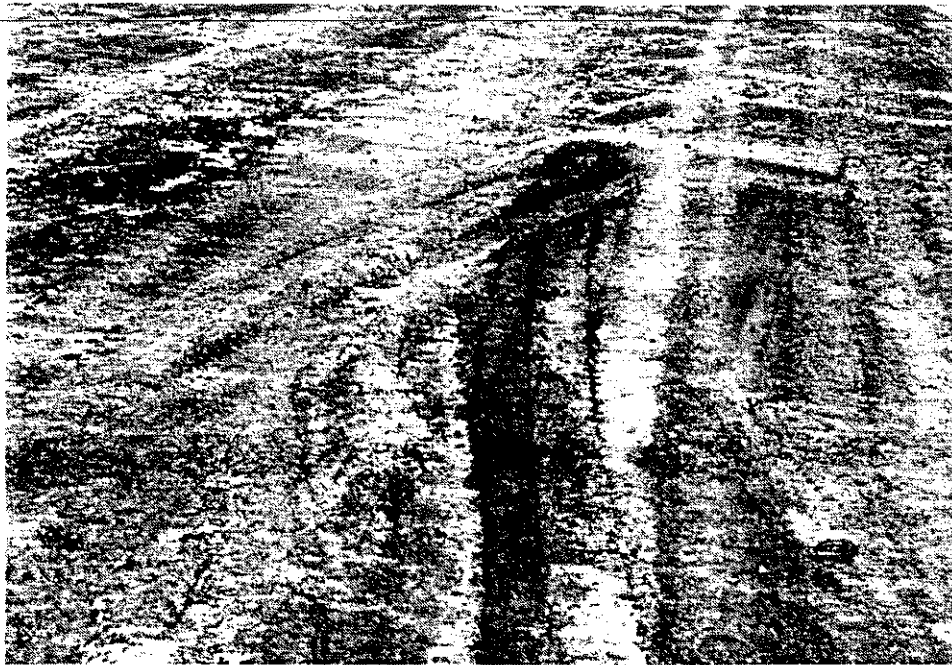
Figure 3. A view of the westbound lane of the experimental AFBC concrete base layer near STA 51+50 shortly after construction.
