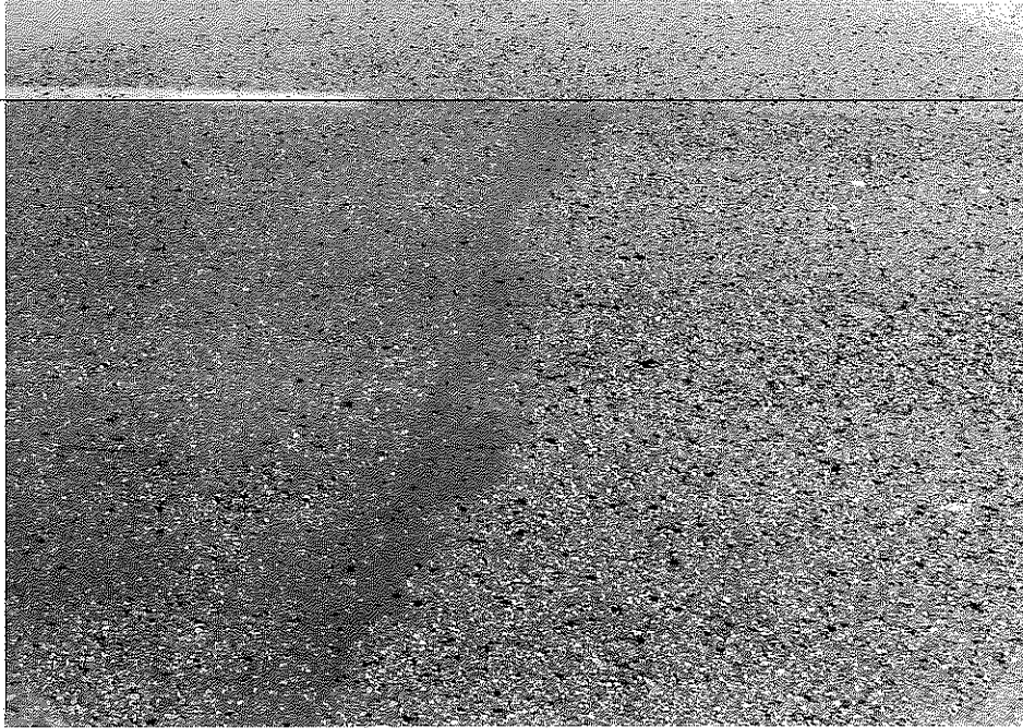
Figure D4. Surface Pitting and Excess Asphalt in the Southbound Lane of Survey Section No. 2.
