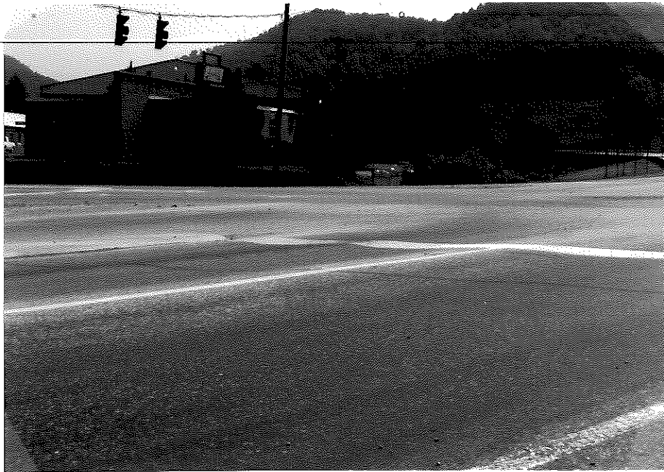
Figure B4. Rutting of the Asphaltic Concrete Pavement at the Junction of Whitesburg Bypass and US 119 (Section No. 1).
