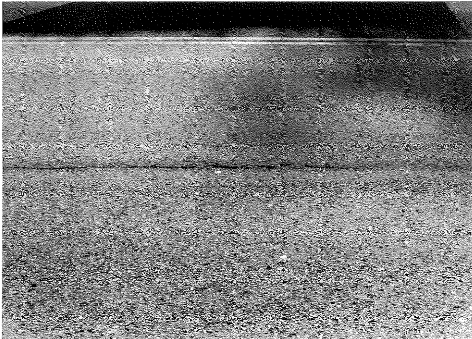
Figure D5. Longitudinal Crack in the Construction Joint between the Main Line and Truck Climbing Lane of Survey Section No. 4.
