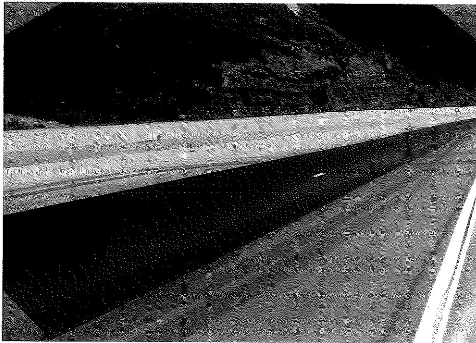
Figure A12. Maintenance Overlays Artificially Inflated Condition Ratings.
