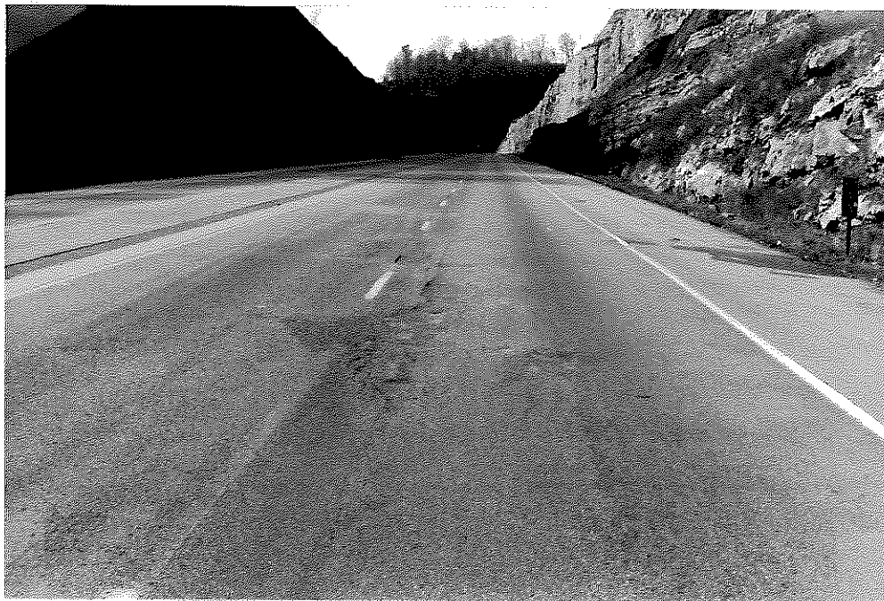
Figure A10. Water Seeping through the Shoulder Pavement near MP 15. Potholes, Longitudinal Cracking, and Surface Raveling are Dominant in both Lanes.
