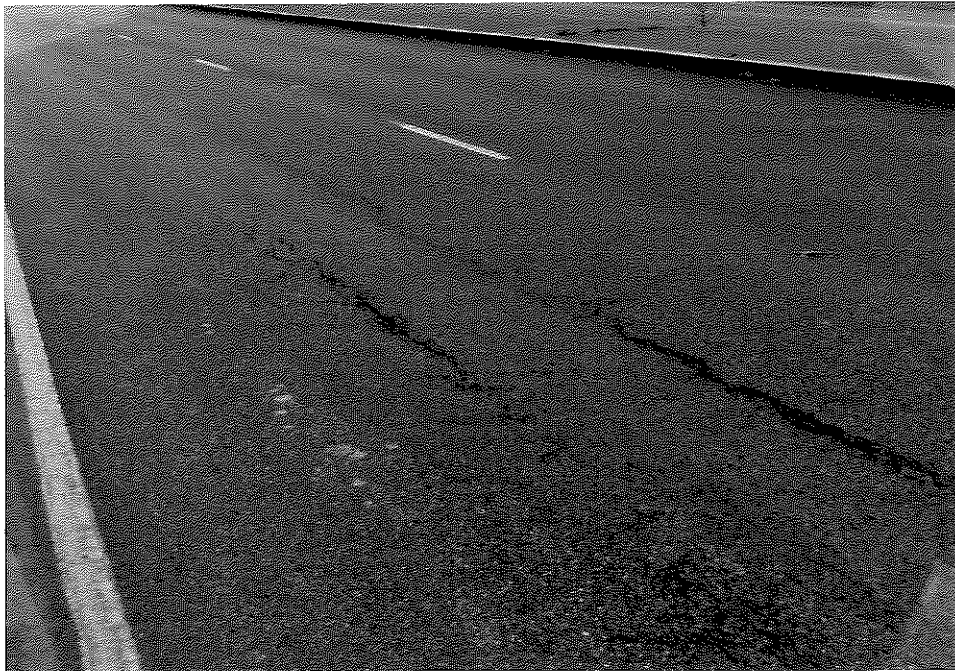
Figure B3. Longitudinal Cracking and Corrugations in the Asphaltic Concrete Pavement (Section No. 6).
