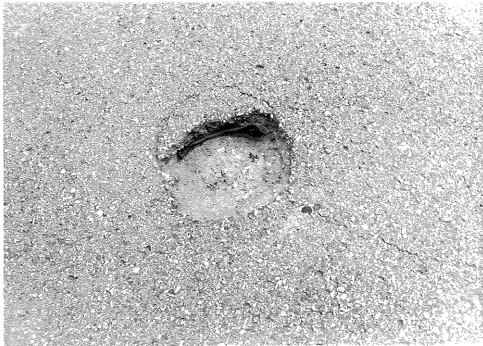
Figure E6. Pothole Formed in Southbound Lane as a Result of Paving over a Hat (Survey Section Number 7).
