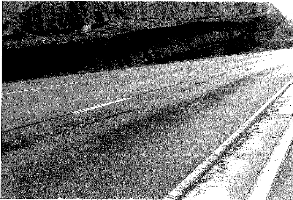
Figure A11. Westbound Shoulder Lane was Overlaid in the Fall of 1985. Median Lane Exhibits Excessive Stripping of the Bituminous Limestone Surface near Survey Station 558+75 in the Spring of 1986.
