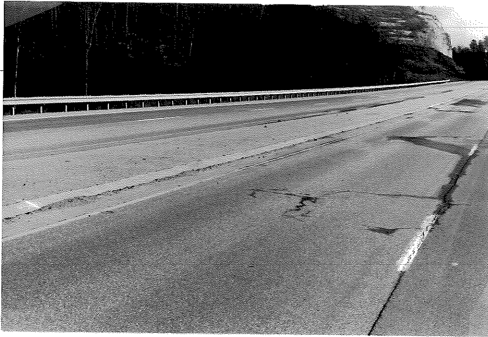
Figure A9. Water Emerging from Longitudinal Cracks in the Median Lane and from under the Lip Curb of the Raised Median near Survey Station 456+10.
