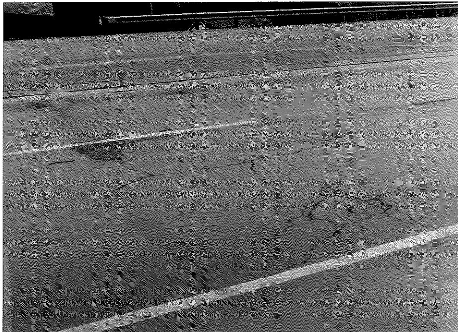
Figure C3. Longitudinal and Transverse Cracking, and Emerging Water near STA 7+00.
