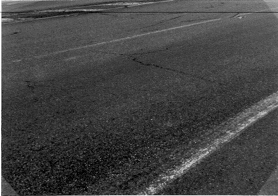
Figure B2. Transverse Cracking in the Asphaltic Concrete Surface (Section No. 8).
