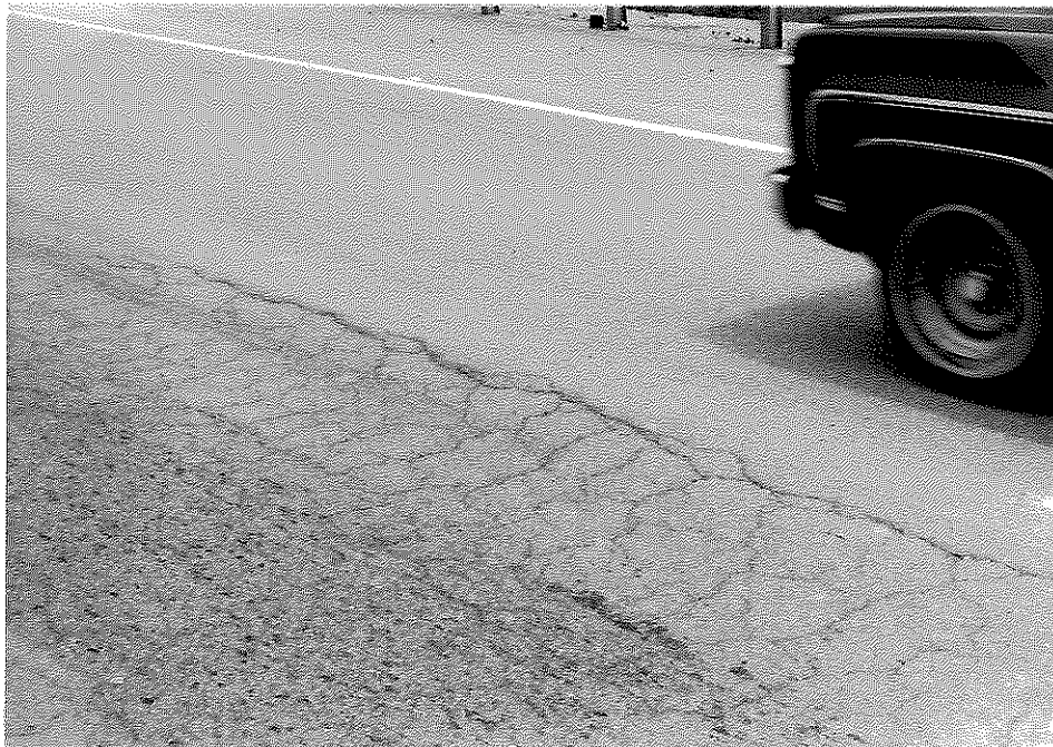
Figure G3. Northbound Median Lane of Survey Section No. 3 had Severe Shoving and Pushing.
