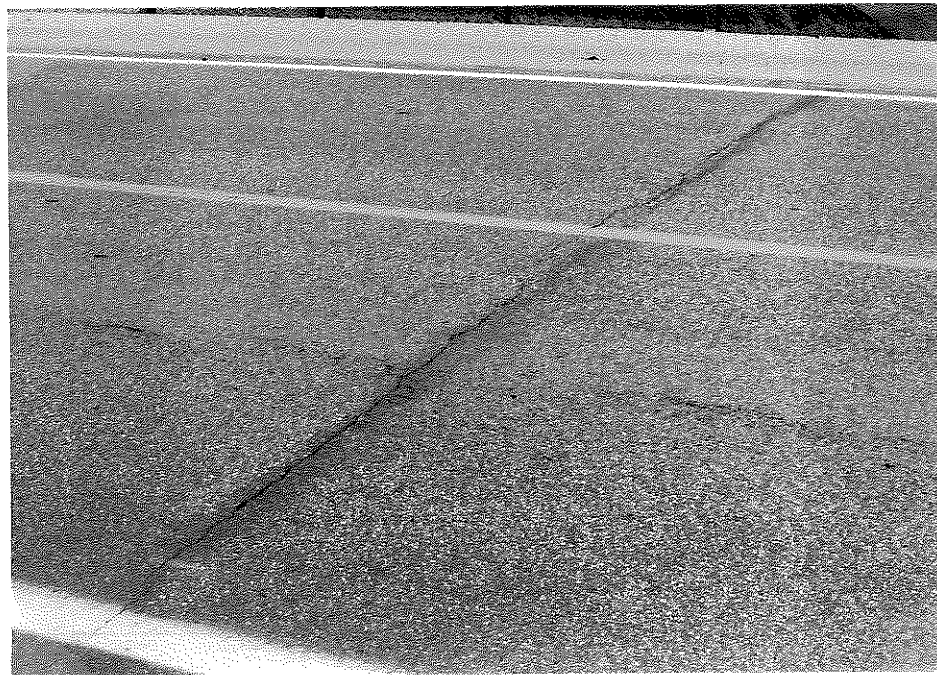
Figure E4. Slight Raveling of Transverse Crack above Construction Joint (Survey Section Number 6).
