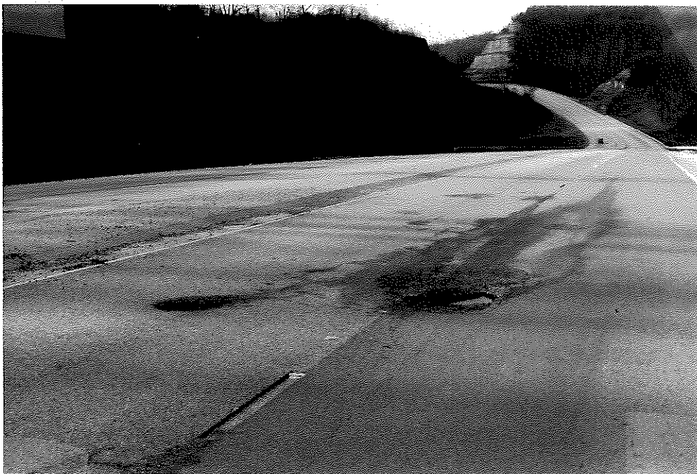
Figure A8. Severe Potholes, Emerging Water, and Longitudinal Cracking (looking Westbound in Survey Section Number 8).
