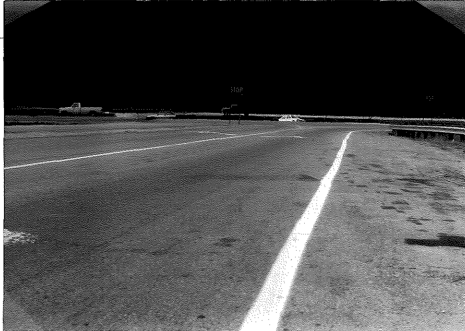
Figure F2. View of Northbound Shoulder Lane near Junction of KY 645 with US 23.
