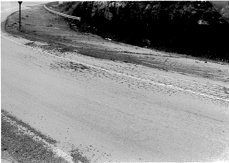
Figure G5. Southbound Shoulder Lane of Survey Section No. 1 showed Severe Alligator Cracking and Shoving and Pushing.
