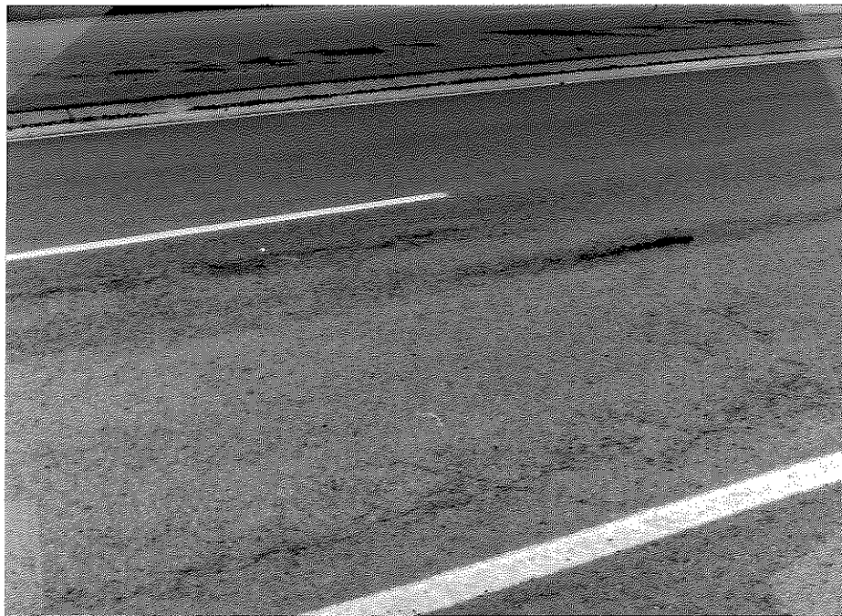
Figure C5. Raveling and Potholes in Pavement Surface near STA 138+25.
