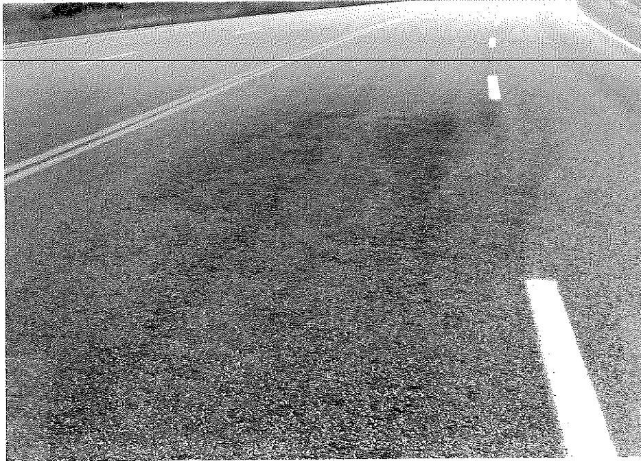
Figure E5. Raveling of the Bituminous Surface in the Northbound Lane of Survey Section Number 2.
