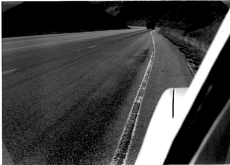
Figure D3. Raveling and Surface Pitting in the Southbound Truck Lane of Survey Section No. 2.
