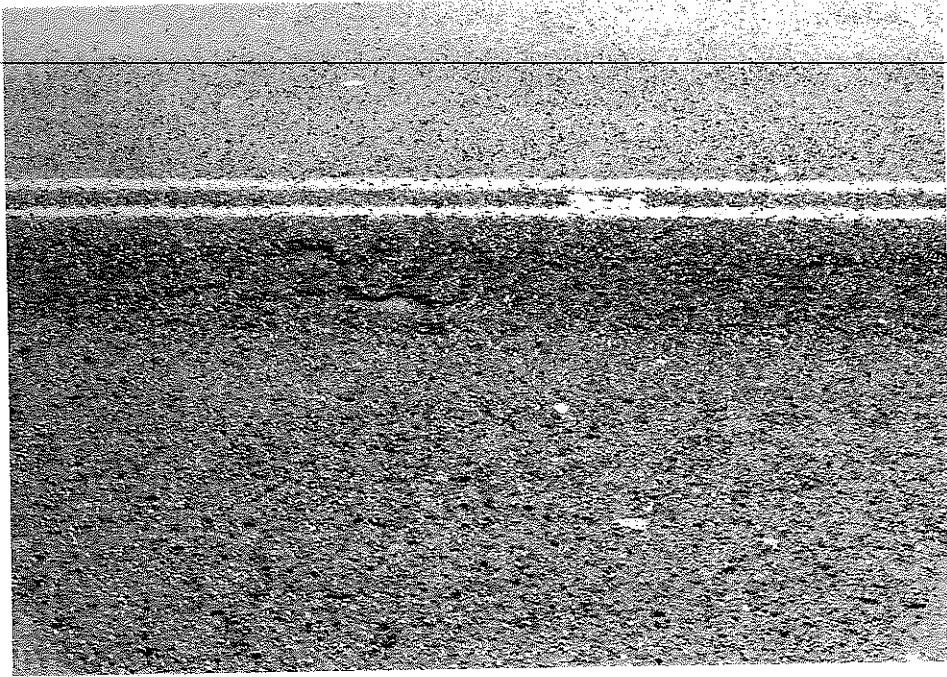
Figure D2. Severe Surface Pitting and Raveling in the Southbound Lane of Survey Section No. 2.
