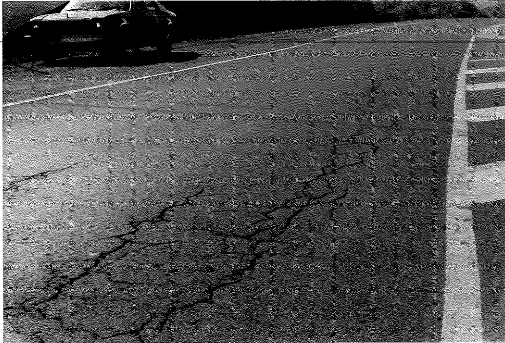
Figure C2. Pavement Cracking and Rutting near STA 1+00.
