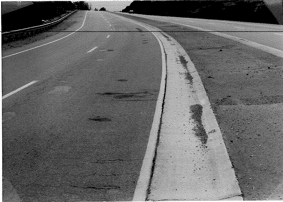
Figure G4. Northbound Median Lane of Survey Section No. 3 had Raveling and Patched Potholes.
