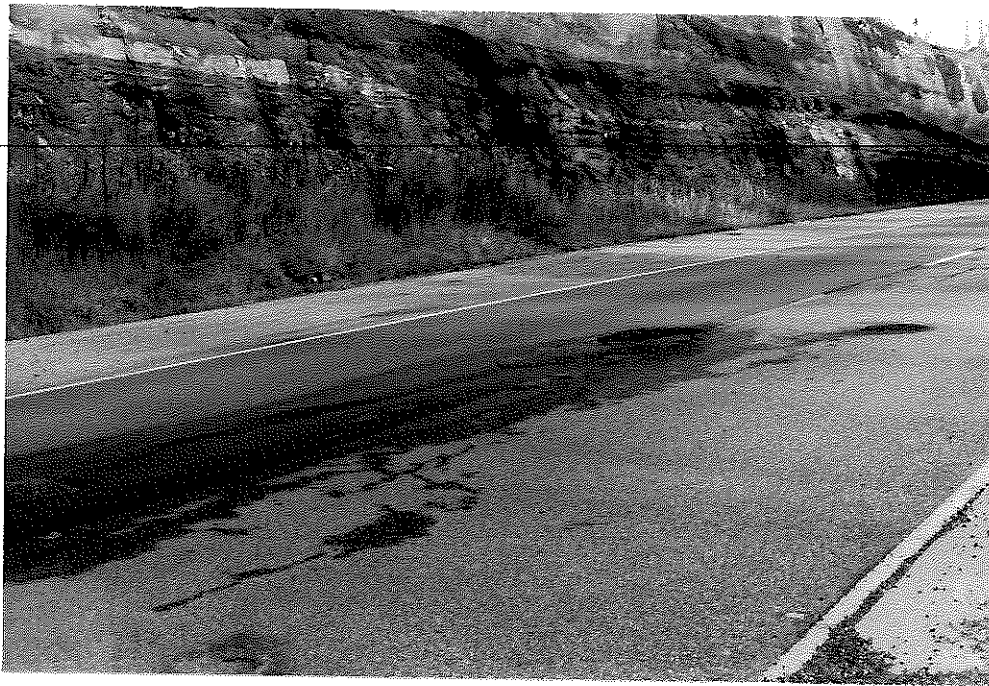
Figure A7. Severe Potholes and Emerging Water from Longitudinal Cracks in the Pavement in Survey Section Number 8.
