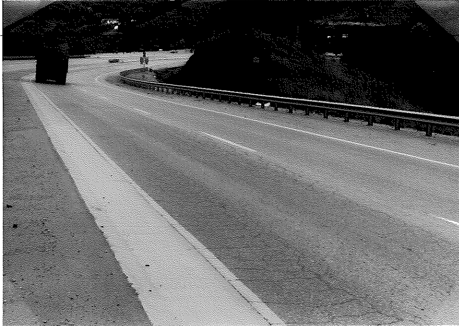
Figure G2. Northbound Median Lane of Survey Section No. 3 Exhibited Severe Rutting and Cracking.
