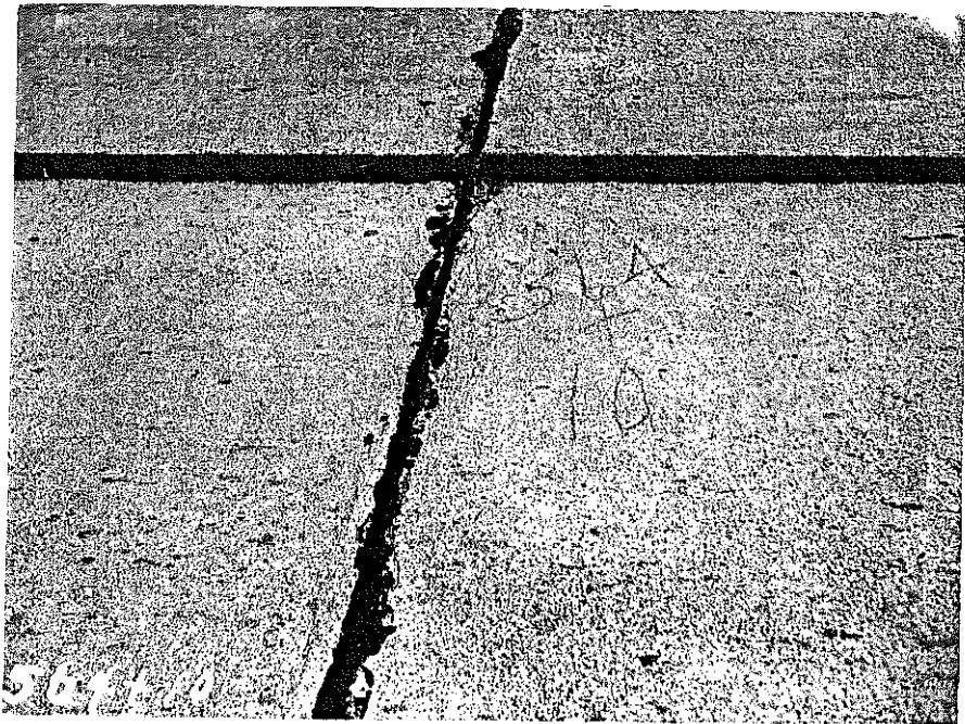
Fig. 5. Cracks formed parallel to a transverse joint at Sta. 564+10 on the Falmouth-Cynthiana Road. The coarse aggregate in this section of the road was glacial gravel, and the cement was normal portland. Only a few cracks parallel to joints were noted in 1947, but there was none in 1946.
