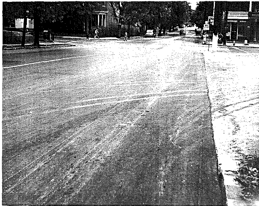
Fig. 6. Appearance of the finished pavement after about a month of use. This photograph was taken from approximately the same location as that in Fig. 1.
