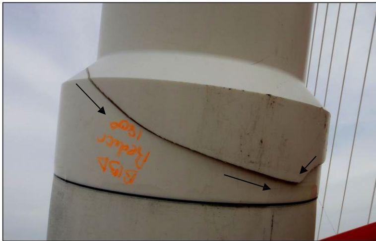
Figure 15: B13D : Reducer Crack at Notch Located at Diameter Transition
