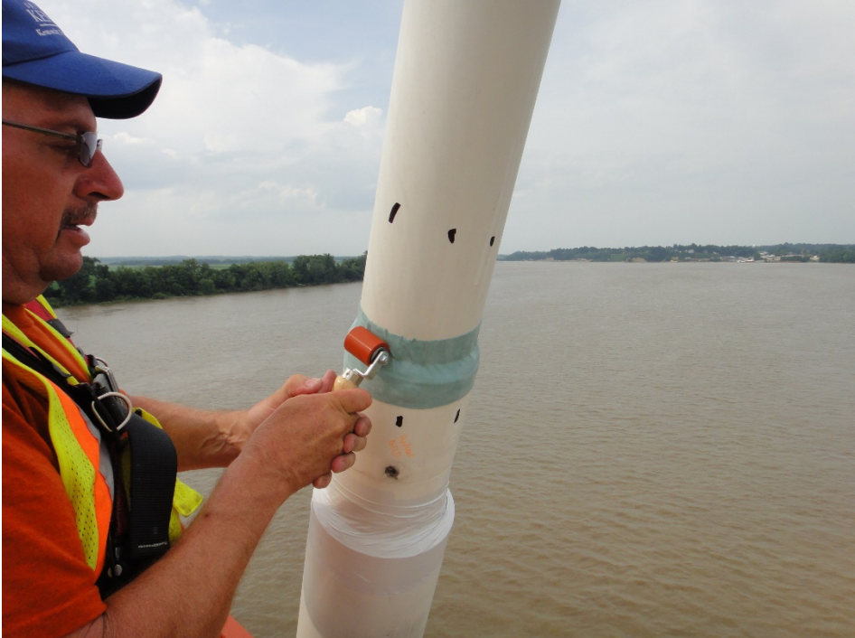
Figure 99. The Application of STOPAQ® Tape to Seal the Reducer-Stay Pipe Gap and Prevent Water Intrusion into the Grout Void.
