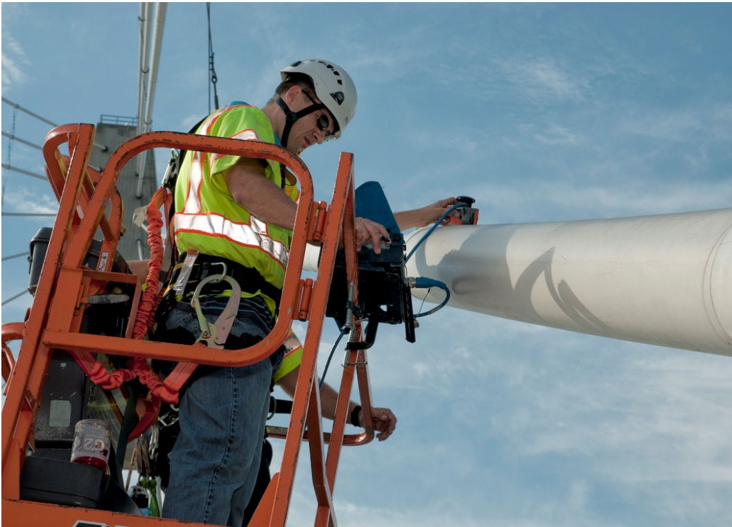
Figure 22. Detecting Grout Voids in Connection Sleeves by GPR using a GSSI Palm Antenna.
