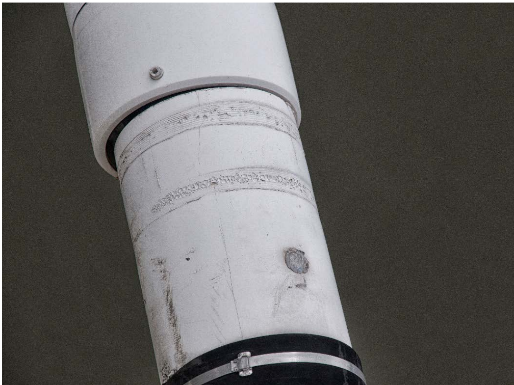
Condition Category 8: Failure of Electrofusion Weld between Connection Sleeve Coupler and Transition Pipe with Longitudinal Separation.
