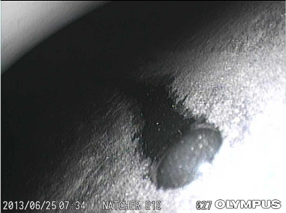
Figure 40. Picture inside a Grout Void Showing the Presence of Water in a Grout Void.
