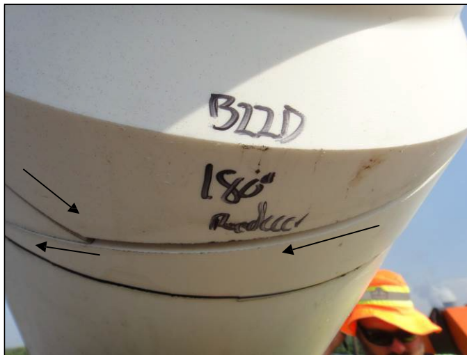
Figure 24: B22D : Reducer Crack at Notch Located at Diameter Transition
