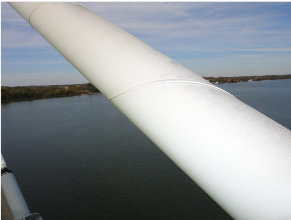
Figure 11. Helically Wound Ribbing on Stay Pipes.
