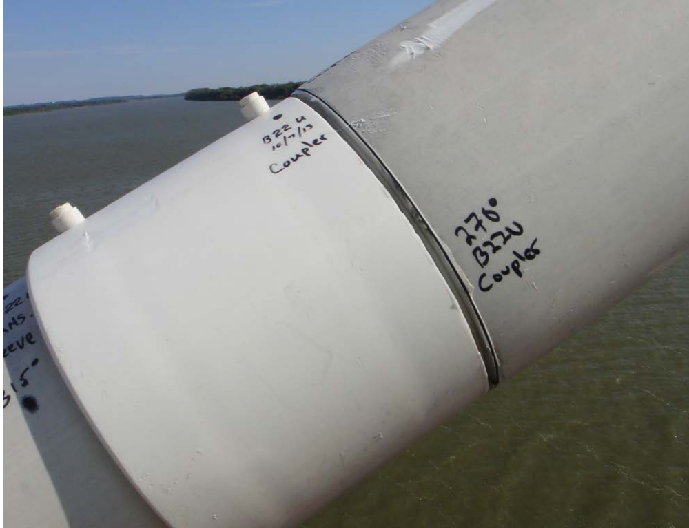
Condition Category 5: Crack in Coupler-to-Connection Sleeve Pipe Section Butt Weld.
