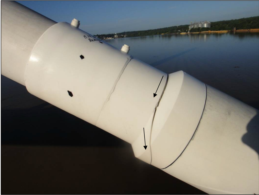
Figure 21: B19D: Reducer Crack at Notch Located at Diameter Transition
