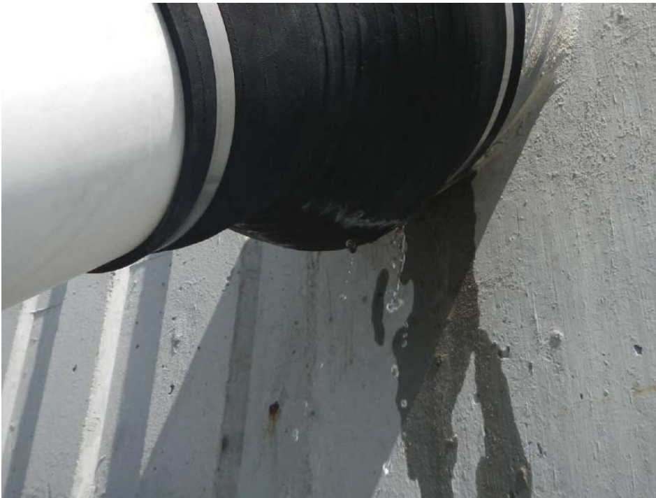
Figure 103. Water Leaking from Neoprene Boot at Tower Anchorage of Cable C7D (Ref. 11).
