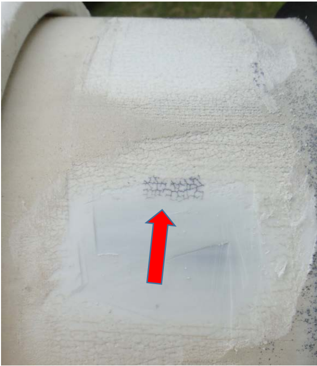
Figure 85. Scrape Location on Transition Pipe Showing Micro-cracking Penetration of White Coextruded HDPE Down to the Black Base Material.
