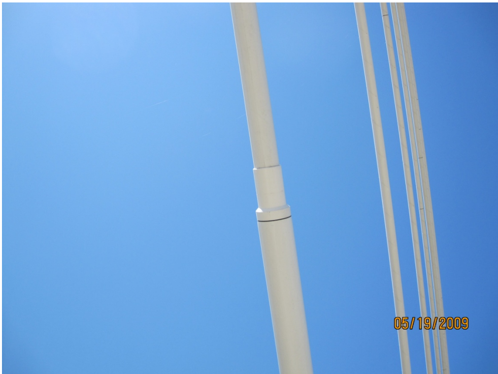
Condition Category 0:- No Cracking (Applies to Both Connection Sleeve Couplers and Reducers).
