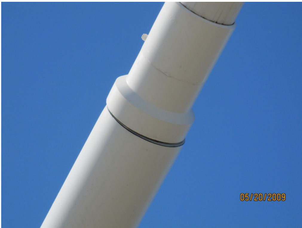
Condition Category 4: Crack in Reducer-to-Connection Sleeve Pipe Section Butt Weld with Lateral Displacement.
