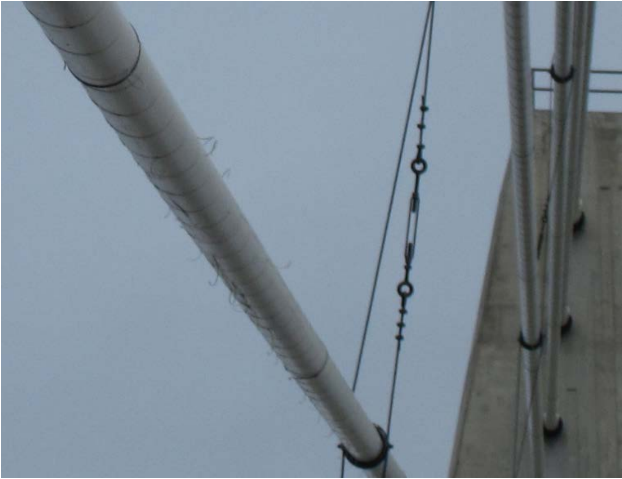
Figure 62. Severe Disbonding of Ribbing from Stay Pipe Segment (2009).
