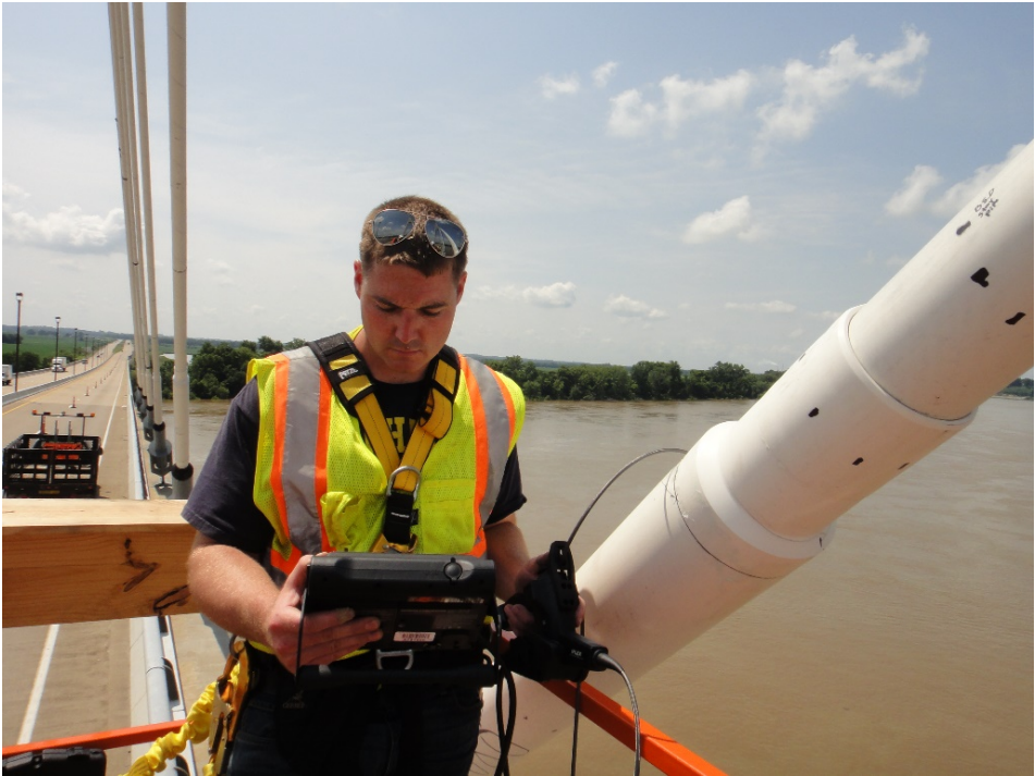
Figure 35. KTC Technician Operating the Articulating Camera of Videoscope inside a Grout Void in a Connection Sleeve.
