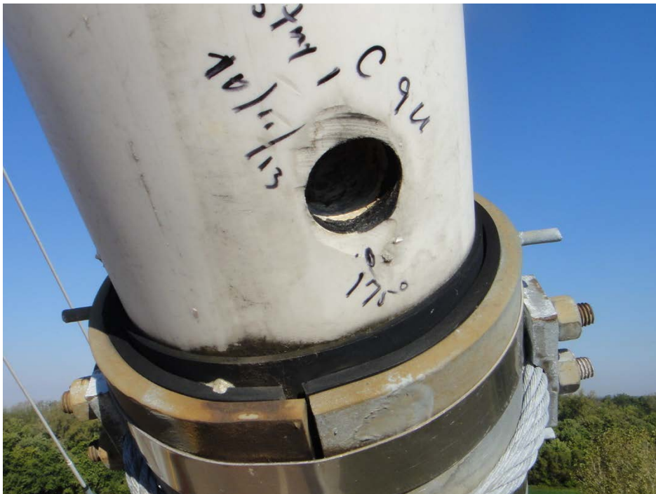
Figure 68. Missing Grout Plug.
