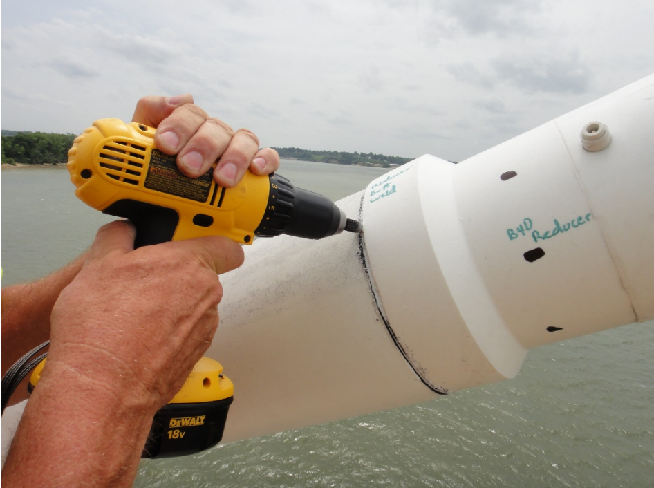
Figure 91. Drill with Rasp Bit Being Used to Create Bevel in a Butt-Weld Crack Prior to Plastic Welding.
