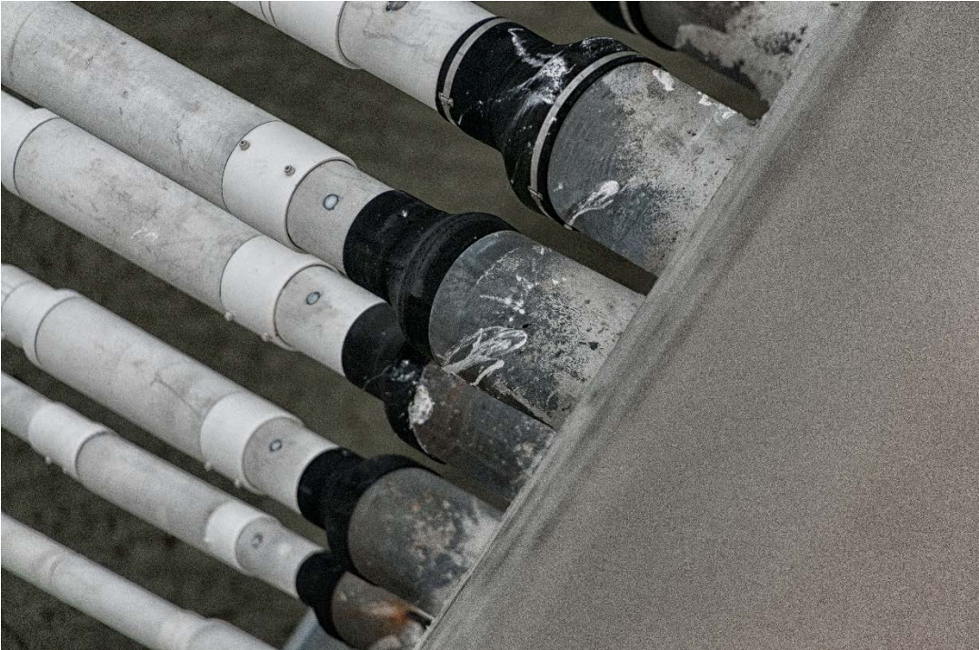
Figure 70. Neoprene Boots at the Upstream Side (Span 9) of Tower B Showing Missing Boot Retaining Bands.
