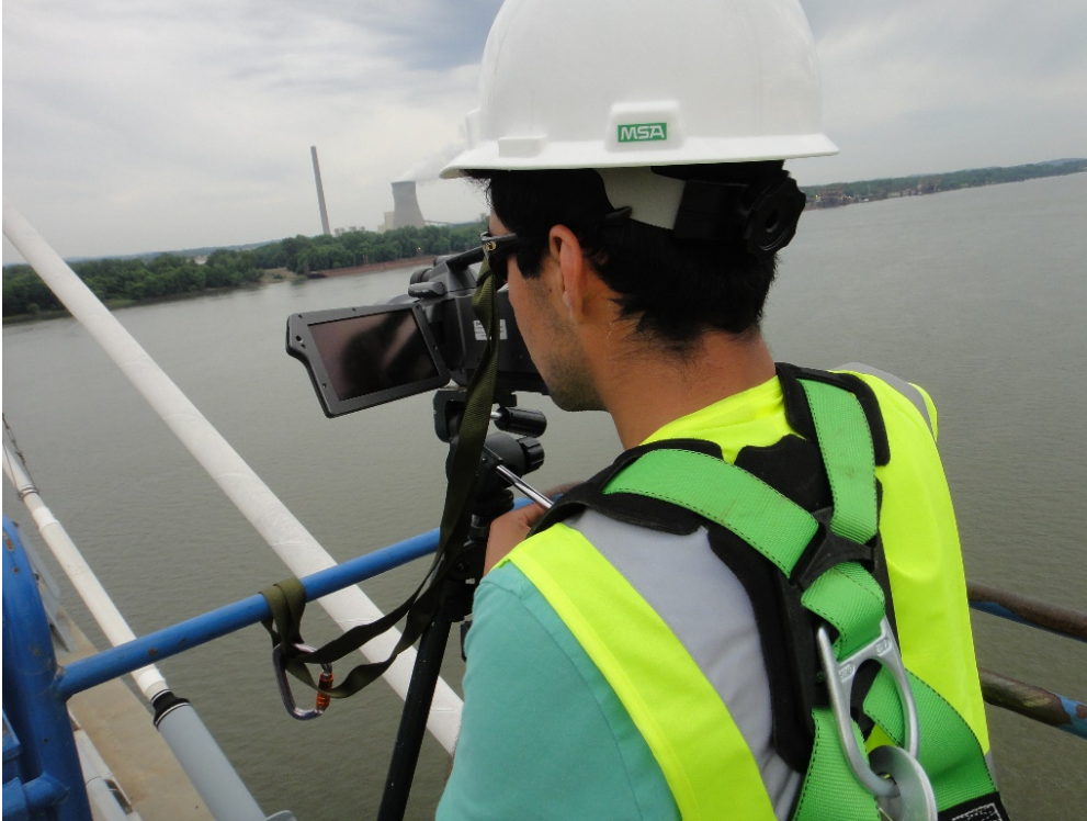
Figure 26. Camera Operator Taking Thermal Images of the Stay Cables from a Man Lift.
