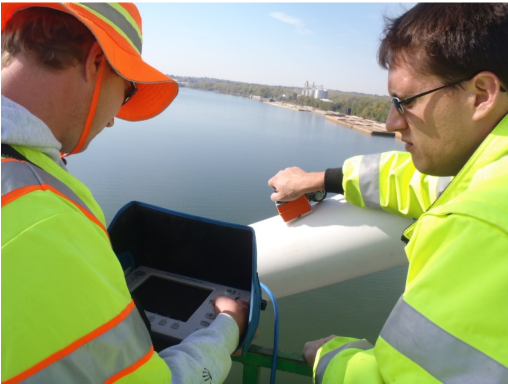
Figure 19. KTC Personnel Using GPR to Locate Voids in Deck Anchorage Piping (October 2010).
