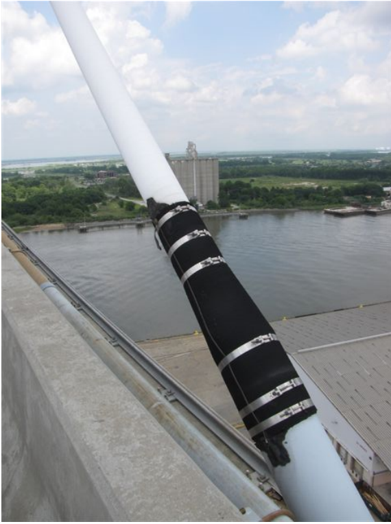
Figure 106. Zipper Sleeve on the US 17 Talmadge Memorial Bridge at Savannah, GA.
