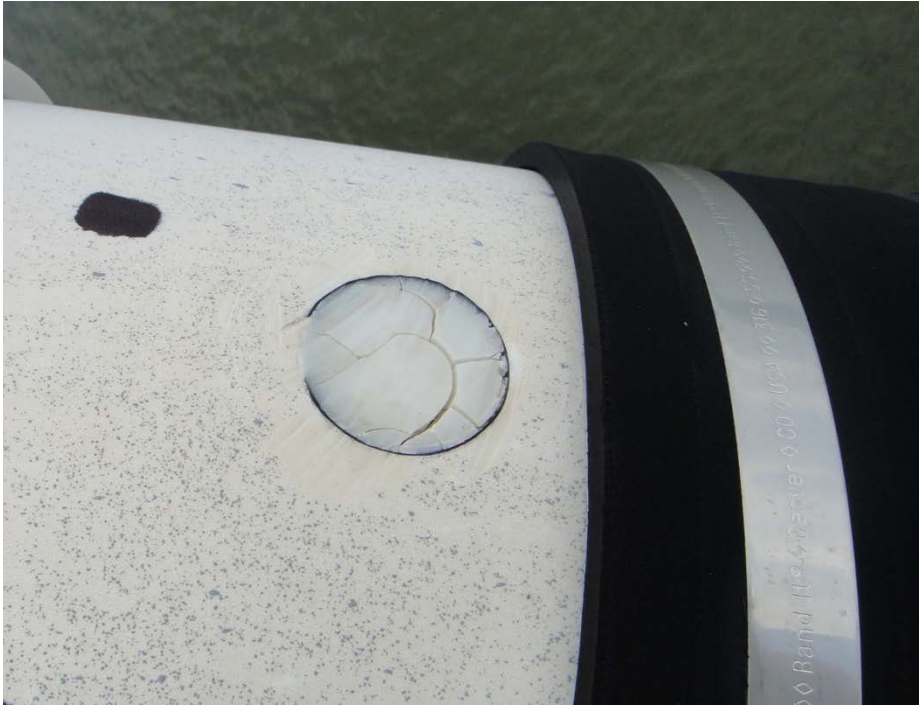
Figure 67. Grout Plug in Transition Pipe Having Extensive Cracking.
