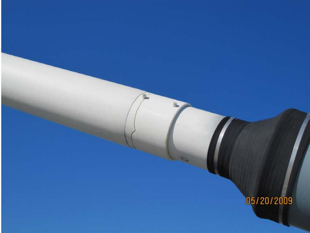
Condition Category 3: Crack Primarily in Small End of Reducer.
