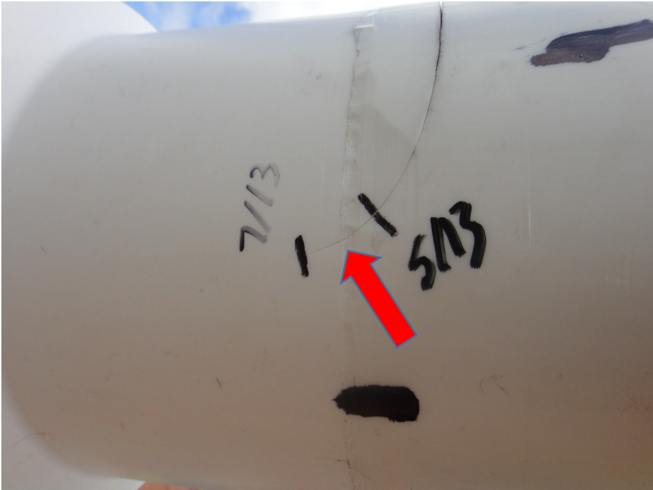
Figure 55. Crack Growth in Reducer Indicated by Marks (5/13 – Consultant and 7/13 – KTC).
