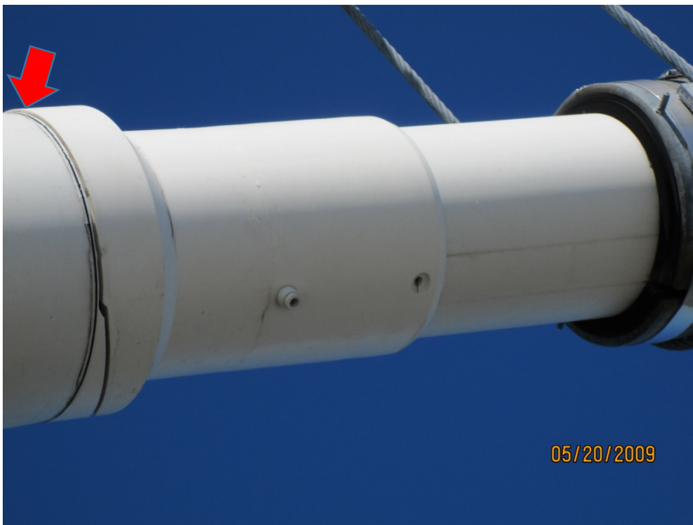
Condition Category 2: Crack Primarily in Reducer-to-Connection Sleeve Pipe Section Butt Weld.
