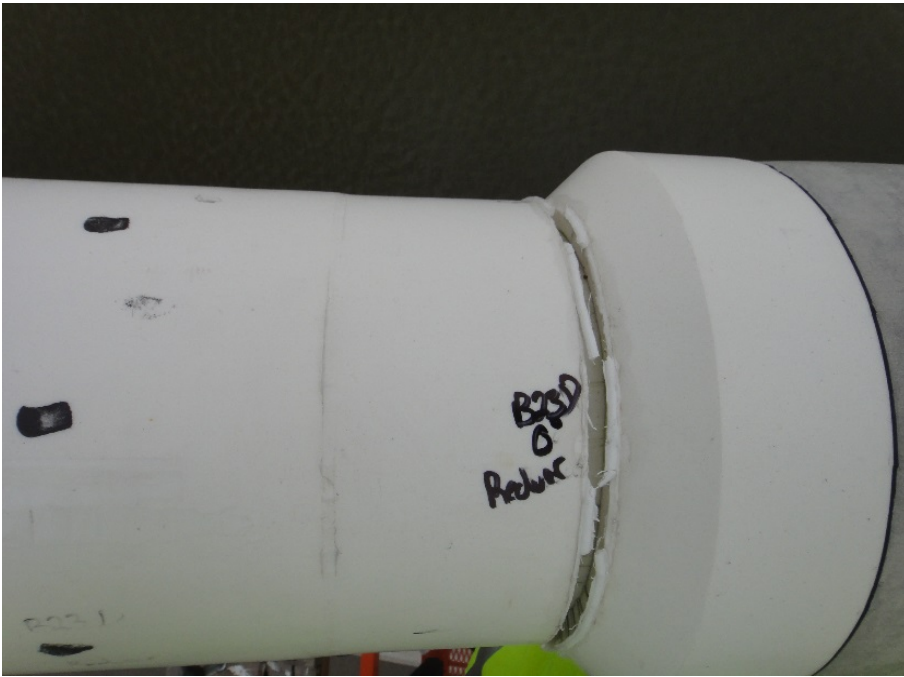
Figure 94. Failed Repair Weld (Ref. Figure 89) Discovered Several Months after Completion of Repair.
