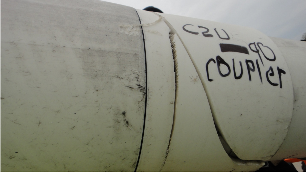
Figure 46. Complex Condition State 6 Cracking – A Single Crack at the Top of the Pipe Which Grew Radially in both the Clockwise and Counter-clockwise Direction to the Bottom of a Coupler (Looking Upward).
