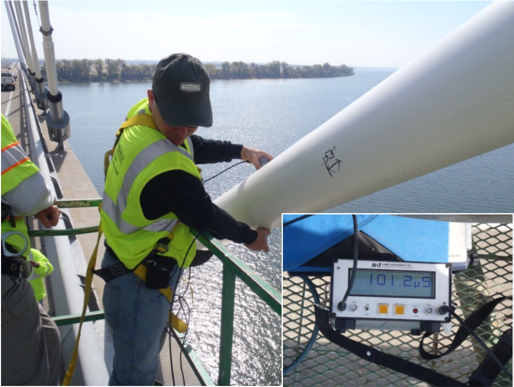
Figure 17. Locating Voids in Deck Anchorage Piping Using the Time-of-Flight Method (October 2010).
