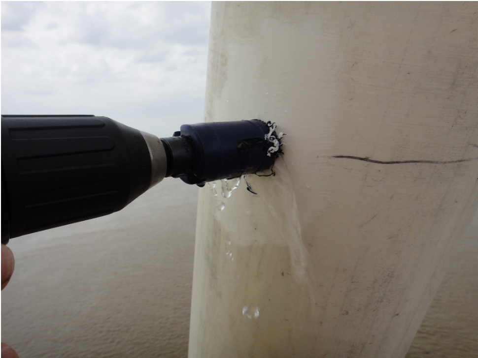
Figure 41. Water Leaking from a Grout Void in the Connection Sleeve Pipe at Stay Cable B12D.
