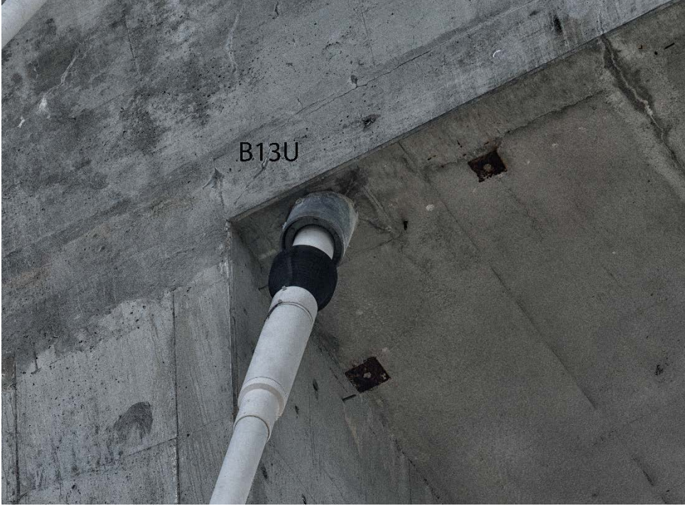
Figure 71. Detached Neoprene Boot at Tower Anchorage of Stay Cable B13U.
