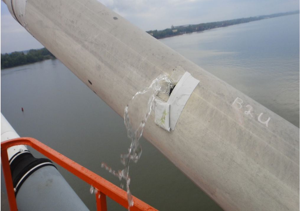
Figure 43. Water Gushing from Void in Cable B2U after Tape Covering Hole was Removed.
