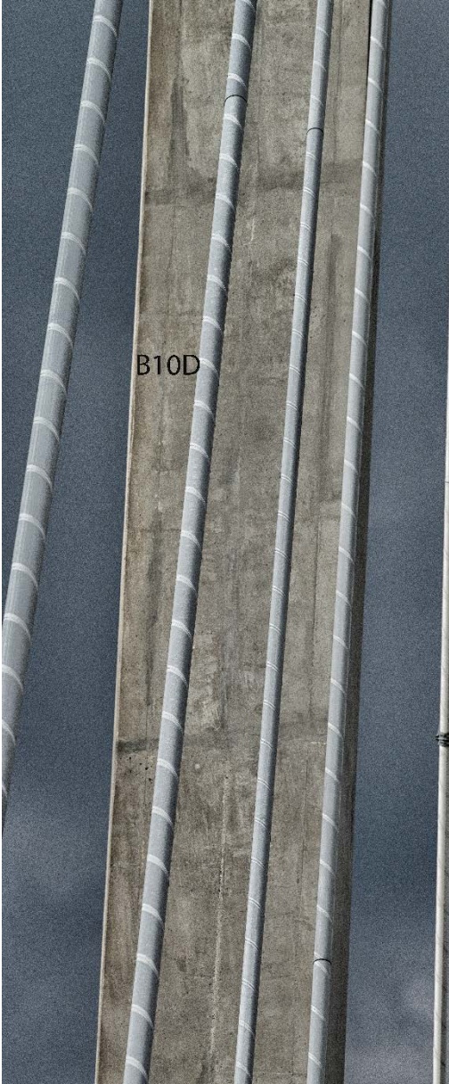
Figure 79. "Candy-Stripe" Appearance of Stay Pipes Due to Micro-cracking Variations at the Helically Wound Ribbing.
