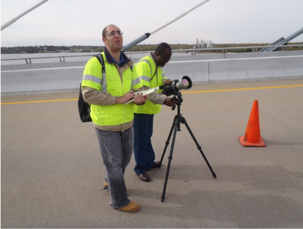
Figure 18. UK IR4TD Personnel Taking IR Pictures of the Deck Anchorage Piping (October 2010).
