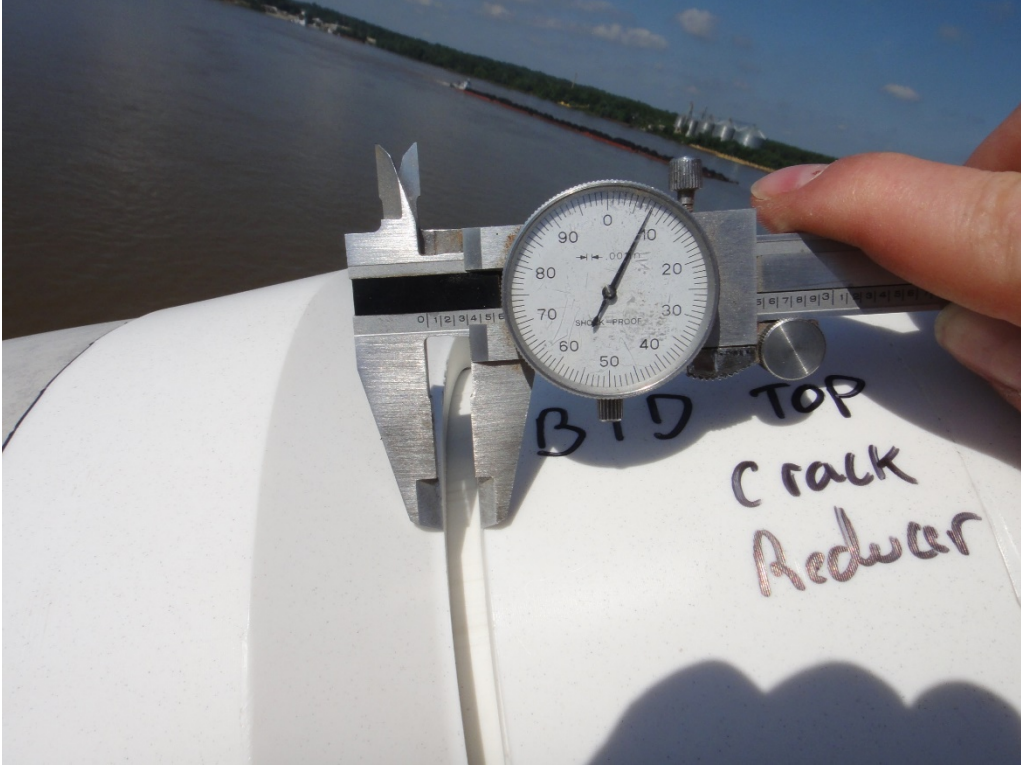
Figure 54. Large Crack Opening without Signs of Significant HDPE Deformation.
