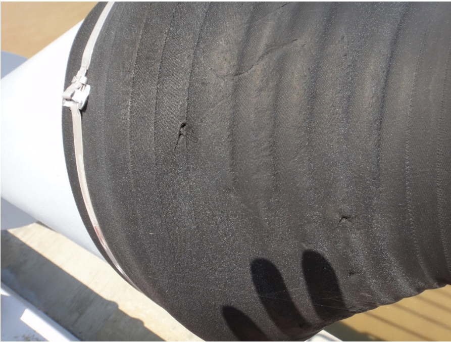
Figure 69. Neoprene Boot at Deck Anchorage with Superficial Damage.
