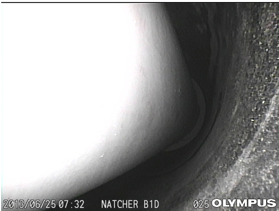
Figure 37. Picture Taken by Videoscope inside a Grout Void Looking Upward Where the Stay Pipe Passes Through the Reducer.
