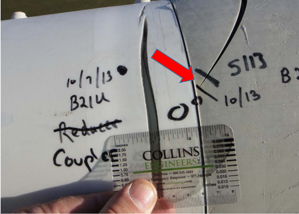
Figure 56. Crack Growth in Connection Sleeve Pipe Indicated by Marks (5/13 – Consultant and 10/13 – KTC).
