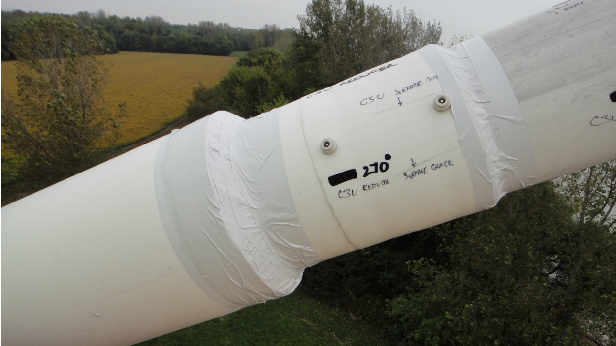
Figure 98. Tedlar Tape Applied over Crack in a Reducer and Reducer-Stay Pipe Gap.
