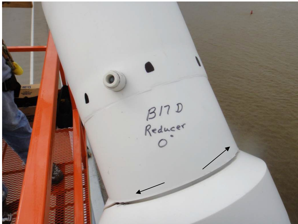
Figure 19: B17D: Reducer Crack at Notch Located at Diameter Transition
