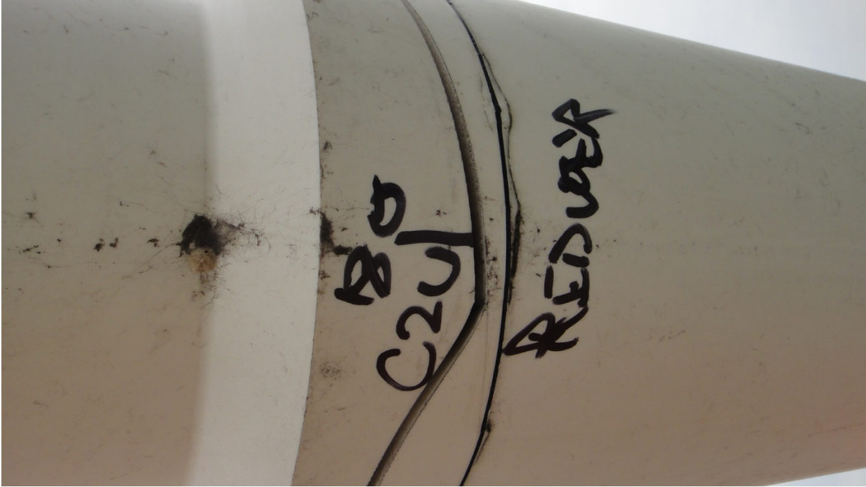
Figure 48. Bottom Side of HDPE Reducer Where Cracks Growing Clockwise and Counter-Clockwise from the Top Side Merge.
