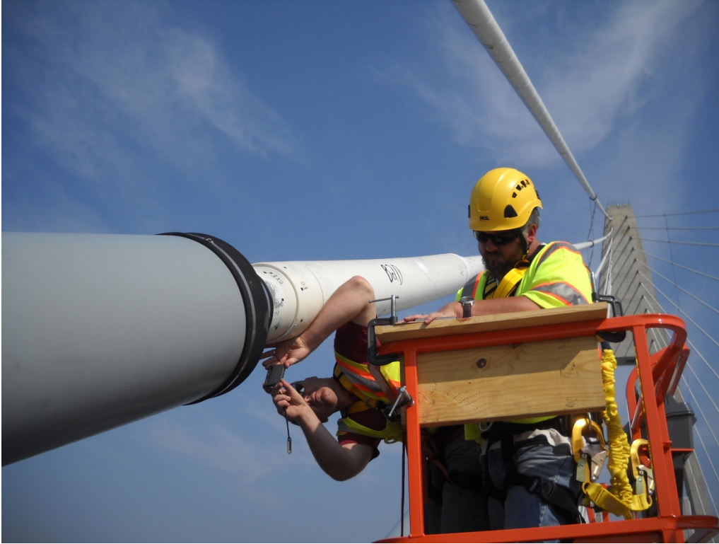
Figure 44. Arm's Length Crack Inspection of the HDPE Piping at the Deck Anchorages.
