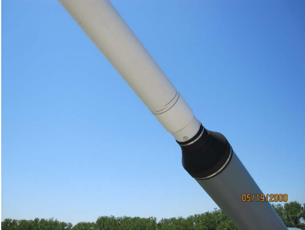
Condition Category 7: Crack in Connection Sleeve Pipe Section.
