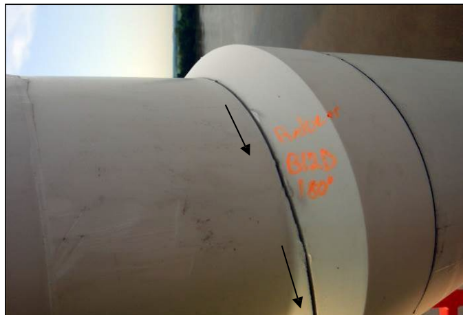
Figure 14: B12D : Reducer Crack at Notch Located at Diameter Transition
