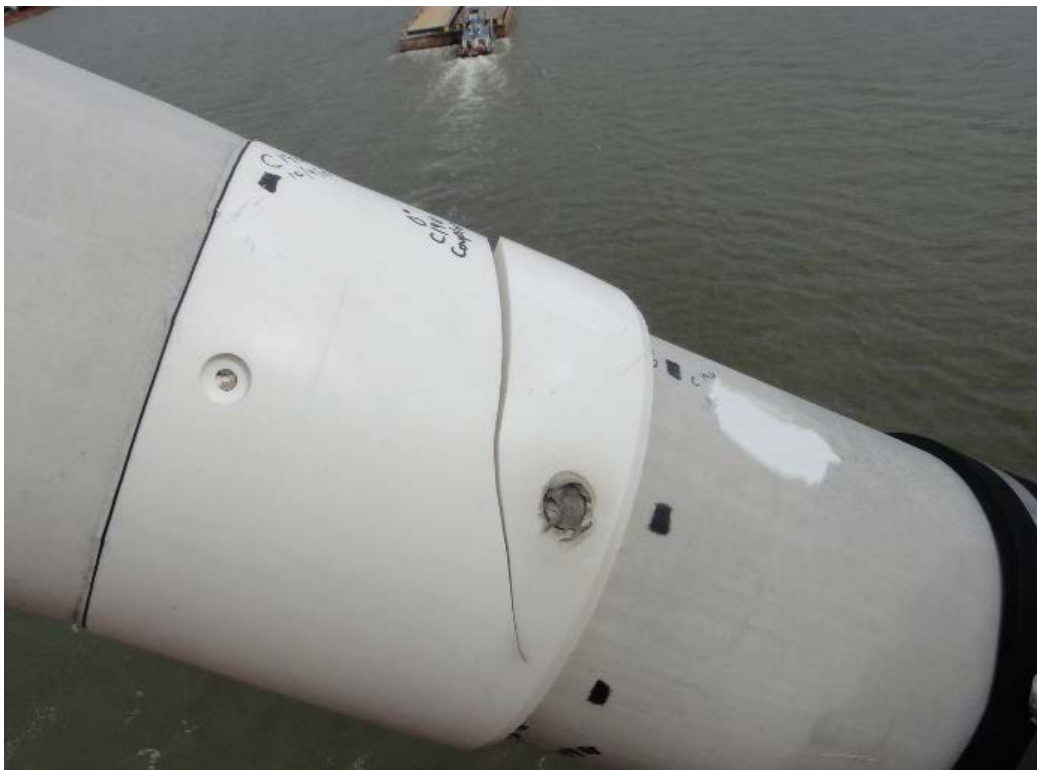
Condition Category 6: Crack in Coupler.
