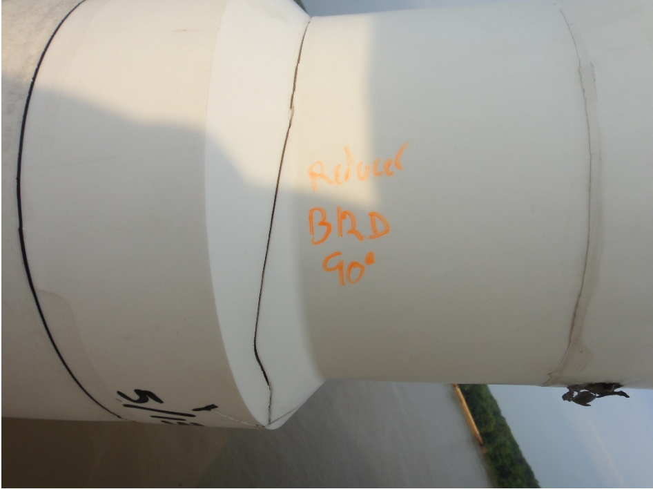
Figure 42. Circumferential Crack in Reducer above Grout Void in Stay Cable B12D.
