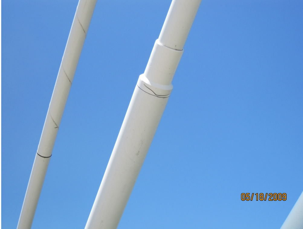
Condition Category 1: Crack in Large End of HDPE Reducer.
