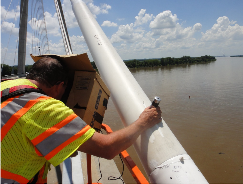
Figure 80. KTC Researcher Using a Digital Microscope Camera to Take Close-up Pictures of Micro-cracking on the Surface of the Coextruded HDPE Pipe of a Connection Sleeve.
