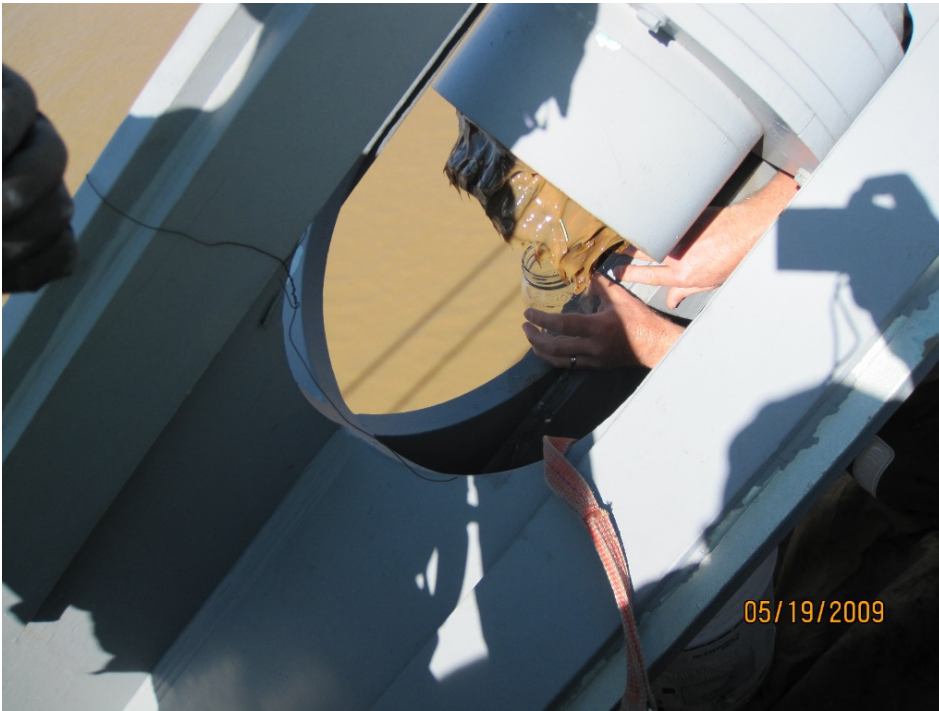
Figure 10. Deck Anchorage Showing Heavy Grease Coating on Strands/Wedges/Anchor Head. Note Water inside Anchorage Piping being Collected
