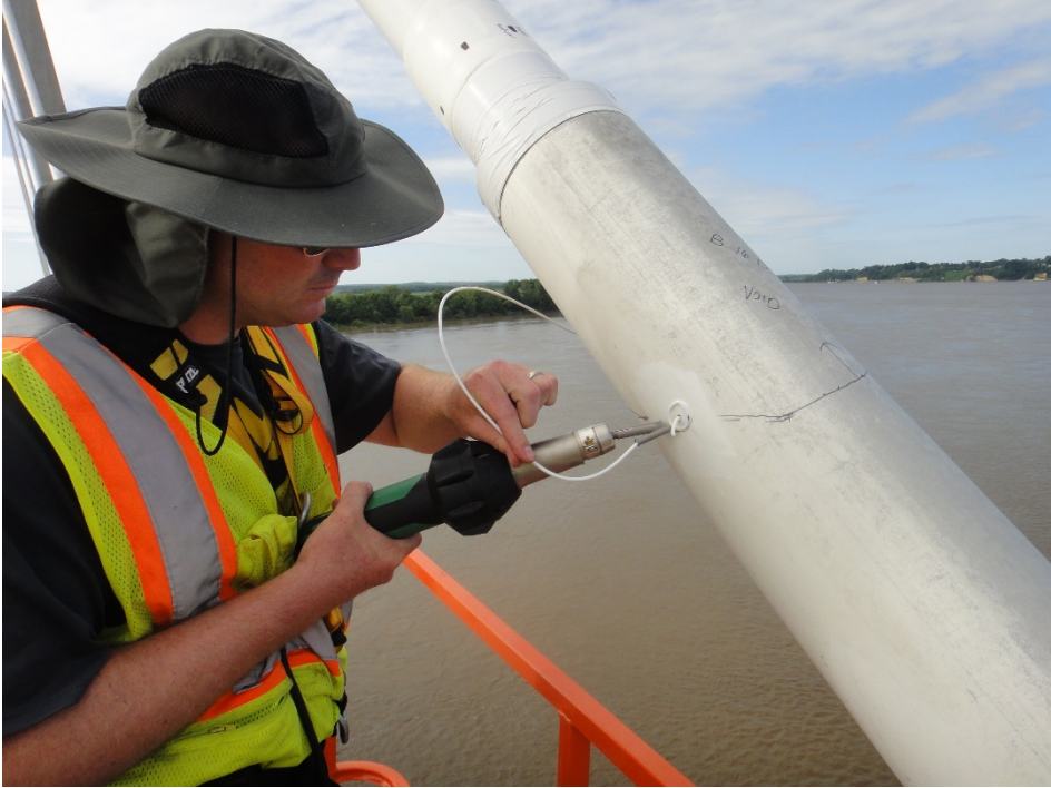
Figure 102. Re-welding HDPE Plug Cut from a Connection Sleeve at a Void Access Hole.
