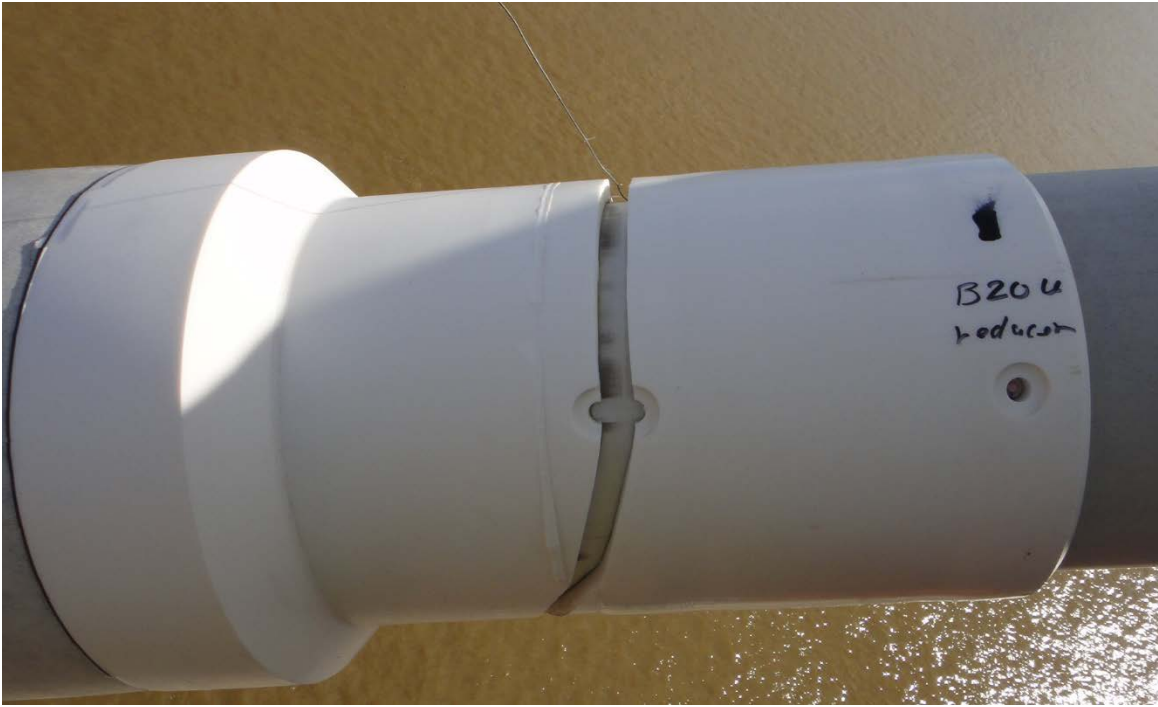
Figure 101. Broken Heating Wire of Electrofusion Weld and Missing Weld Nipples of Cracked Reducer.
