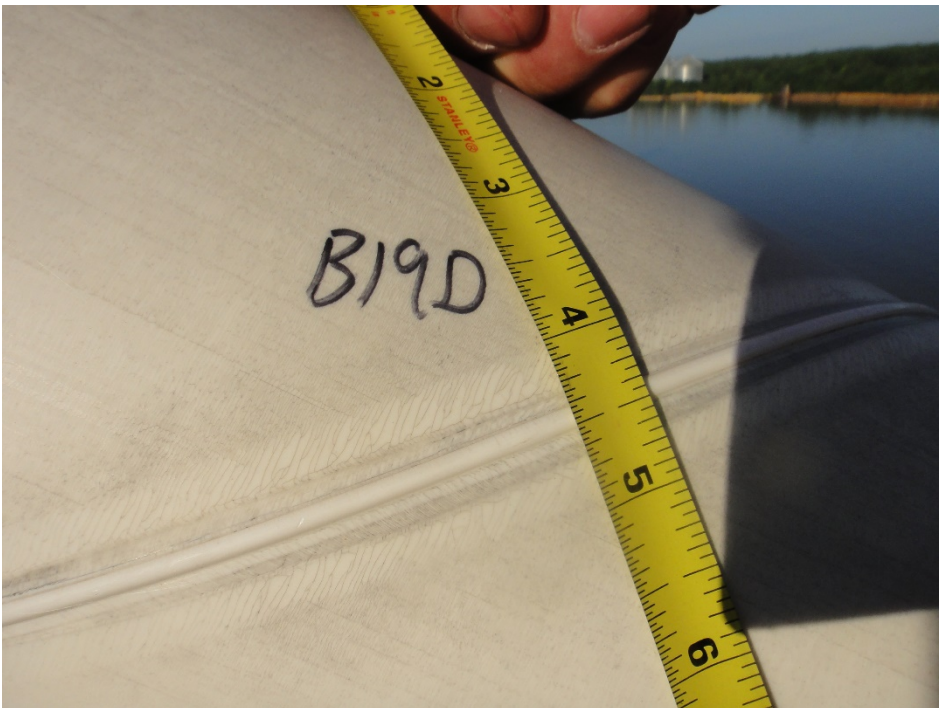
Figure 78. Differences in Micro-cracking in a Stay Pipe Adjacent to the Ribbing.
