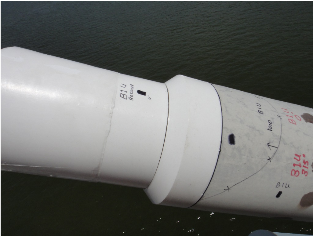
Figure 47. Simple Condition State 3 Cracking Perpendicular to Axis of Piping.
