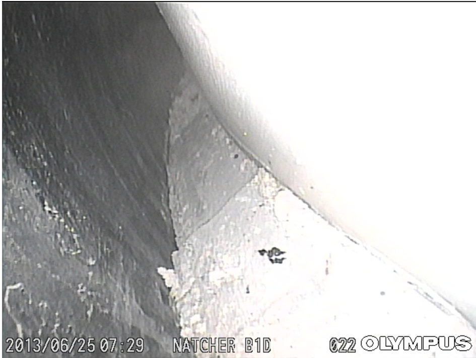
Figure 36. Grout Interface between the Inner Wall of the Connection Sleeve Pipe and the Stay Pipe.
