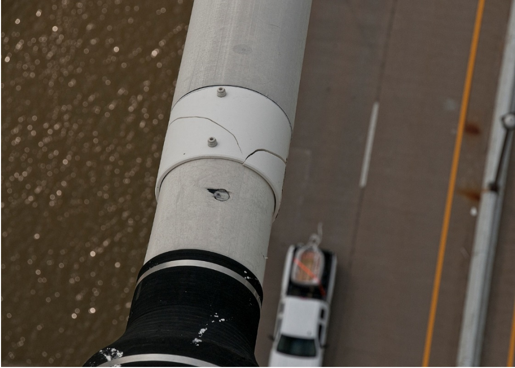
Figure 57. Coupler Crack at Tower Anchorage on Cable B1U.
