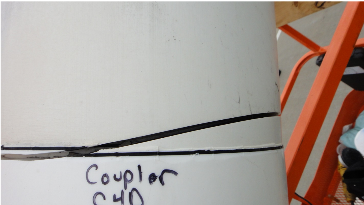
Figure 45. Crack Growth from Coupler Butt Weld into Connection Sleeve Pipe Section (Looking Downward).
