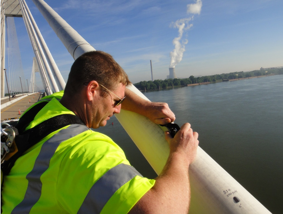
Figure 82. KTC Technician Using Hand Plane to Take Scrape Samples from the Surface of the White HDPE.
