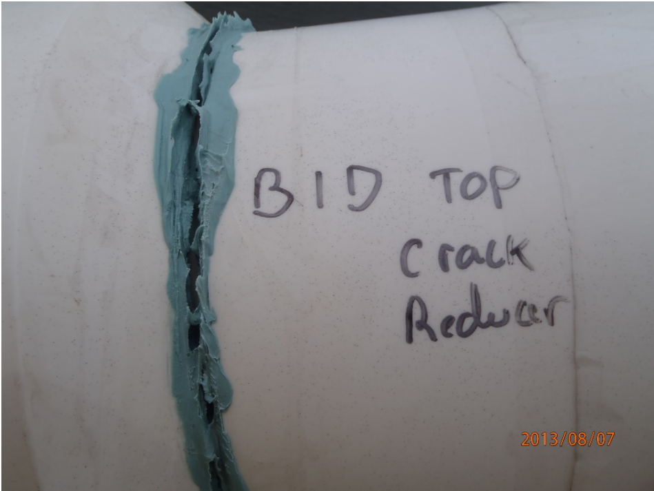
Figure 97. Failure of Stopaq® Paste Seal Found Several Months after the Repair.
