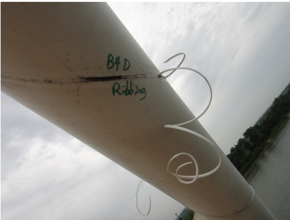
Figure 64. Ribbing Detaching from Stay Pipe near Deck Anchorage
