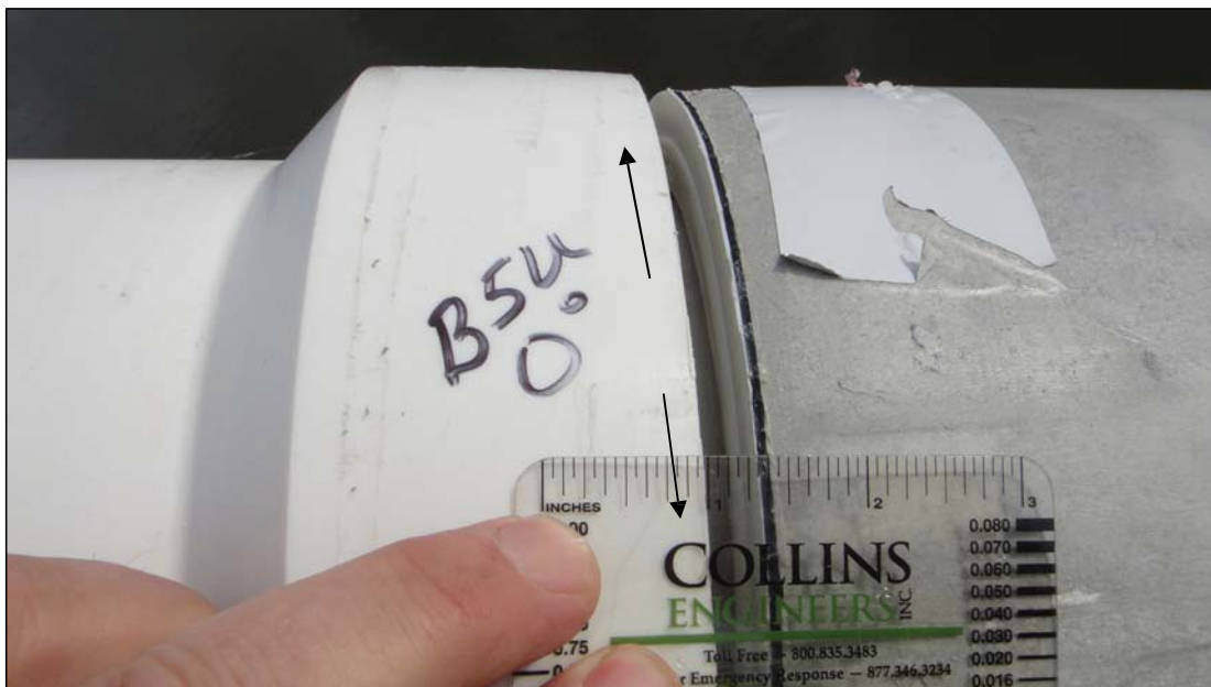
Figure 27: B5U: Reducer Crack at Fusion Butt Weld to Larger Diameter Pipe
