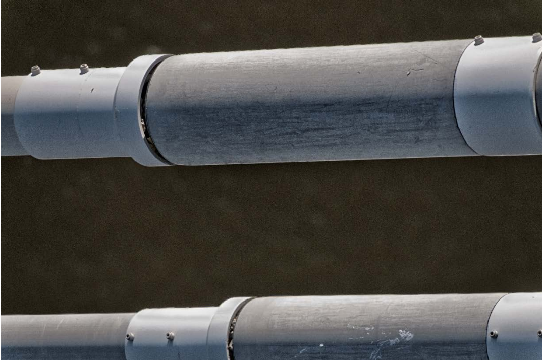
Figure 58. Cables B4D and B5D at Tower Anchorage Showing Gaps Created by Butt Weld Fracture between Reducers and Pipe Sections of Connection Sleeves.
