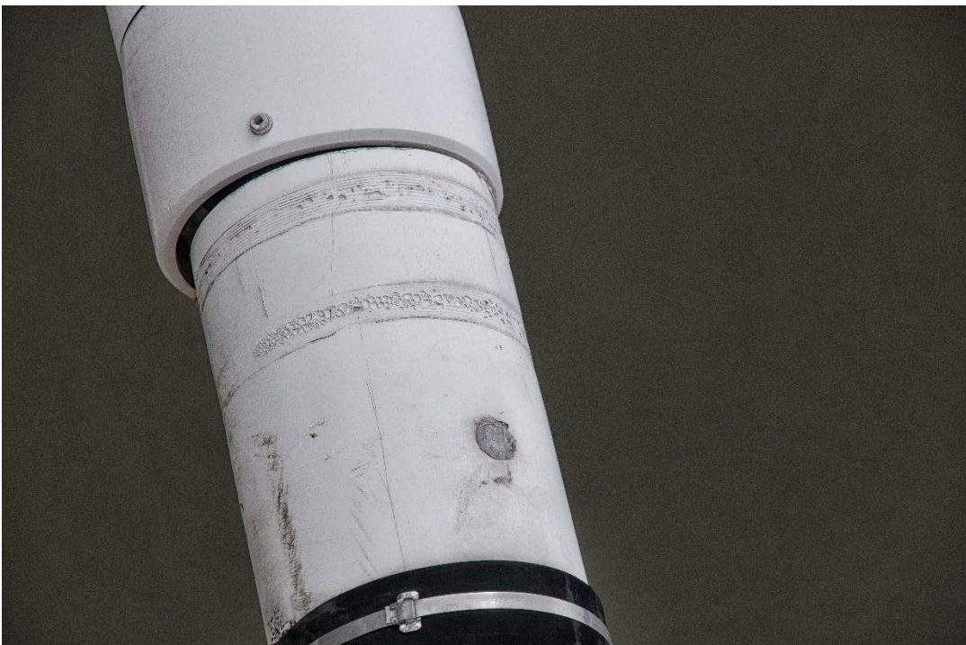
Figure 59. Slippage of Coupler off Transition Pipe at Tower Anchorage B4D due to Shear Failure of Electrofusion Welds.
