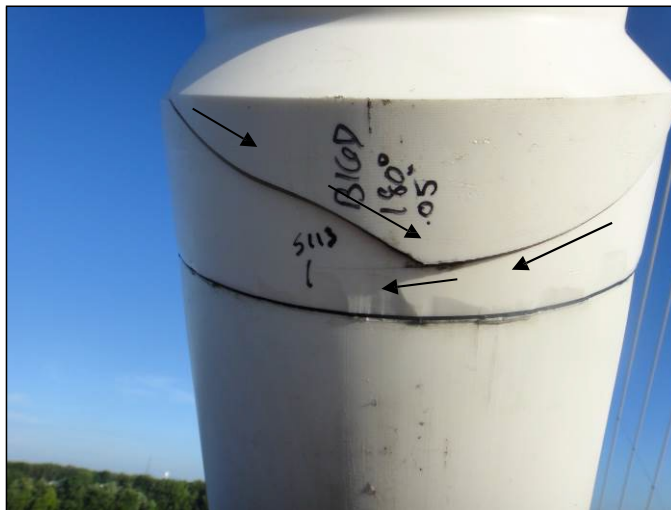
Figure 18: B16D : Reducer Crack at Notch Located at Diameter Transition
