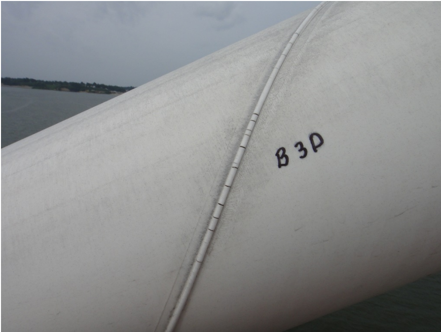
Figure 63. Cracking of Ribbing Still Bonded to Stay Pipe (2013).
