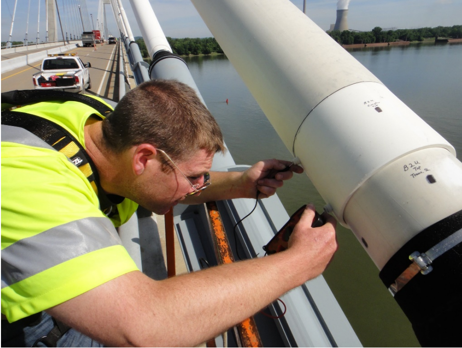
Figure 100. Measuring Resistance of an Electrofusion Weld at the Weld Nipples on a Coupler.
