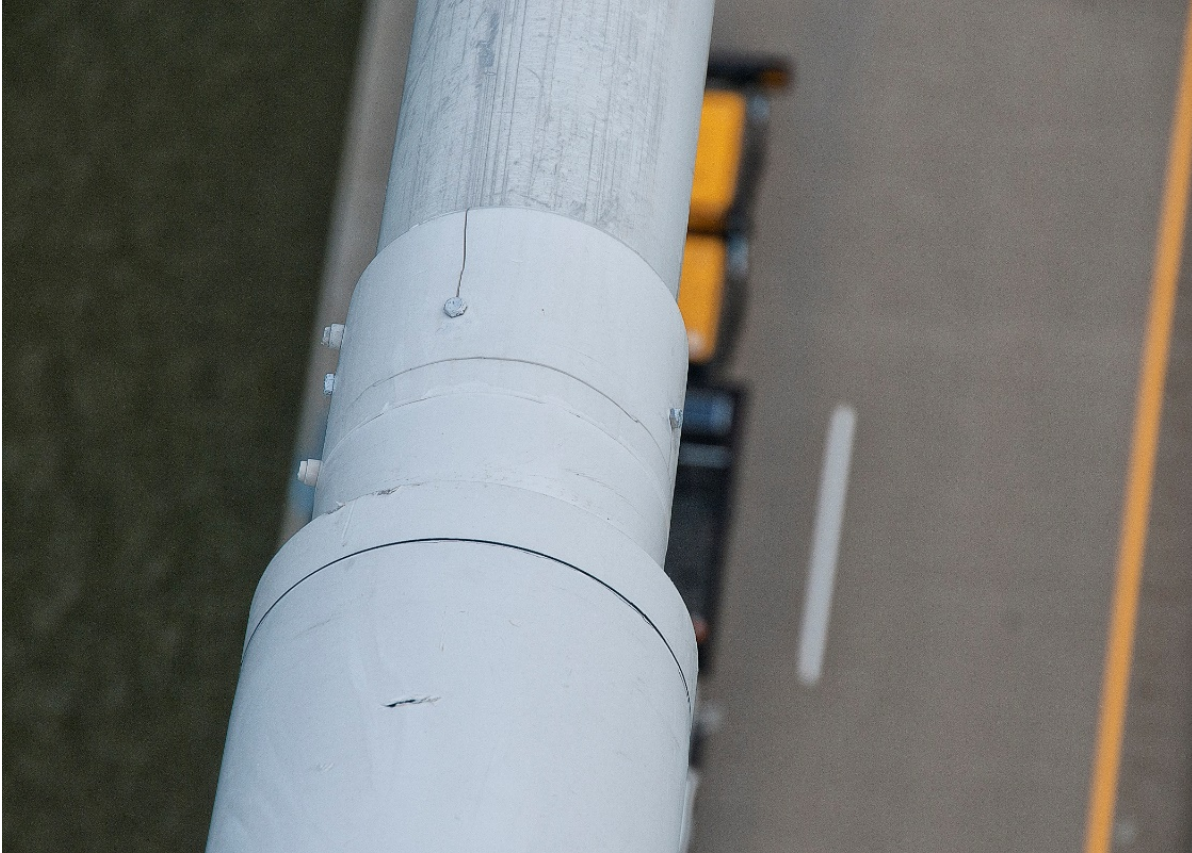
Figure 60. Longitudinal Cracking of Reducer at Lag Bolt Retrofit Added During Construction.
