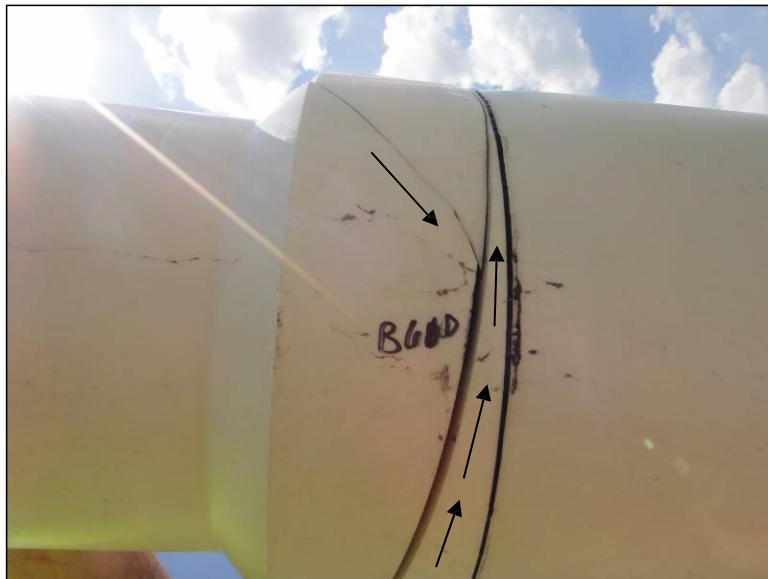
Figure 8: B6D : Reducer Crack at Notch Located at Diameter Transition
