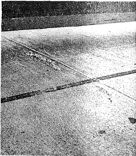
Fig. 6. Joint at Station 622/62 in December, 1949. The first evidence of spalling at this joint was recorded three months prior to this time.
