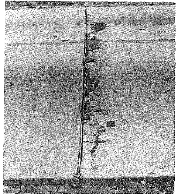
June, 1951. Spalling about the joint extended with time and the bituminous patch material was removed by passing traffic.
