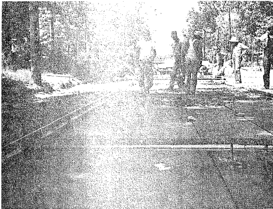
Fig. 14. Experimental aluminum joint in place at Station 70+00. Removable cap is in place.
