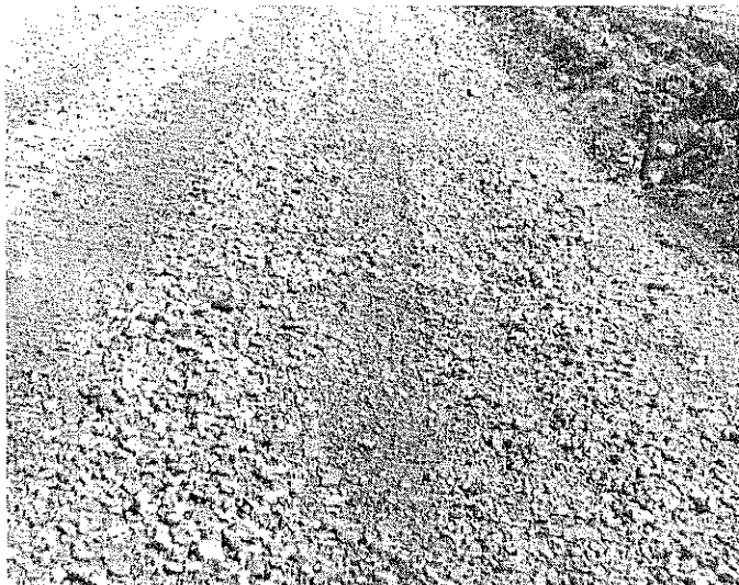
Fig. 24. Raveling of the initial 4-inch base course in Livingston County. A large quantity of gravel 4-inches and larger was contained in this material from the Young pit located between the rivers.
