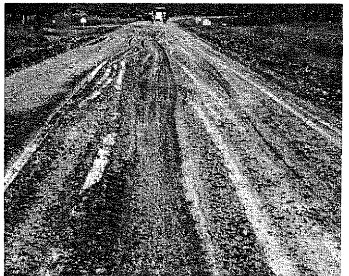
Fig. 18. A freshly laid section of base at Sta. 115+00 which was severely rutted by passing traffic after the rainfall of September 10. Further rutting occurred during and after the rain of September 12-13. Softening was much in evidence with considerable rutting of the uncured portions. Material shown was placed just two days prior to the first rainfall.
