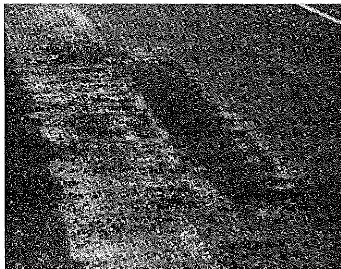
Fig. 23. Location shown in Fig. 22 after four months. The thin porous cold patch was raked from the failure of this picture.
