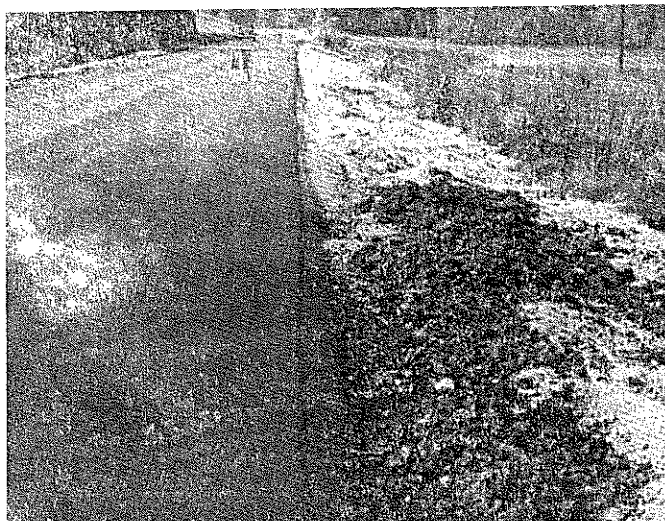
Fig. 20. Weak spot within the 8000-foot section where existing traffic-bound material was trenched 0.7 foot, prior to base construction. Subgrade soil worked up through the base in several spots and kept the base weak even after the bituminous binder was placed. When the surface course reached this section, material was excavated by hand at all the locations showing signs of failure, the openings were backfilled with surface mix, and the pavement finished. Note excavated material on the shoulder.
