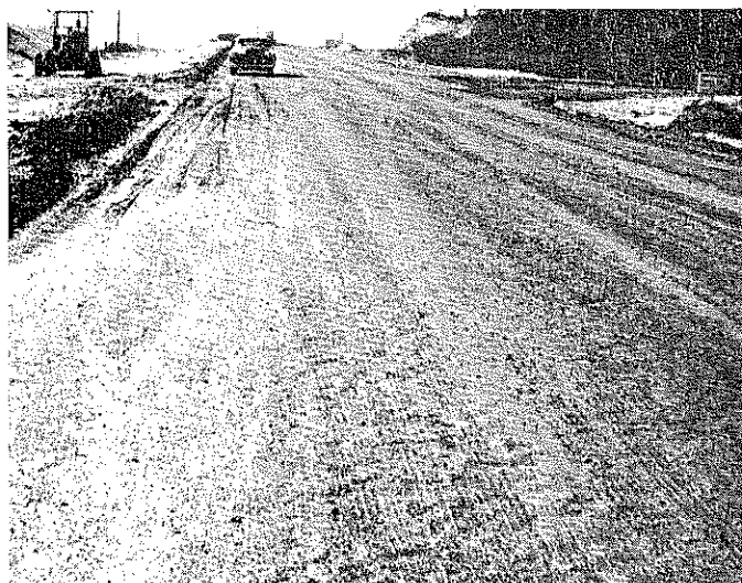
Fig. 26. A section of non-plastic base in Livingston County looking west toward station 450/00. The gravel was from the Max Bohannon pit, and was exceptionally sandy at this point. Note the evidence of non-consolidated material.
