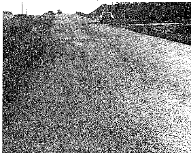
Fig. 27. Patched binder course at the location of the non-consolidated base in Fig. 26. The dark section in the center of the pavement is not a patch but was caused by a badly cracked condition. Conditions shown existed about four months after the binder course was laid. Final surfacing of this portion of the road will be carried out during the 1952 season.
