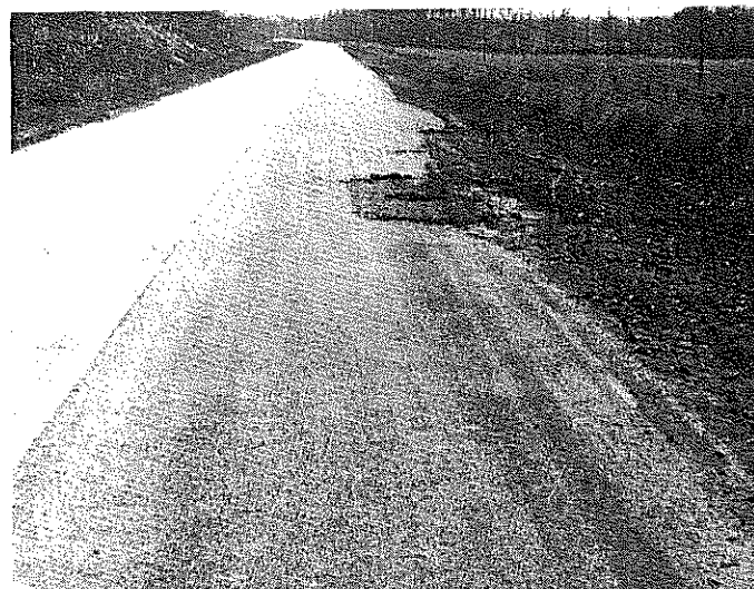
Fig. 21. Location shown in Fig. 20 after four months. The cracked pavement has been patched with a thin layer of porous cold patch. There was very little bond between the patch and the pavement. The failure is confined to the right wheel track of the north lane for a distance of 15 to 20 feet.
