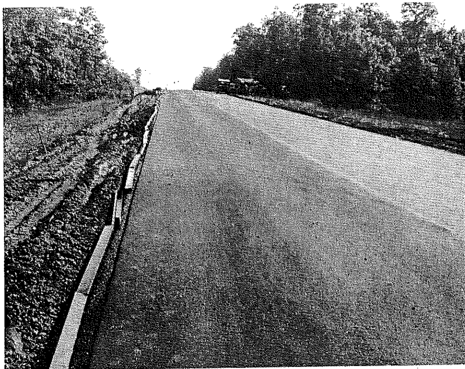
Fig. 19. Finished pavement at about Sta. 190/00 as it appeared on October 8, 1951. A section of the finished base under the left (North) lane was soft and shoved under loads at the time of bituminous binder-course construction. This condition existed in three spots totaling about 1000 feet in length. Upon examination it was found that the binder soil and gravel in the first 2-inch course of stabilized base had not been properly mixed and that lenses of binder soil were present. Records showed that this binder soil had been placed on the road and became very wet while in a windrow, and it remained wet at the time of mixing with the gravel.
