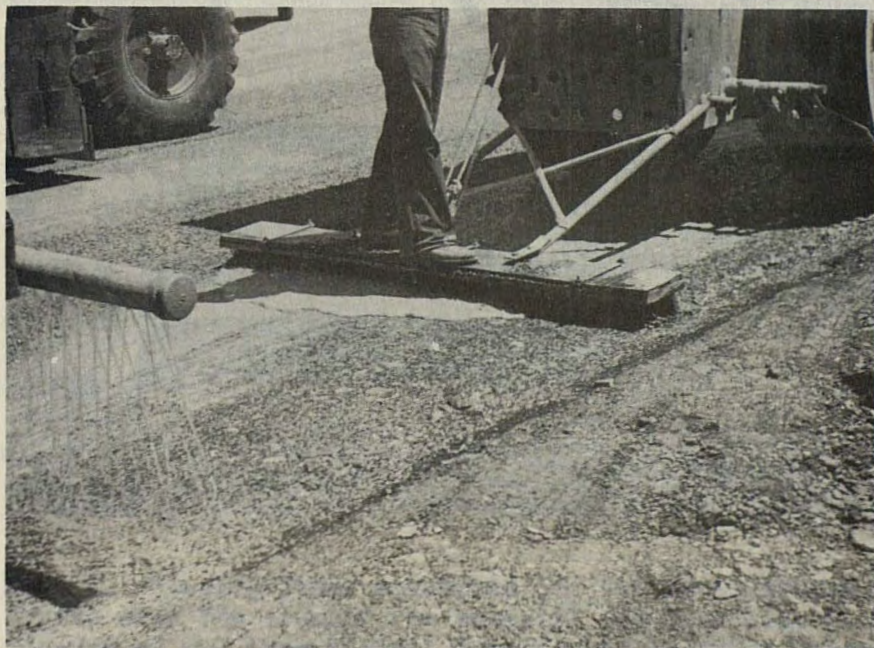
Fig. 4. Watering, brooming and rolling on the water-bound construction. Note slurry in front of the broom.
