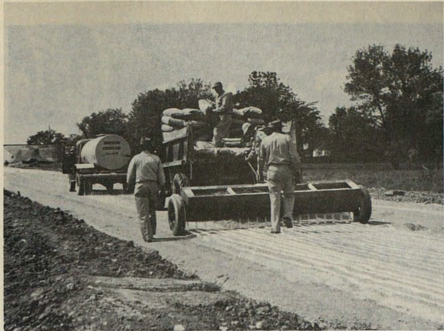
Fig. 7. Water was applied to thoroughly wet the stone prior to application of calcium chloride. This was done to assure an adequate moisture content and prevent segregation as well as facilitate manipulation during the mixing process that followed.
