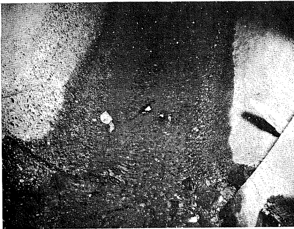
Fig. 14 - Interior of reinforced concrete pipe. Exposure of coarse aggregate has resulted from corrosion and removal of mortar by acid water. Date-August, 1954 Age - 4-1/3 yr.
