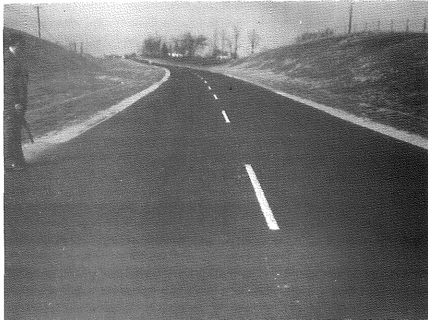
Fig. 6 - U. S. 27 south of Lexington showing where entrance was made through the crust near scaling in the wheel tracks.
