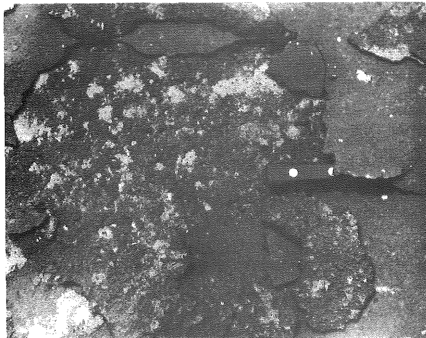
Fig. 2 - Close up of the section in Fig. 1 showing loosened crust and pockets of stripped sand. The surface was not broken here until this exposure was made. Crust contained 6.94% asphalt by extraction; 77°F Pen. - 36. Asphalt in the material underlying the crust seemed much softer.
