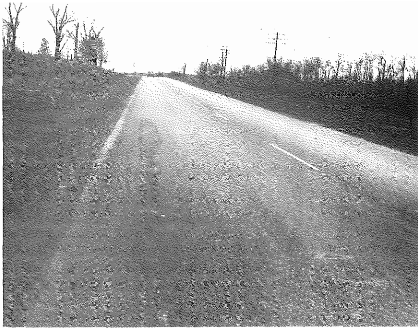
Fig. 5 - U. S. 27 south of Lexington, showing typical scaling in the outer wheel track of the left lane. On this road, these failures were very localized.
