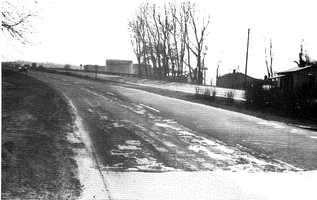
FIG. 46: Section I, Control A, Northbound Lanes. This general view looking southward from Sta. 0+00, shows severe rutting in the outside lanes. Damage began approximately six weeks after construction. Since then the damaged areas have been patched twice. The bright areas are remnants of patch material enriched by heavy applications of prime coat.
