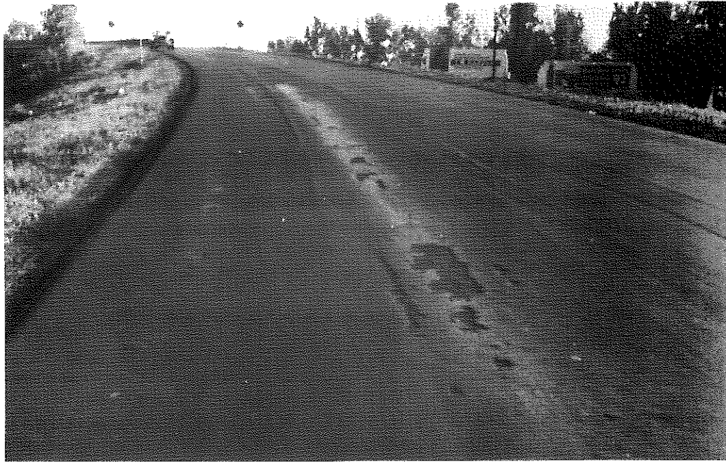
FIG. 33: Section I, Control B (Same as Figs. 31 and 32). After about three days, traffic had fairly well compacted and stabilized the material; but the earlier condition left the surface rough, deeply furrowed and in need of correction.
