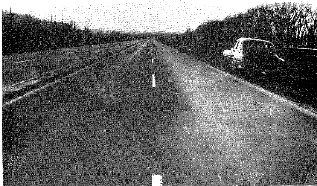
FIG. 57: Section IV, Dry Heated to 235°F, Southbound Lanes, Showing Only Isolated Scaling in Outside Lanes. Similar material in opposite lanes also shows only very slight amount of failure.
