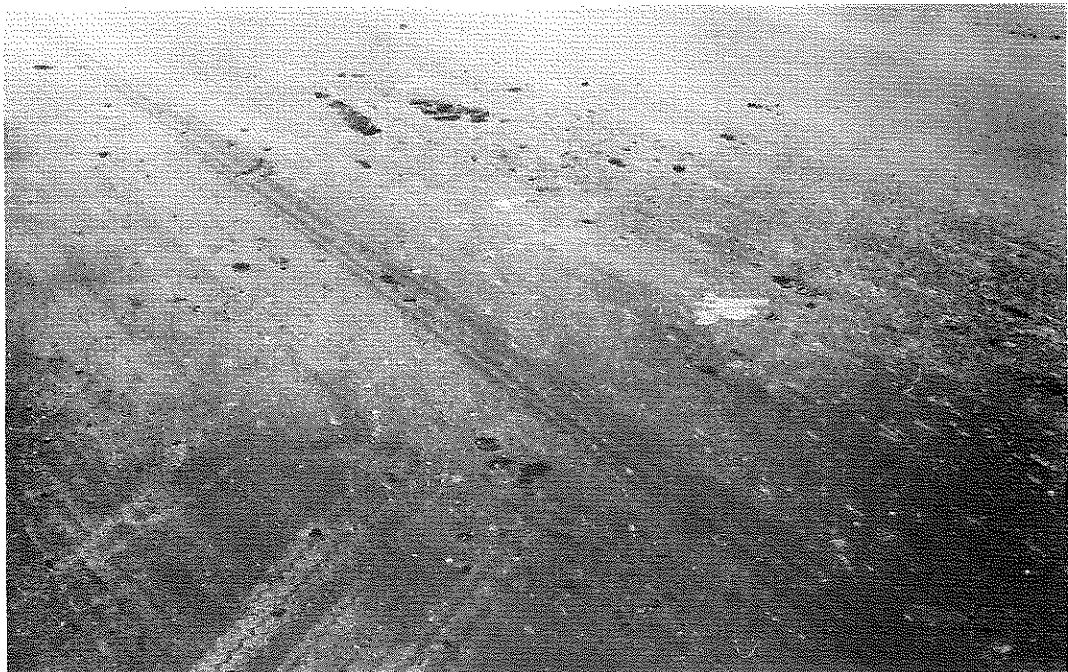
FIG. 40: Section VI, Containing Powdered Asphalt, Dry Heated. Cinders, or clinkers, due to overheating and coking show up as pop-outs. This section was not paved to the full 1-in. depth. Actually about 60 lb. per sq. yd. were used and clinkers were less likely to be submerged. These seemed to encourage scaling around their perimeter.
