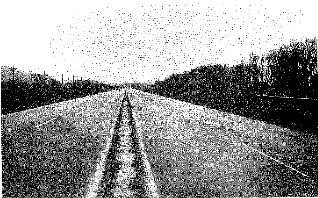
FIG. 55: Section III, Steamed, Containing Powdered Asphalt No. 1. Foreground shows well developed scale in outside wheel tracks. Inside lanes are undamaged. Section IV, dry heated to 235°F. Background is practically free of damage except for a few isolated spots of scale. Similar materials in opposite lanes are only slightly damaged.
