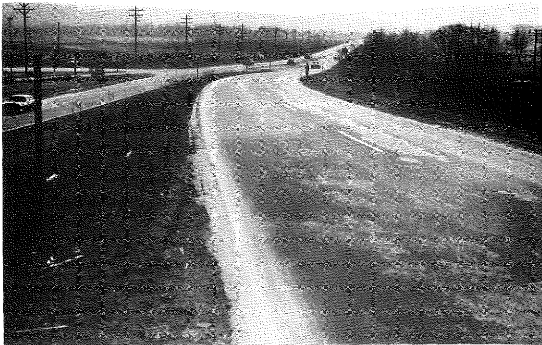
FIG. 49: Section I, Control B, Southbound Lanes. Extensive rutting is confined to the outside lane. This area was patched, soon after laying, with a thin overlay.
