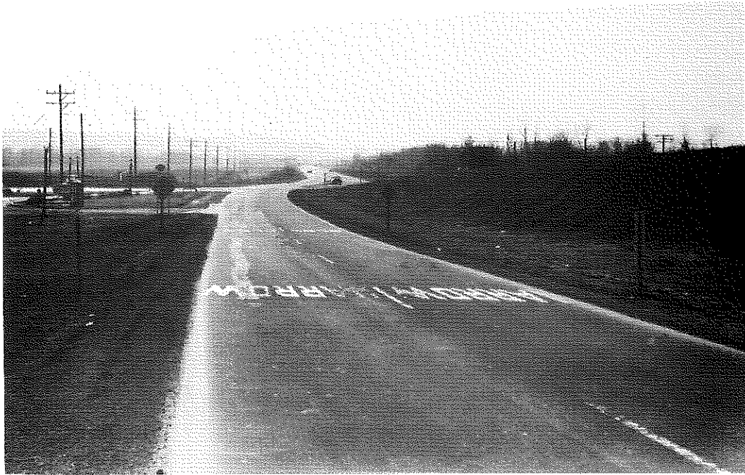
FIG. 48: Section I, Control A, Northbound Lanes. Showing Scaling in Wheel Tracks of Outside Lane. The bright areas are patches. This area was reworked with the heater-planer after 2 months because of the development of small hairline cracks. Treatment apparently retarded but did not prevent scaling.
