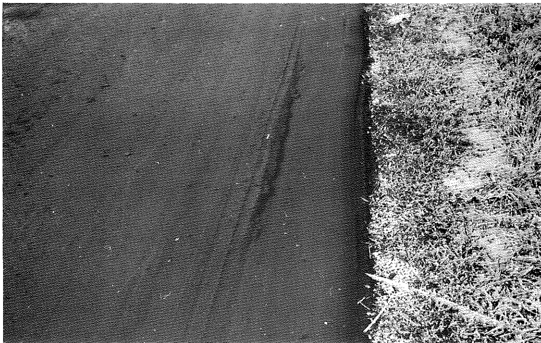
FIG. 32: Section I, Control B (Same as Above) Showing Severe Shoving and Displacement. At some locations as much as 4 in. of the surface was shoved off the edge of the pavement. The wheel tracks were rather deeply furrowed, and some material picked-up on the tires.
