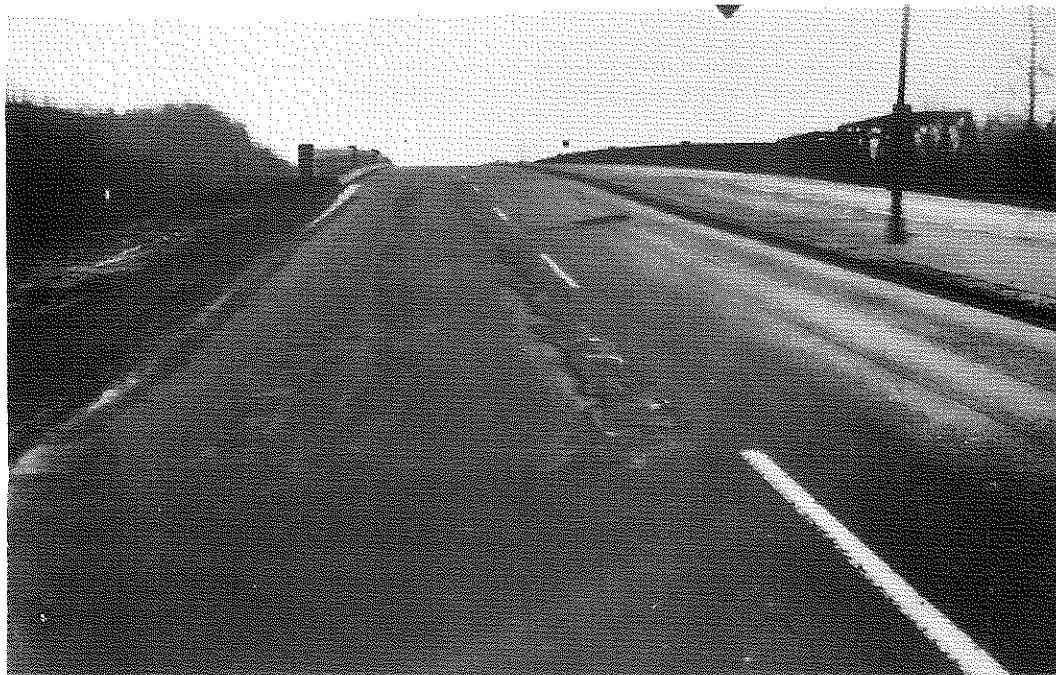
FIG. 59: Section VI, Containing Powdered Asphalt No. 2, Dry Heated, Northbound Lanes. Failure seems to be rather general throughout this section, but again only in the outside lanes.
