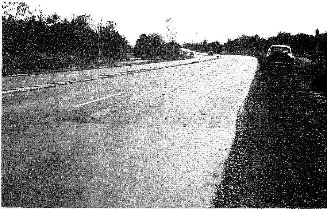
FIG. 43: Unscheduled Section Containing Powdered Asphalt No. 2, Steam Heated. During construction, hydraulic fluid from the paver leaked onto the roadway. Although this was mopped and broomed away, the material quickly rutted out of the wheel tracks. Accordingly, this section has been eliminated from further consideration in the evaluation of performances. The undamaged section in the foreground is dry heated material containing 3 percent PAC-3.
