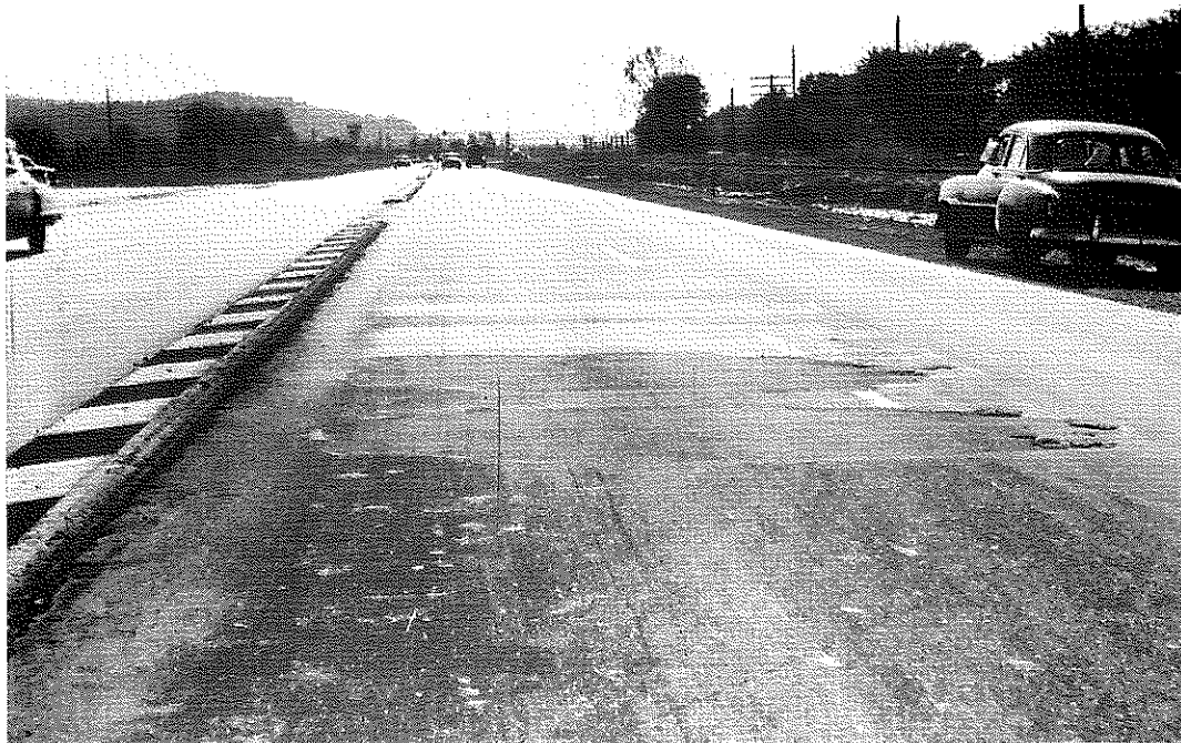
FIG. 42: Example of Very Severe Damage Resulting From Fuel Oil Spilled During the Construction of the Raised Median Divider Strip. Fuel oil was evidently used to clean shovels, etc. This photo was taken after patching. Oil was tracked a considerable distance in the direction of traffic, and softened the surface, showing as bright spots, but caused no damage requiring patching.
