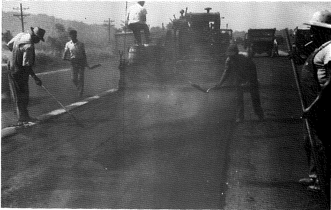
FIG. 37: Paving with Dry Heated Materials. The vapor rising from the pavement had a bluish color which presumably indicated volatilizing oils. This was common to all dry heated materials, particularly above about 220°F. Note raker at left removing a clinker. The particular mixture here contained 2 percent PAC-3.
