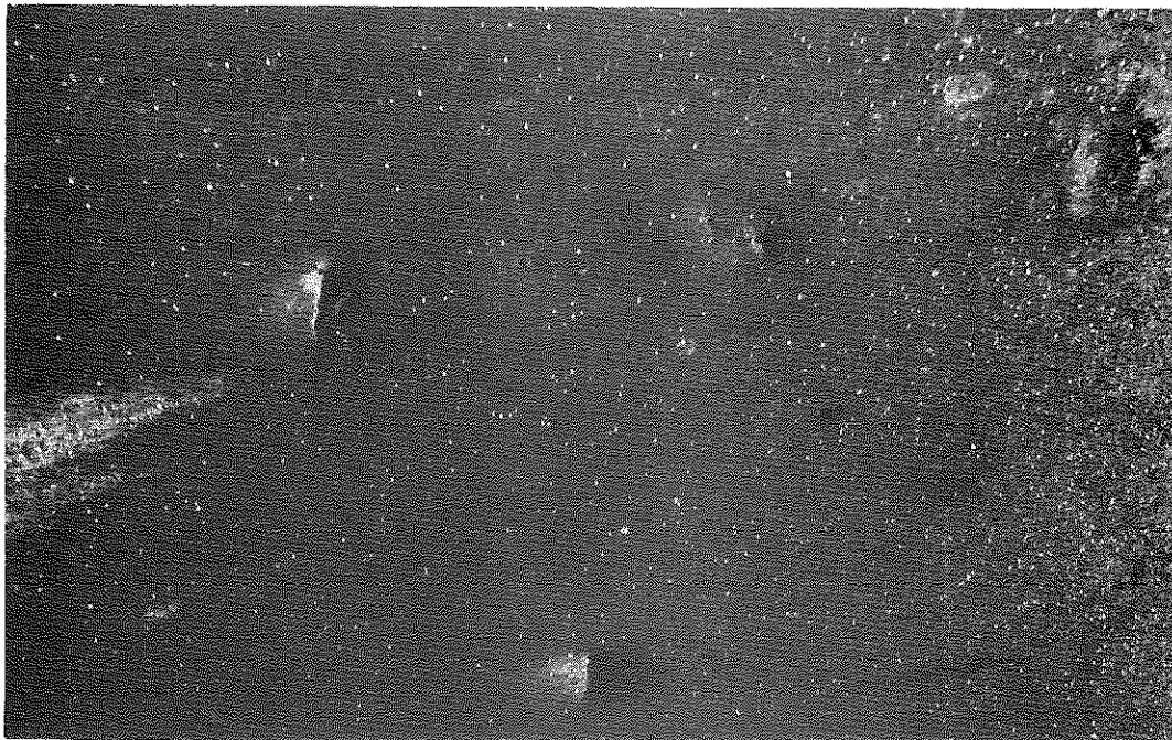
FIG. 38: Typical Example of Bubble Formation in Dry Heated Materials. Most of these seemed to occur near the middle of the lane and in material which had been in contact with the hottest part of the screed.
