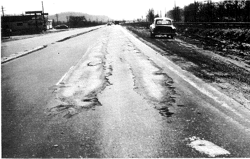
FIG. 54: Section II, Antistrip No. 3, Used in Southbound Lanes Only. This view shows the transition from Antistrip No. 2 (foreground), undamaged, to Antistrip No. 3, damaged. Only the outside lanes with No. 3 show appreciable failure.
