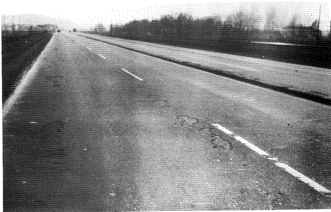
FIG. 52: Section II, Antistrip No. 1, Northbound Lanes. Scaling has developed in the outside lane while the inside lane is undamaged. Section containing Antistrip No. 2 is similarly affected but to a lesser extent.
