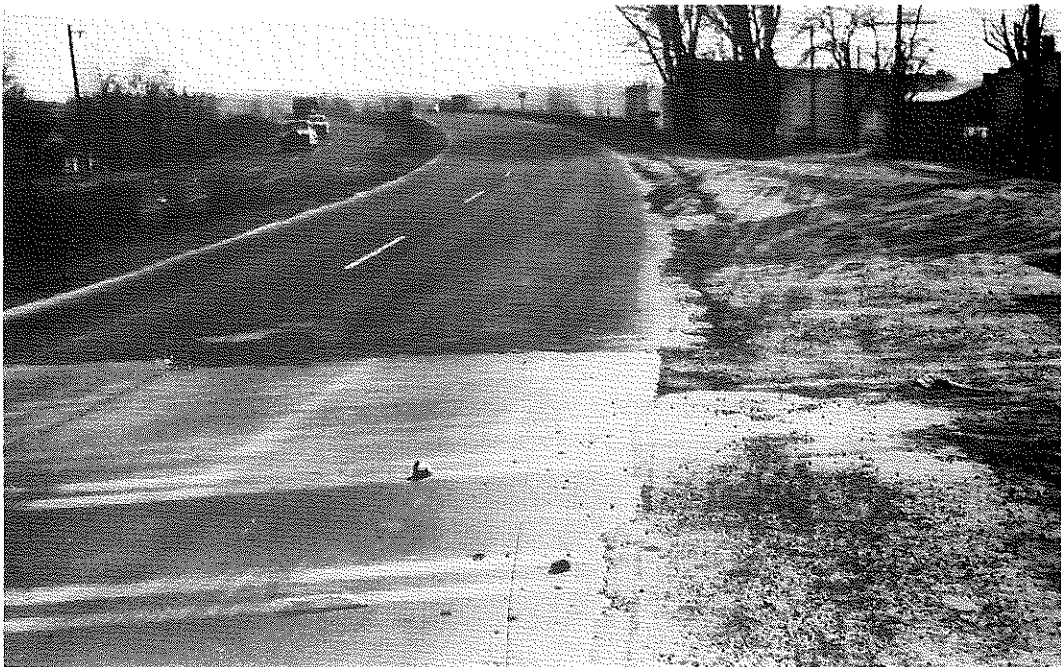
FIG. 47: Section I, Control B, Southbound Lanes, Looking Southward from Sta. 0+00. Rutting is practically continuous throughout the entire section but has been confined almost exclusively to the outside lane. This section has also been patched twice previously.
