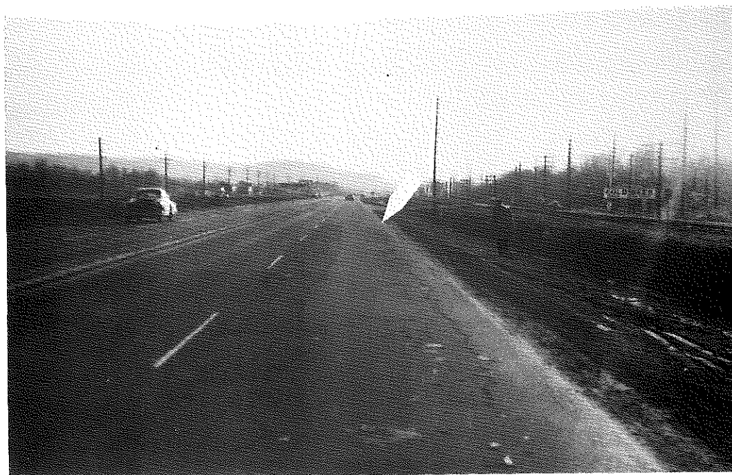
FIG. 53: Section II, Antistrip No. 1 and No. 2, Southbound Lanes. Scale here is 1/4 to 3/8 in. deep. Joint between No. 1 (foreground) and No. 2 (background) is indicated by arrow. No. 2 has not suffered in these lanes but has scaled in the northbound lanes.
