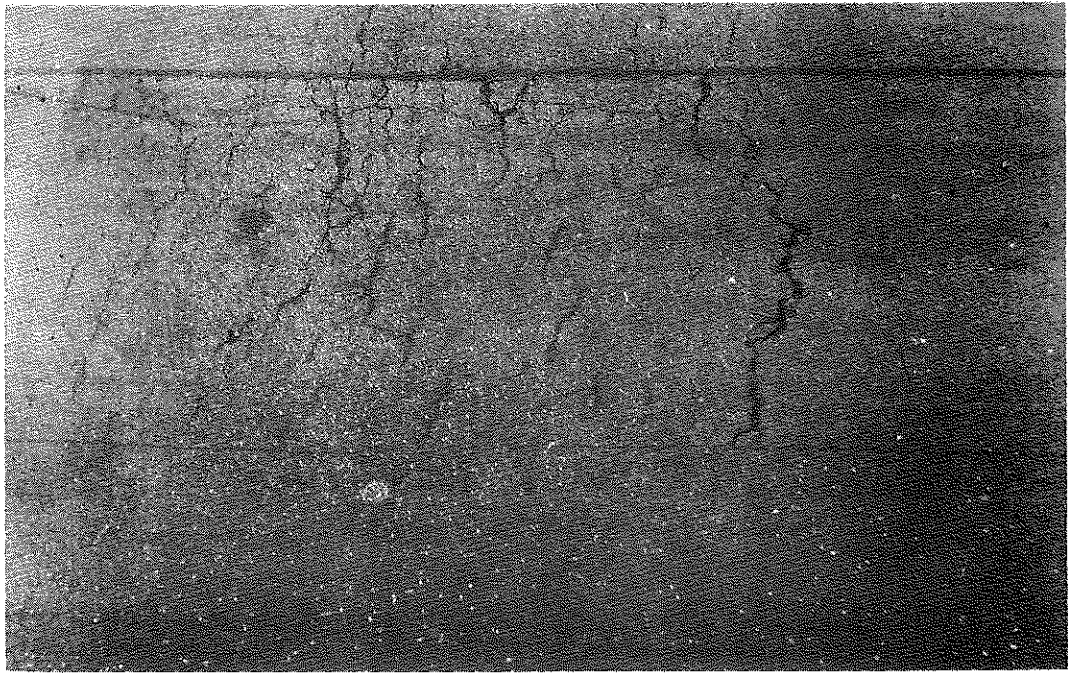
FIG. 39: Section IV, Dry Heated. The small area shown was overheated and partially coked by the hot screed while paver stood idle between deliveries of material. Usually these were removed and replaced; but a few spots were left for observation, and later patched.
