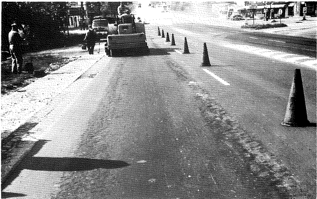
FIG. 44: Section VI, Containing 1 Percent Powdered Asphalt No. 2, Dry Heated. Only 60 lb. per sq. yd. were laid on this section. Continuous pitting and loss of material from the wheel tracks are evident in the outside lane. Heater-planer is shown in the background attempting to re-smooth the section.
