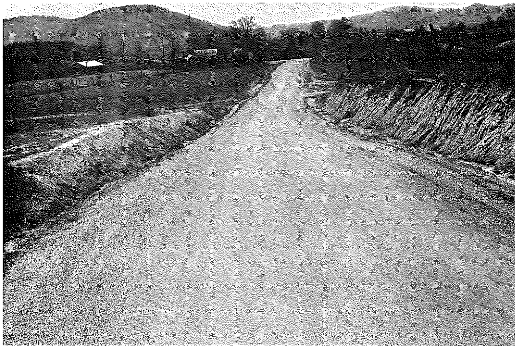
Fig. 51: Madison Co.: Section Where Culverts Were Installed. Some damage due to flood has occurred. Wheel-tracks show considerable deformation which may have been caused by heavy logging trucks. (4-24-57)
