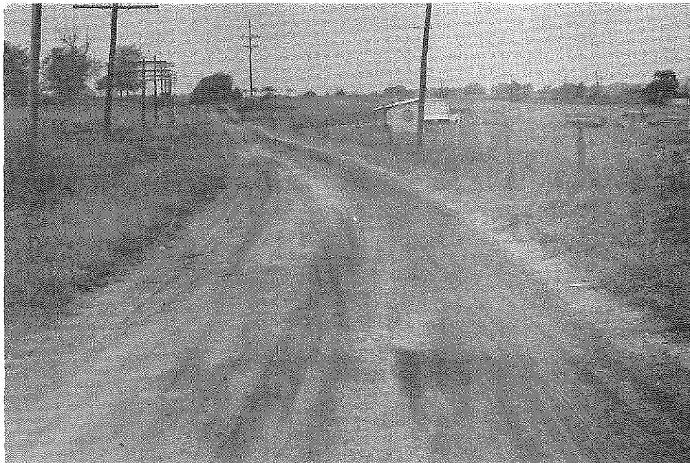
Fig. 3: Breckinridge Co.: Same Road as above before Stabilization, Looking West. Note markedly different condition of original surface. (Before 10-2-56)
