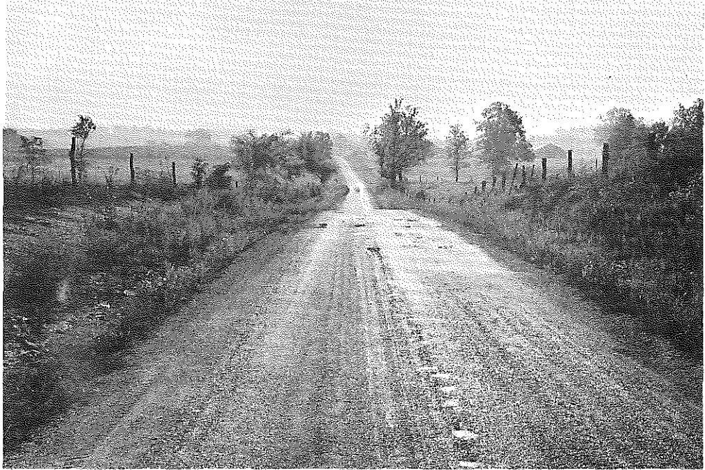
Fig. 62: Montgomery Co.: Section Affected by Underlying Shale and Poor Drainage. (8-20-57)
