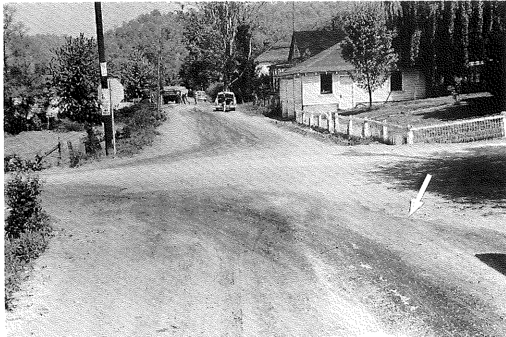
Fig. 83: Johnson Co.: Raveling and Pot-Holes in W. Van Lear Section. Maintenance crew adding more rock to bog shown in Fig. 80. (5-2-57)
