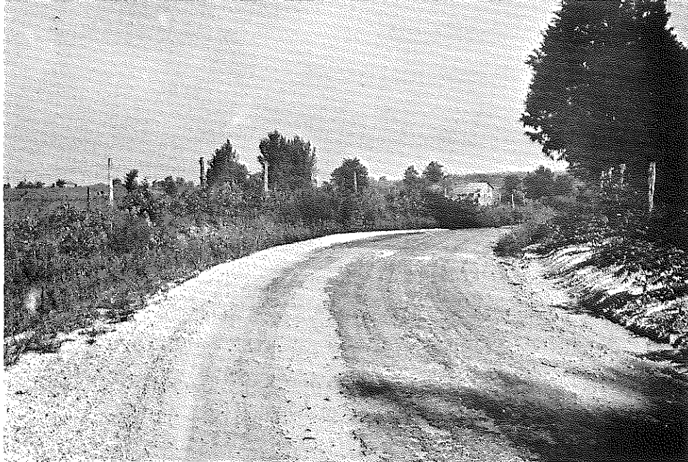
Fig. 60: Montgomery Co.: Curve Showing Wear and Raveling. (8-20-57)
