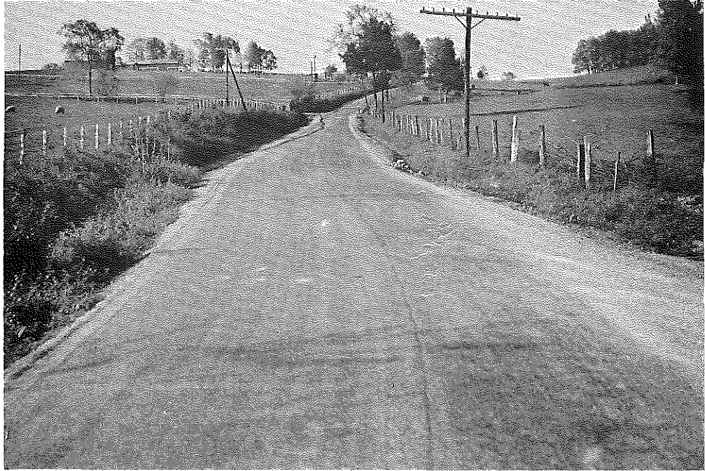
Fig. 40: Barren Co.: Similar Section after 7 Months. (4-24-57)
