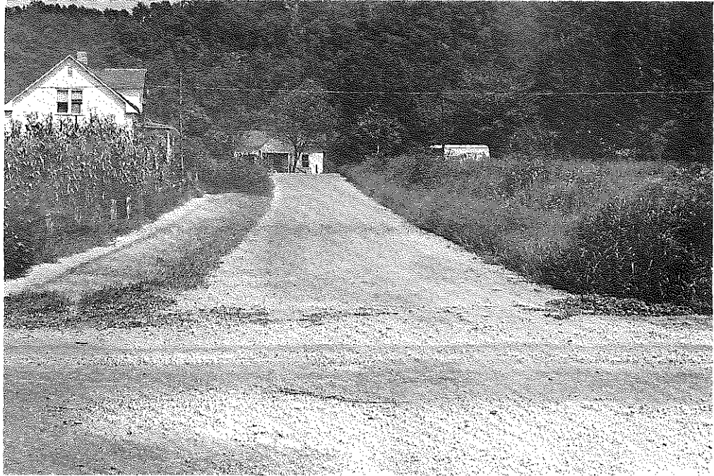
Fig. 86: Johnson Co.: Short Cross-Street in W. Van Lear. Several streets such as this were stabilized but none of them carries much traffic. (8-20-57)
