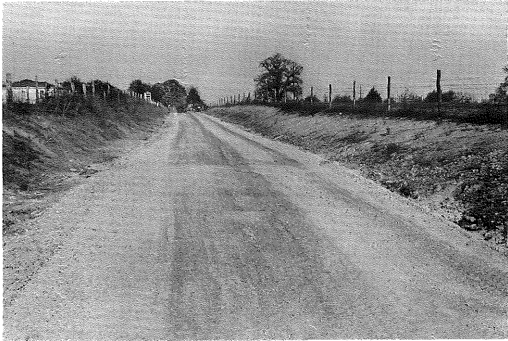
Fig. 58: Montgomery Co.: Shale Outcropping and Poor Side Drainage, which Cause Poor Performance. (5-27-57)
