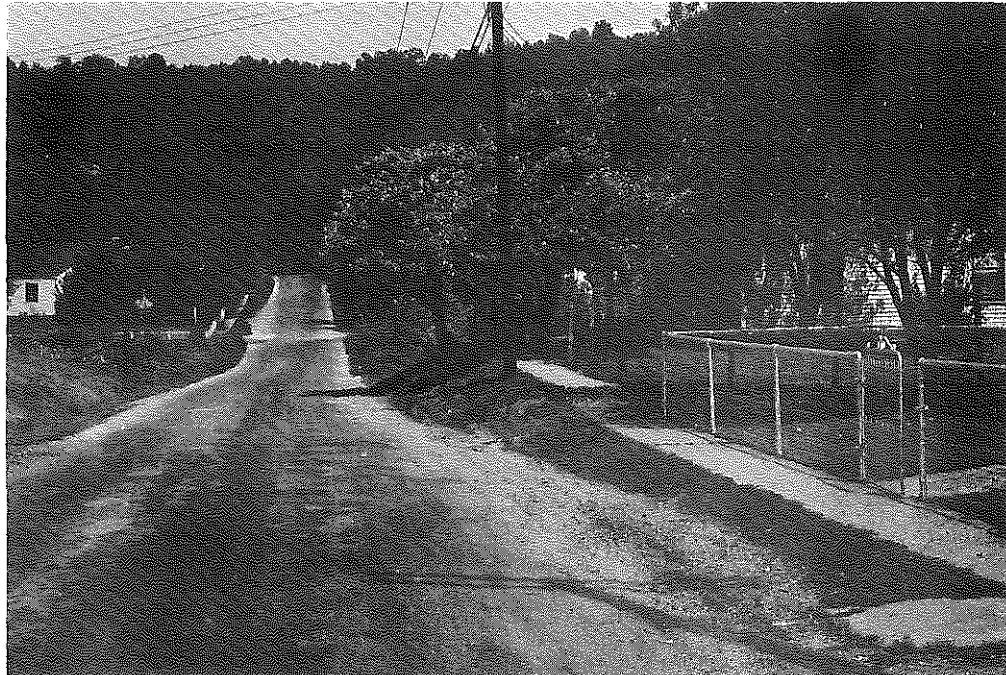
Fig. 84: Johnson Co.: Same Street Shown in Previous Fig. Softness occurred at one spot because of clay pocket in the left foreground. (8-20-57)
