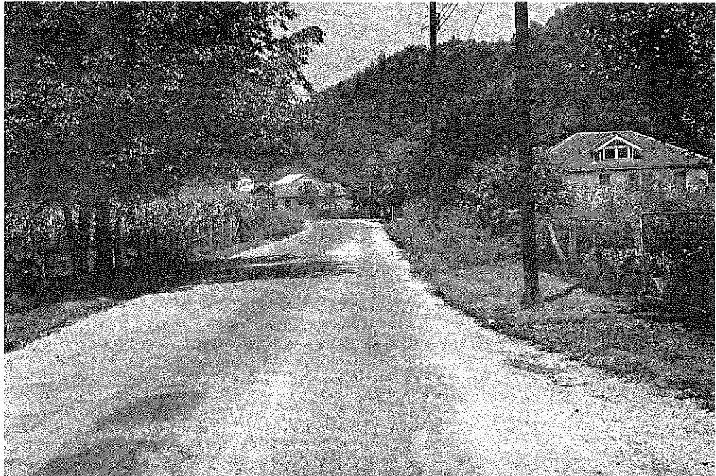
Fig. 87: Johnson Co.: Section Last Stabilized. This received a heavier application of SS-1, and some softness has resulted. (8-20-57)
