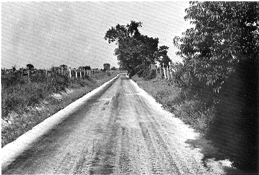
Fig. 61: Montgomery Co.: Section Showing a Few Pot-Holes. However, condition is generally good. (8-20-57)
