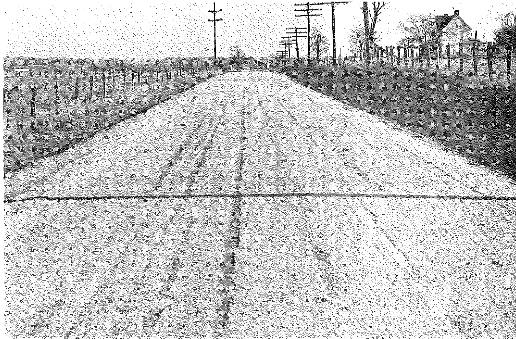
Fig. 9: Breckinridge Co.: General Condition of Road after about 2-1/2 Months. Failure of seal coat to stick is attributed to absence of prime. (1-3-57)
