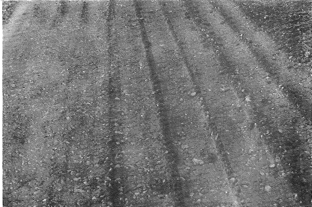
Fig. 22: Ballard Co.: Close-up of AE-200 - Bank Gravel Base after First Pass of Pneumatic Roller. (10-12-56)
