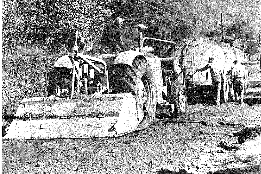
Fig. 76: Johnson Co.: W. Van Lear. Trav-L-Plant Connected Directly to SS-1 Transport. SS-1 was mixed in single pass, re-blended later. Existing roadbed was scarified preparatory to mixing with emulsion, no additional granular material required. (10-29-56)
