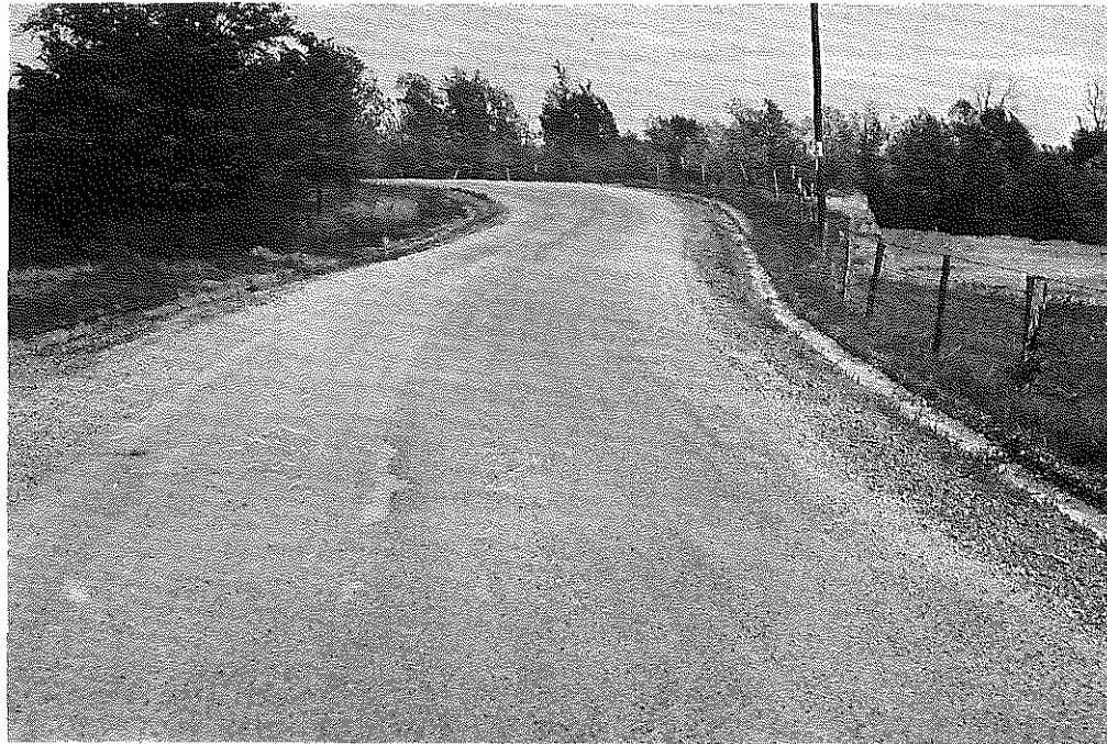
Fig. 33: Marshall Co.: Seven Months after Stabilization. General performance and appearance have been good. Note gravel pit immediately to the right of roadway. (4-24-57)
