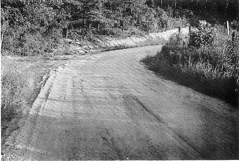
Fig. 52: Madison Co.: View of Curve Shown in Fig. 50, after 10 Months. (8-5-57)
