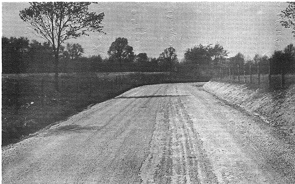
Fig. 11: Breckinridge Co.: General Condition of Seal after about 7 Months. (4-24-57)
