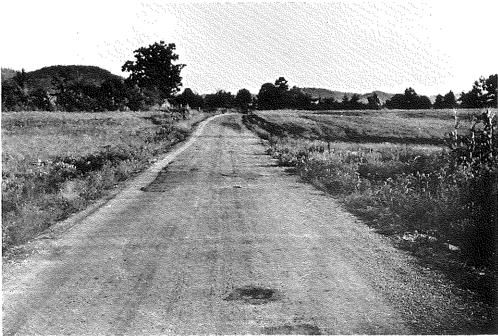
Fig. 53: Madison Co.: View of Section Where Culverts Were Installed, 3 Months Later. Some patching has been required. (8-5-57)
