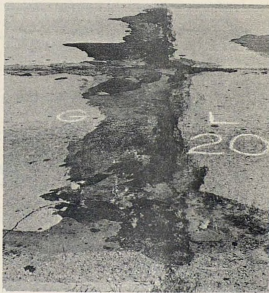
D - Greatly enlarged crack or joint, with excessive spalling and corner breaking
