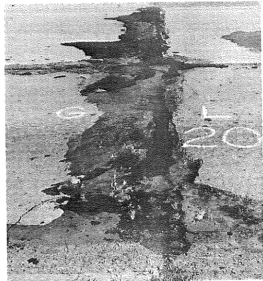
D - Greatly enlarged crack or joint, with excessive spalling and corner breaking
