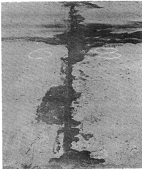
C - Enlarged crack or joint, showing considerable spalling and corner breaking
