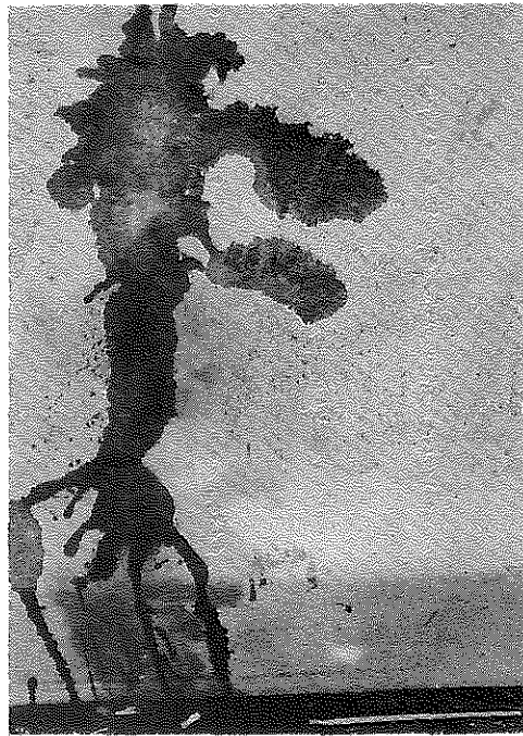
Fig. 17. This Close-up of a Flooded Crack Showed the Effect Obtained with a Thicker Coating of epoxy and sand. The crack was well sealed as evidenced by its refusal to allow ingress of water.
