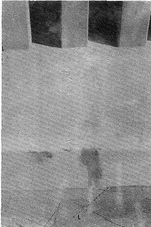
Fig. 8. This is a Typical Crack After the Resin and Sand has been Applied and the Mixture Flattened out to Fit the Contour of the Existing Concrete.
