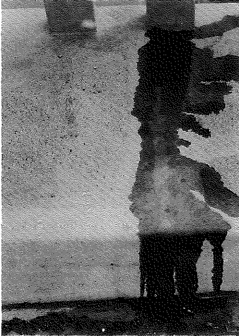
Fig. 16. This is a Typical Crack After 6 Months Service which was Flooded to Detect any Seepage. No water entered the crack and its water tightness was verified. The outline of the crack can be seen here through the thin covering of transparent resin. If it had been possible to apply more sand before the swath of resin hardened the sealed crack would not have been visible. However, the crack was sealed and the concrete and steel protected.
