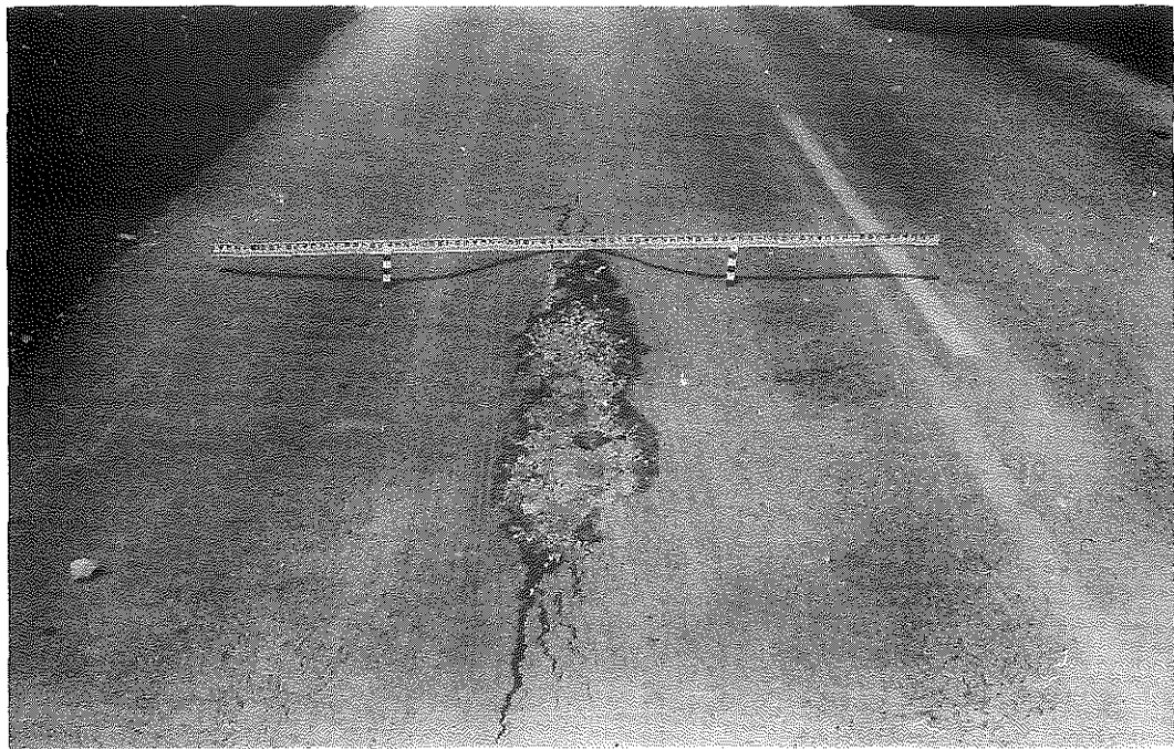
Fig. 8: Photograph Illustrating Extreme Rutting and Upheaval.
