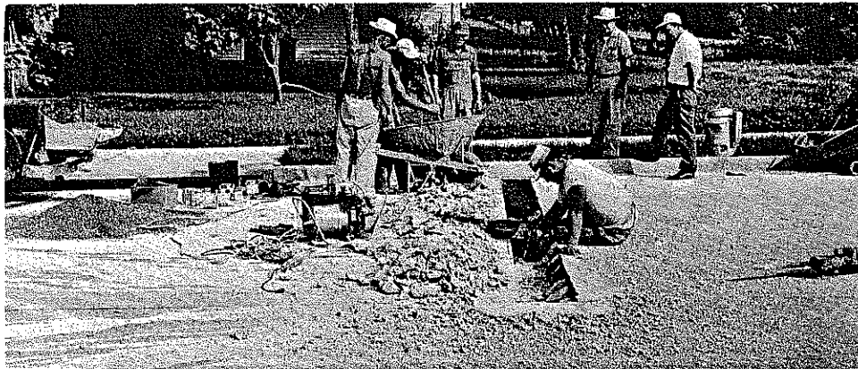
Fig. 7. Routed Defective Area at Station 63 + 27. A groove was formed along the right hand edge of the repair area; the hole is primed with epoxy and some epoxy patching material has been placed as backfill, 6-7-62.
