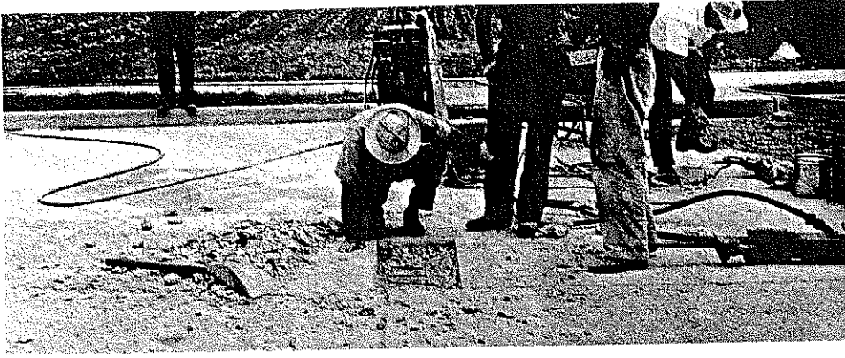
Fig. 1. Defective Area at Station 55 + 75. Hole has not been completely routed and cleaned, 6-7-62.
