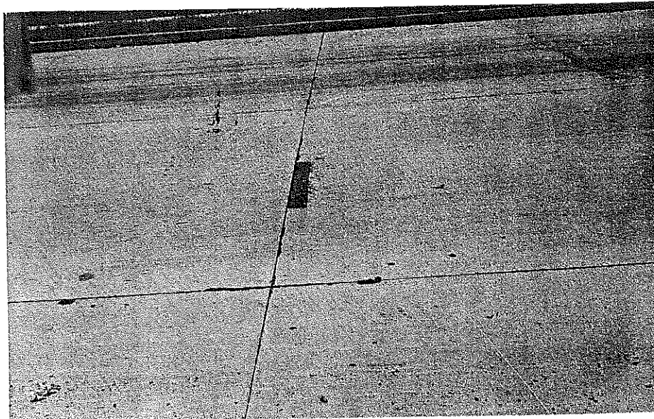
Fig. 5. Repaired Area at Station 59 + 75. Masonite divider wrapped in sheet polyethylene was used to maintain the joint; the divider has been removed but the polyethylene sheeting remains. The joint had not been sealed, 6-14-62.
