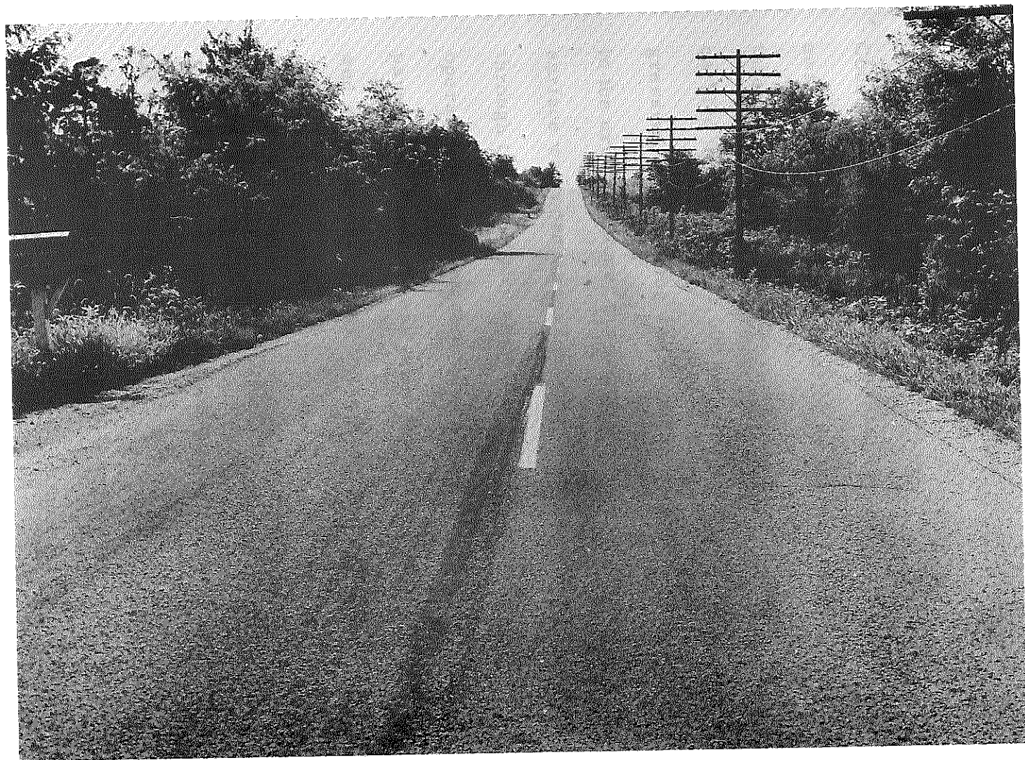
Fig. 7. Nelson County SP Group 31 Test Section after an Asphaltic Emulsion Seal Coat had been Placed (October 1961)
