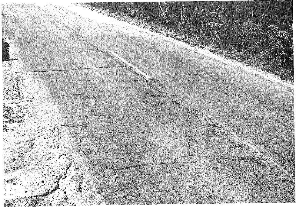
Fig. 5. Area of Transverse Cracking Near Station 370 of Nelson County SP Group 31 Test Section (Before Surfacing with Curtiss-Wright Binder)
