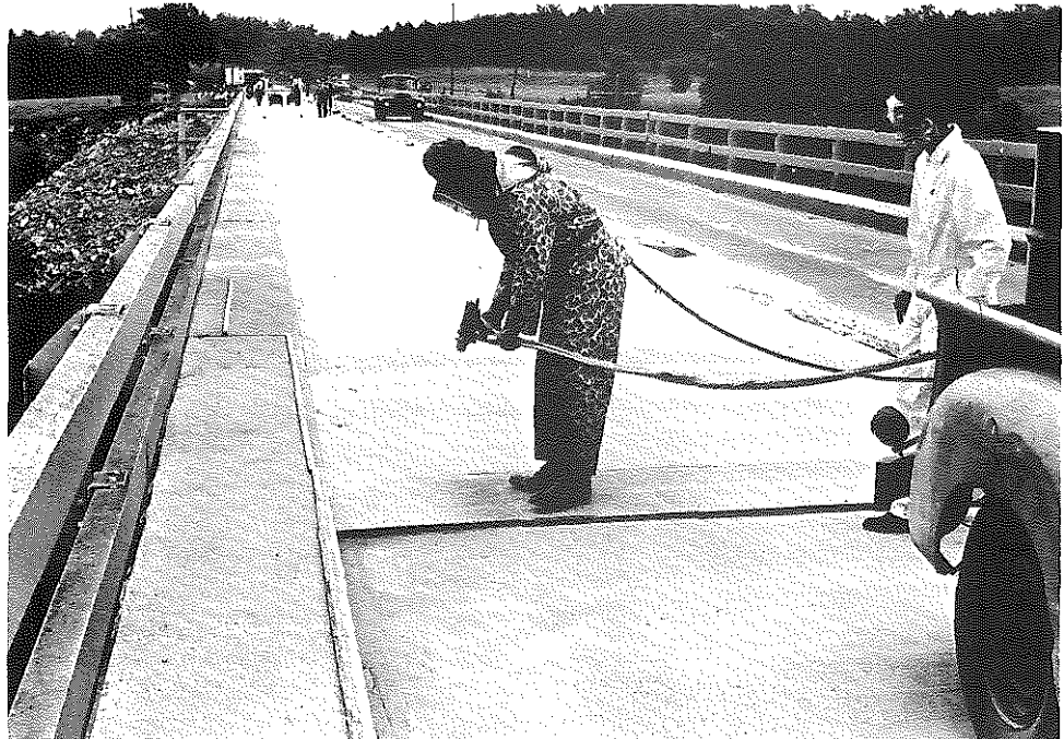
Fig. 98. Lake Cumberland Bridge; Westbound Lane, Facing East; Application of Epoxy Resin; Pyles Gun; Workman's Protective Suit Ventilated through Hose from Tanks of Compressed Breathing-air Carried in Truck. Wood laths were used as spacers to help gage application rate, July-August, 1962. Note: The latex mortar in this lane had been exposed to traffic through the winter sand blasting and other cleaning immediately preceded the application of epoxy.
