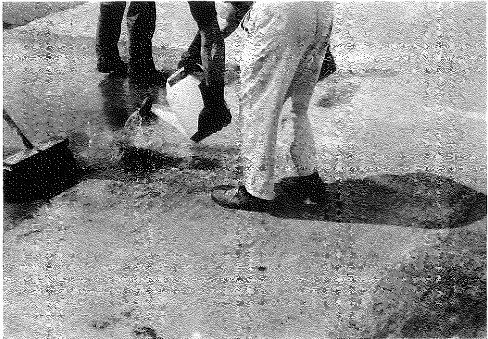
Fig. 70. Salt River Bridge, North-bound, Kentucky Turnpike; Acid Etching, Preparatory to Application of Epoxy-Tar Seal (Guardkote 140), August 24-25, 1960.
