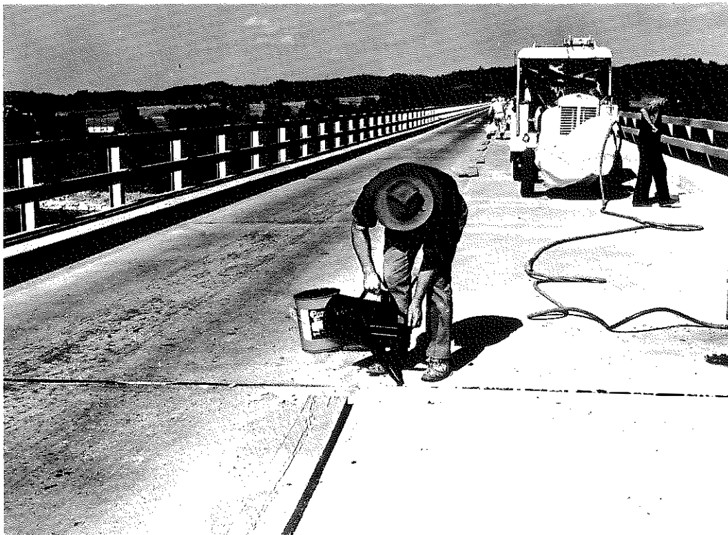
Fig. 94. Filling Joints with Prestite, No. 404, Pourable Joint Sealer (Two-Component, Polysulfide Rubber). Note: This material was later found to be reactive (de-polymerized, re-liquified) toward asphaltic materials. About 35 joints or portions thereof were reopened the following summer, 1962; sponge rubber inserts were installed in the joints to insulate new joint sealer from the asphaltic material below. The joints were repoured with the polysulfide compound.
