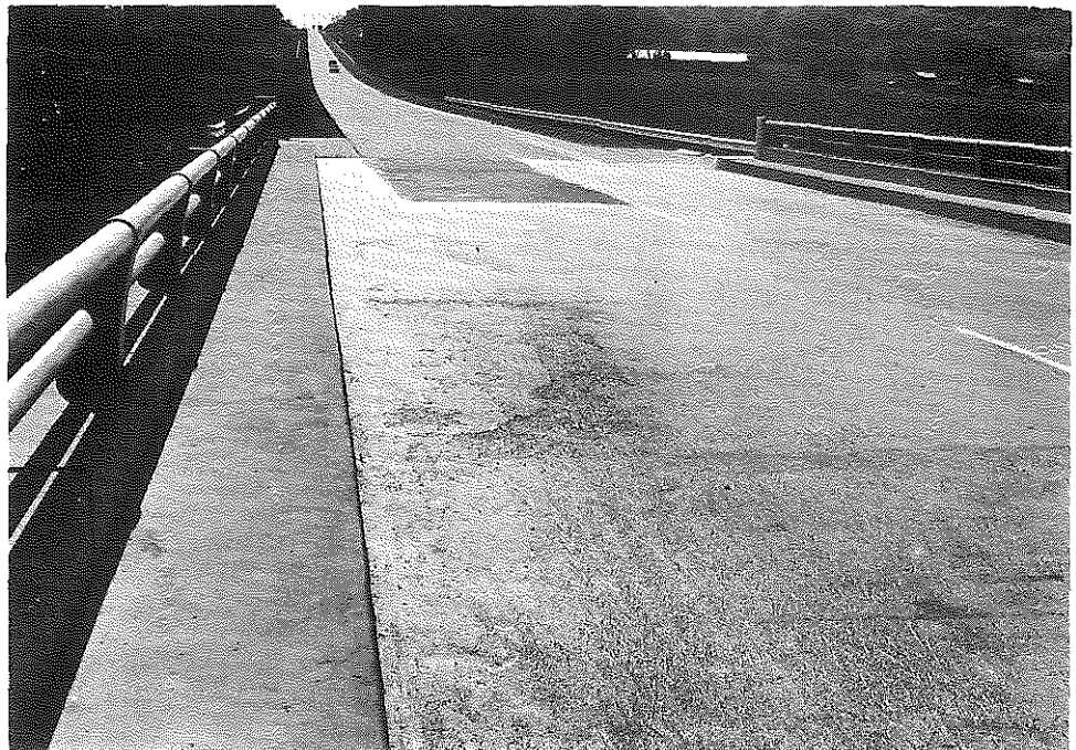
Fig. 108. South Benson Creek Bridge Above; Facing West; Guardian Chemical Company's Clear Bond (Styrene-Buladiene), Unfinished Here, Finished Later. Note scaling in left lane and transverse cracks conforming to construction joint and position of screeding templates.
