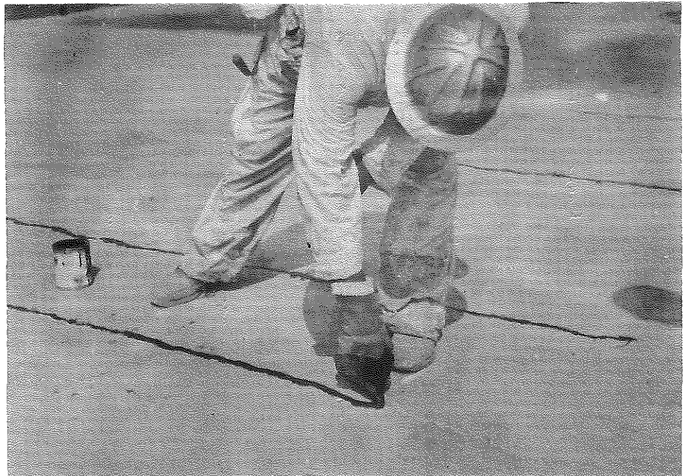
Fig. 54. Salt River Bridge, Kentucky Turnpike; Sealing Cracks with Furof Resin; Penntrowel Section.
