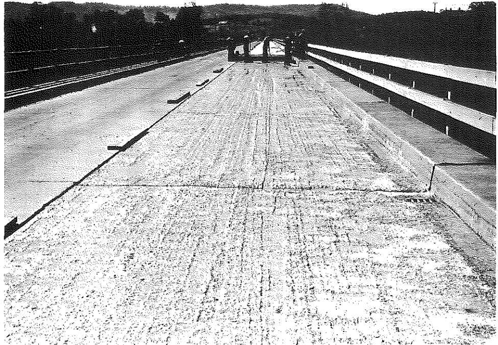
Fig. 90. Lake Cumberland Bridge, Facing West. Foreground shows routed and scarified deck; background shows application of mortar topping; extreme background shows polyethylene curing-blanket. Left lane (eastbound) shows mortar overlay after curing and after epoxy-sand seal, open to traffic.
