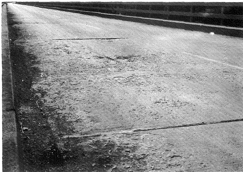
Fig. 84. Close-up View of Deck, Lake Cumberland Bridge. Note raveling and debris in gutter, 6-61.
