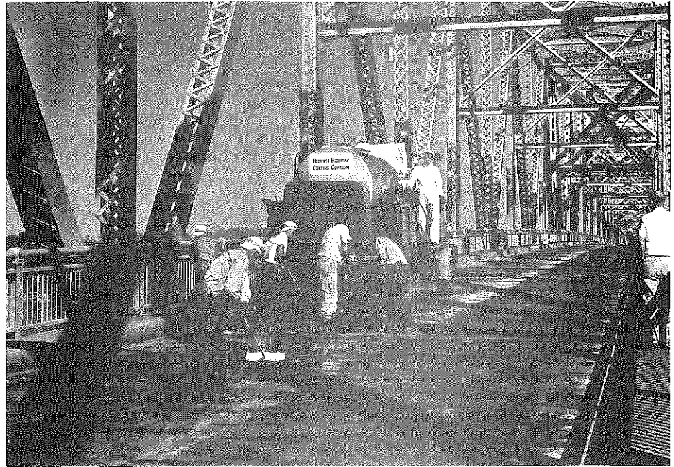
Fig. 113. Owensboro Bridge (Ohio River); Facing North; Showing Application of Acid and Scrubbing. This treatment was preceded by washing with detergents.
