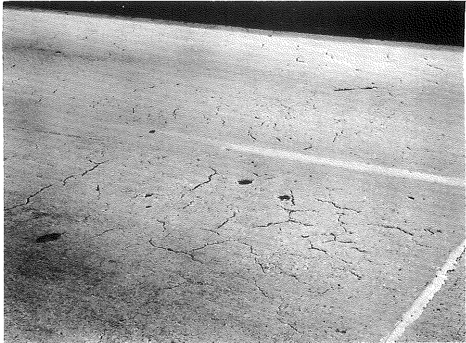
Fig. 131. Clays Ferry Bridge. Close-up view of impending failure of deck, near south end of bridge.
