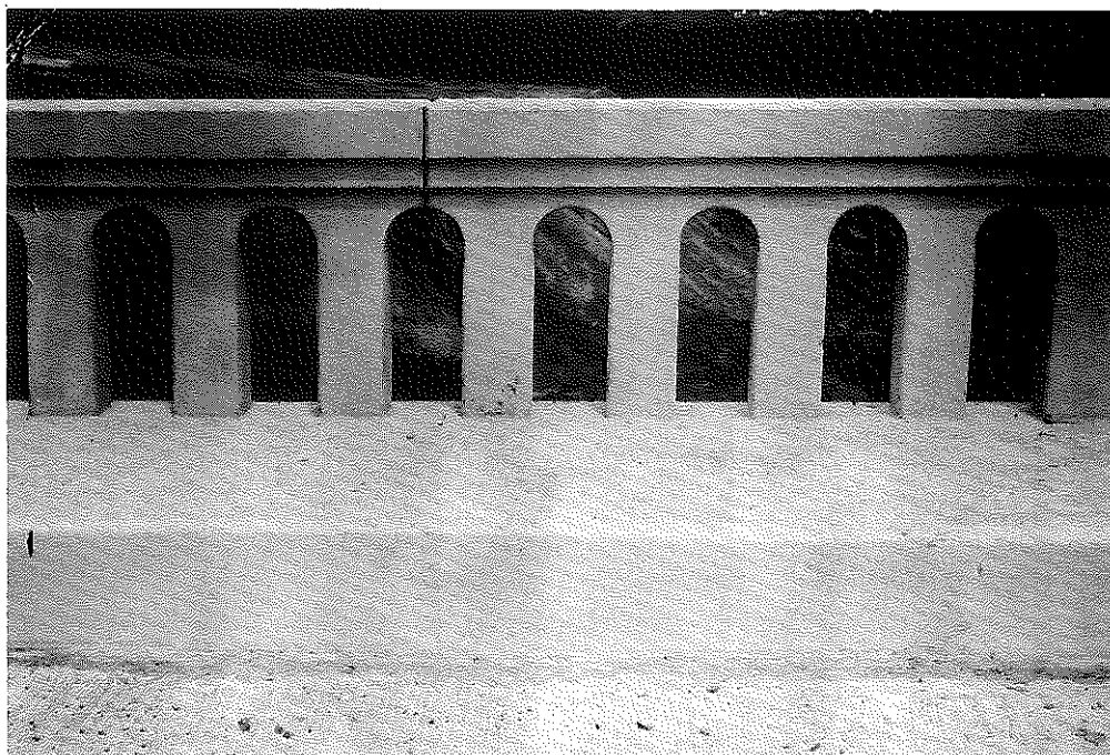
Fig. 8. Levisa Fork Bridge. Cracks patched with Relcote 60 (epoxy) and sand (Ref.: "The Use of Epoxy Resin for Sealing Cracks in a Reinforced Concrete Bridge," by Milton Evans, Jr., July, 1959; RHMRL, Vol. XIV, p. 311).
