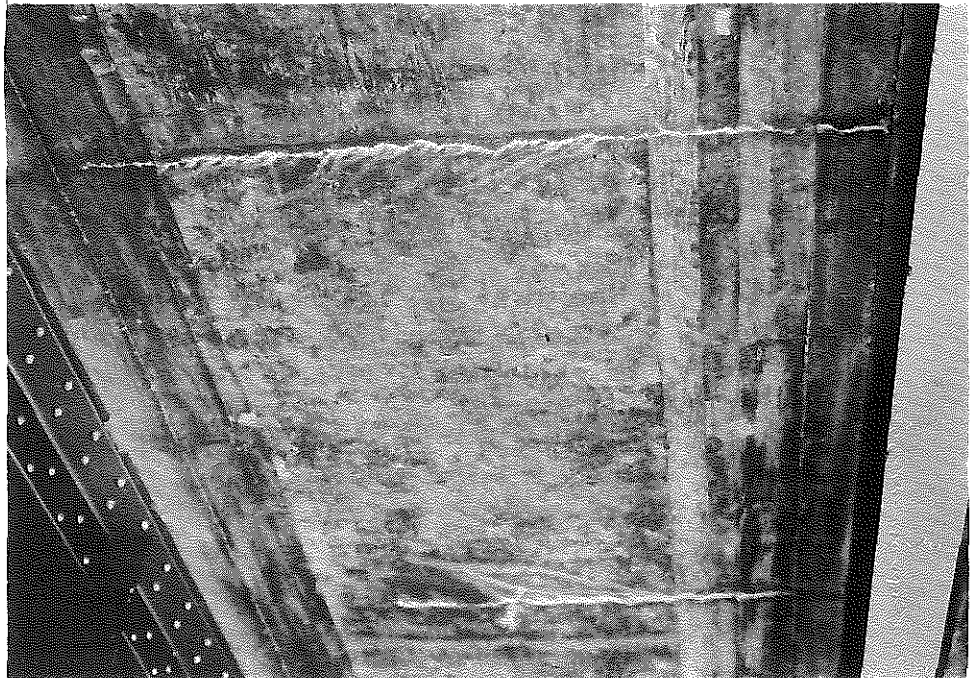
Fig. 42. Salt River Bridge, Kentucky Turnpike; Transverse Cracks, Underneath Side of Deck, Showing Deposits of Salt.
