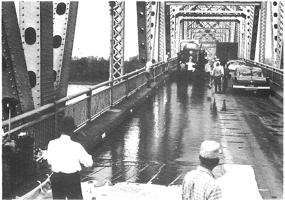
Fig. 116. Owensboro Bridge; Application of Resiweld Guardkote 140 (H. B. Fuller Company), Through Mixing Distributor; Application Rate, 3.3 Lbs. Per Sq. Yd. Note polyethylene sheet in foreground (for starting), followed immediately by application of sand.
