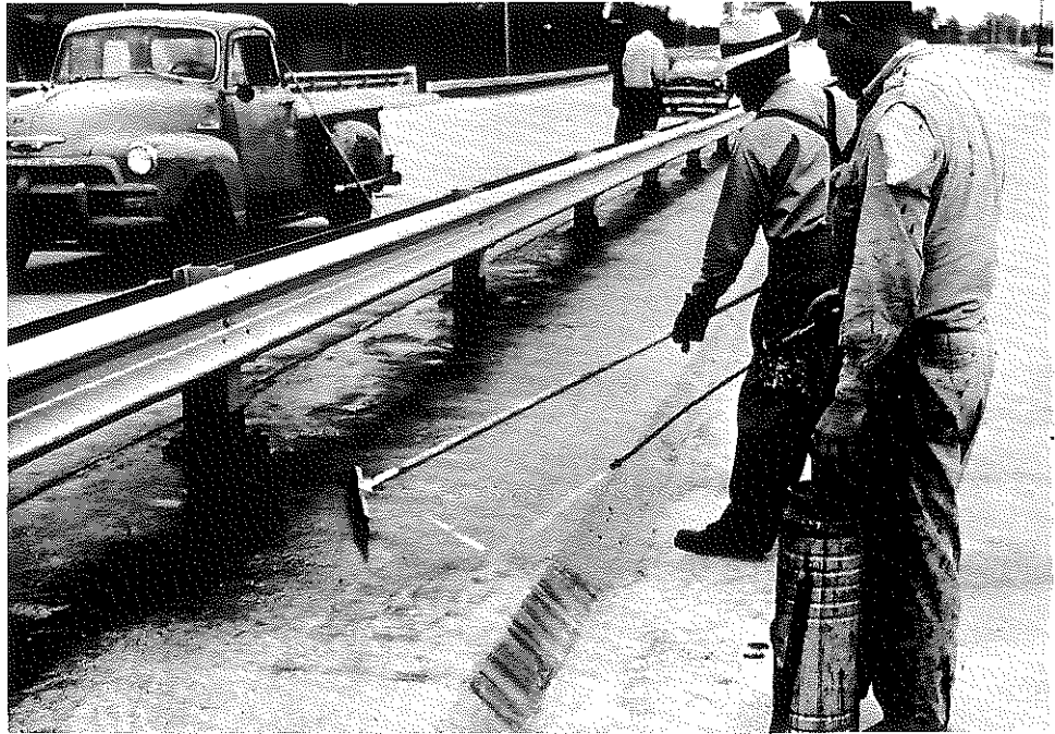
Fig. 35. St. Catherine's Street Bridge, Application of Polystyrene. Penetrant to Median Curb; Southbound Lanes, Looking South.
