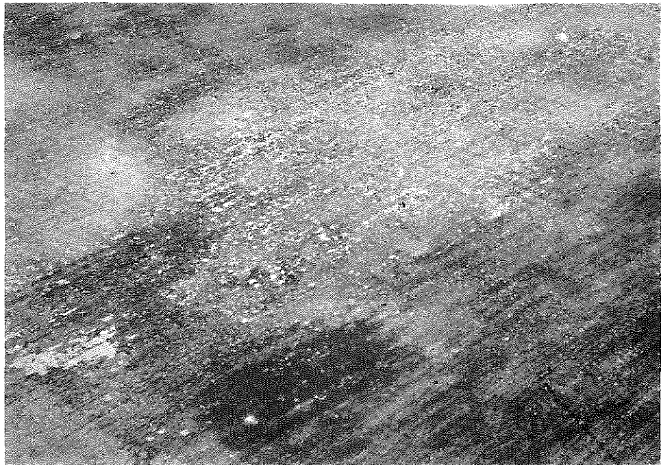
Fig. 49. Salt River Bridges, Kentucky Turnpike; Epoxide-Alkyd Coating, after One Winter.
