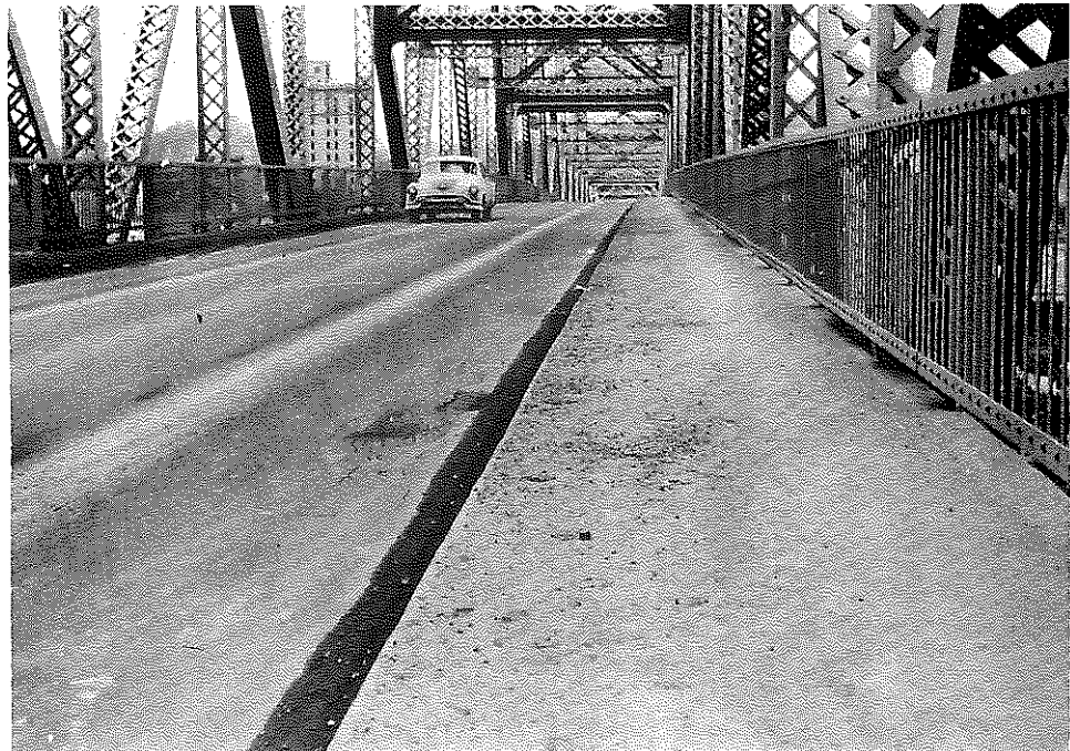
Fig. 34. Ashland-Coal Grove Bridge, March 1960. Note Cinders in gutter and distressed area in outer wheel track.
