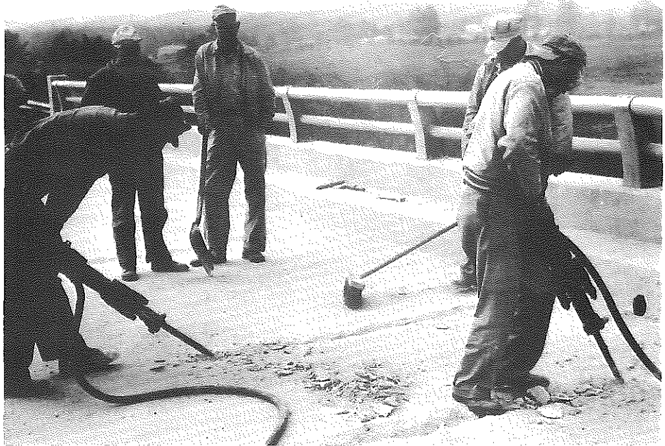
Fig. 58. Salt River Bridges, Kentucky Turnpike; Deep-Routing Transverse Cracks, Preparatory to Placing Latex-Mortar Overlay, October, 1960.
