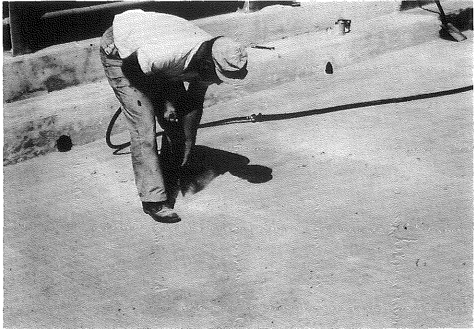
Fig. 53. Salt River Bridge, Kentucky Turnpike; Chipping Cracks, Preparatory to Sealing Them; Penntrowel Section, 8-31-60.
