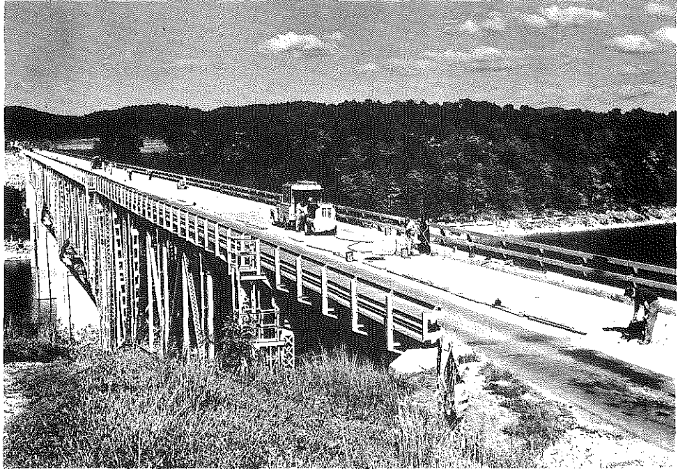
Fig. 92. Lake Cumberland Bridge, Over-all View, Facing East, Showing Joint-Sealing Operations in Eastbound Lane.
