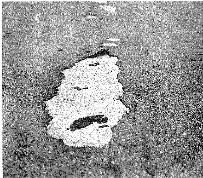
Fig. 69. Salt River Bridge, Kentucky Turnpike; American Bitumuls Heavy Duty Resurfacer; Showing Peeling During First Winter.
