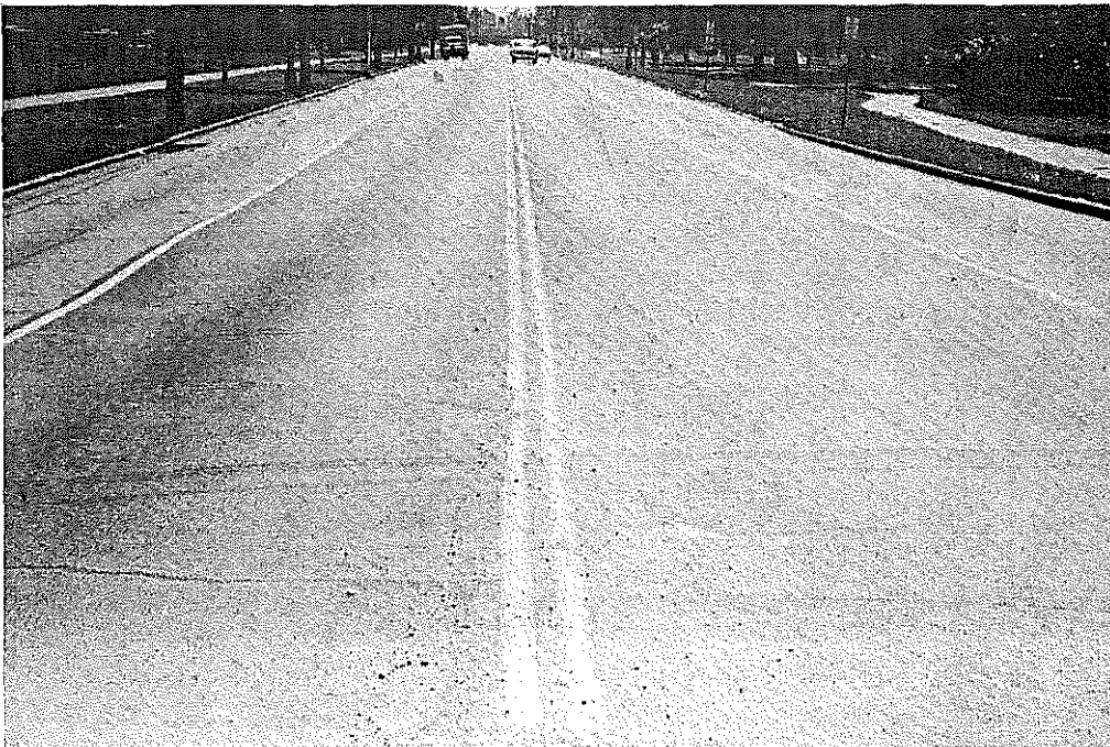
Fig. 15. South Third Street, Louisville. The seal contains silica sand from near Mt. Vernon. Only the two center lanes have been sealed. Note the shrinkage cracks in the old surface.
