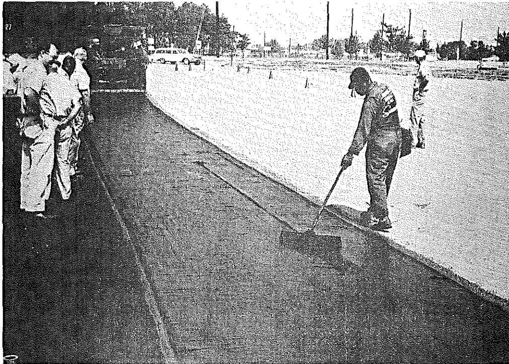
Fig. 4. Kentucky State Fairgrounds. The laborer is smoothing a streak caused by an over-sized aggregate particle. The dark stripe next to the fresh slurry is water from the spray-bar beneath the slurry machine.
