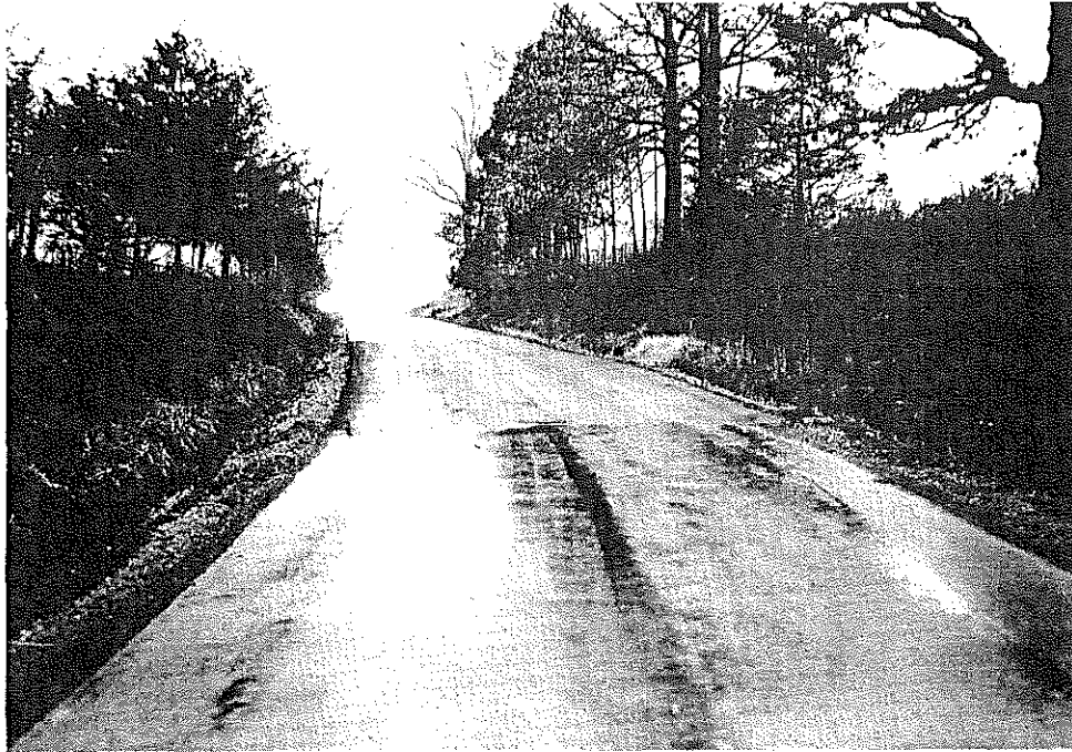
Fig. 7. Large Failed Area in a Cut-Section. The failure occurred during the winter of 1961-62. The surface contains 6.5 percent asphalt (1-7-63).
