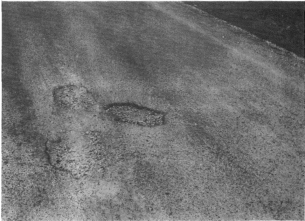
Fig. 13. RS 24-655-1. Potholes Formed in a Low, Wet Area, April 11, 1963.
