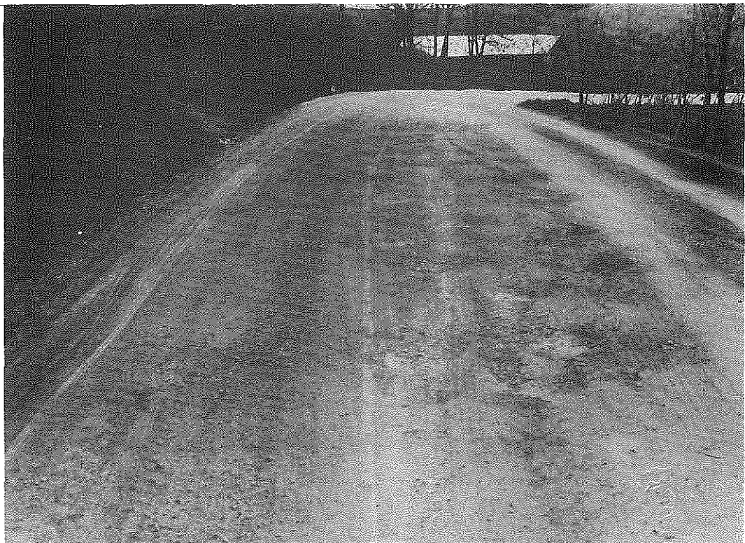
Fig. 6. RS 32-189. Condition of Roadway at the Crest of a Rise, April 23, 1963.
