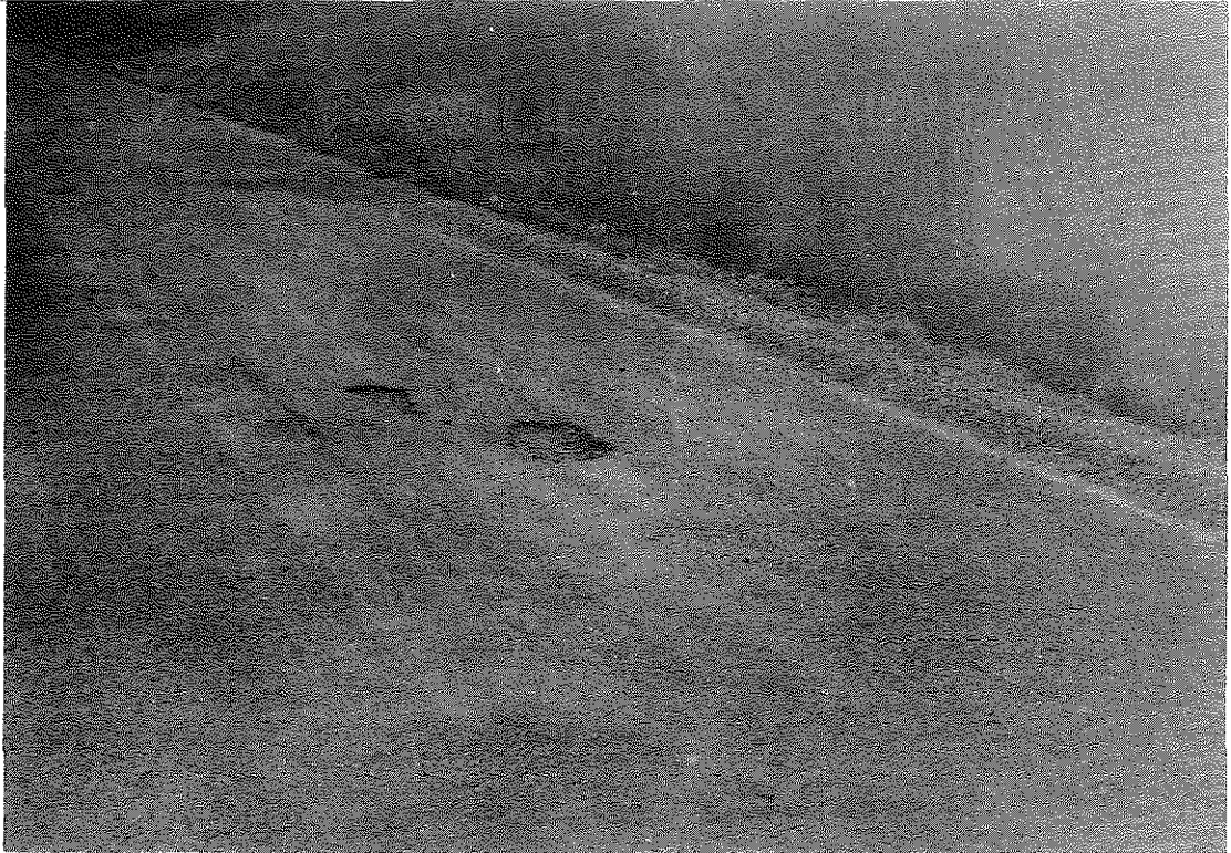
Fig. 11. RS 2-415. Condition of Roadway in Poor Drainage Area, April 11, 1963.
