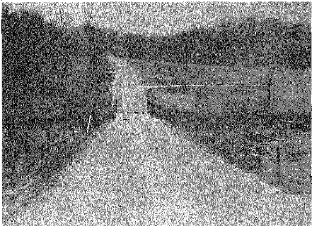
Fig. 14. RS 24-655-1. Condition of Roadway on April 11, 1963. The eastern portion of the project is in the background.
