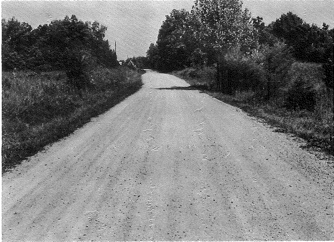
Fig. 1. RS 100-635. Condition of Roadway on August 16, 1962.
