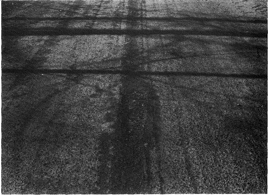
Fig. 7. RS 100-635. Condition of Roadway in a Low Area, January 22, 1963.
