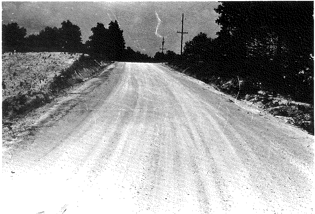
Fig. 8. RS 24-655-1. Condition of Western Part of Project, July 30, 1962.
