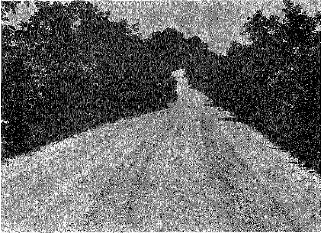
Fig. 1. RS 32-189. Condition of Roadway on July 10, 1962.
