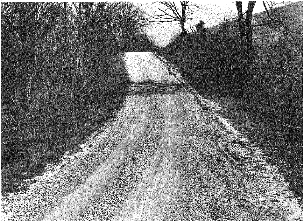
Fig. 2. MP 87-377. Poor Drainage Condition on Northern Portion of Roadway, April 10, 1963.
