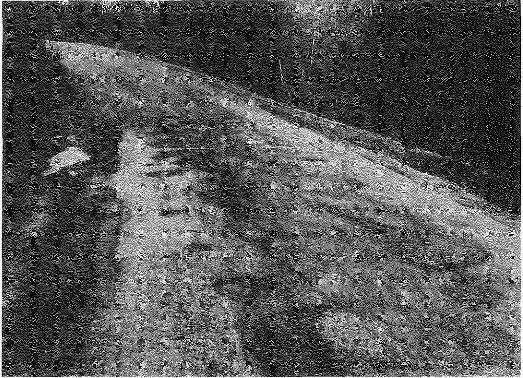
Fig. 7. RS 32-189. Soft Area in Roadway, April 23, 1963.
