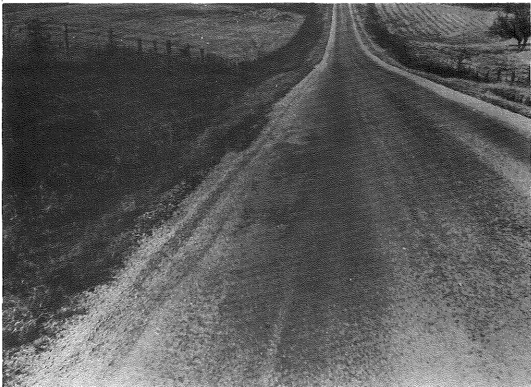
Fig. 6. RS 40-326. Distressed Area in Outside Wheel Track of Roadway, December 27, 1962.
