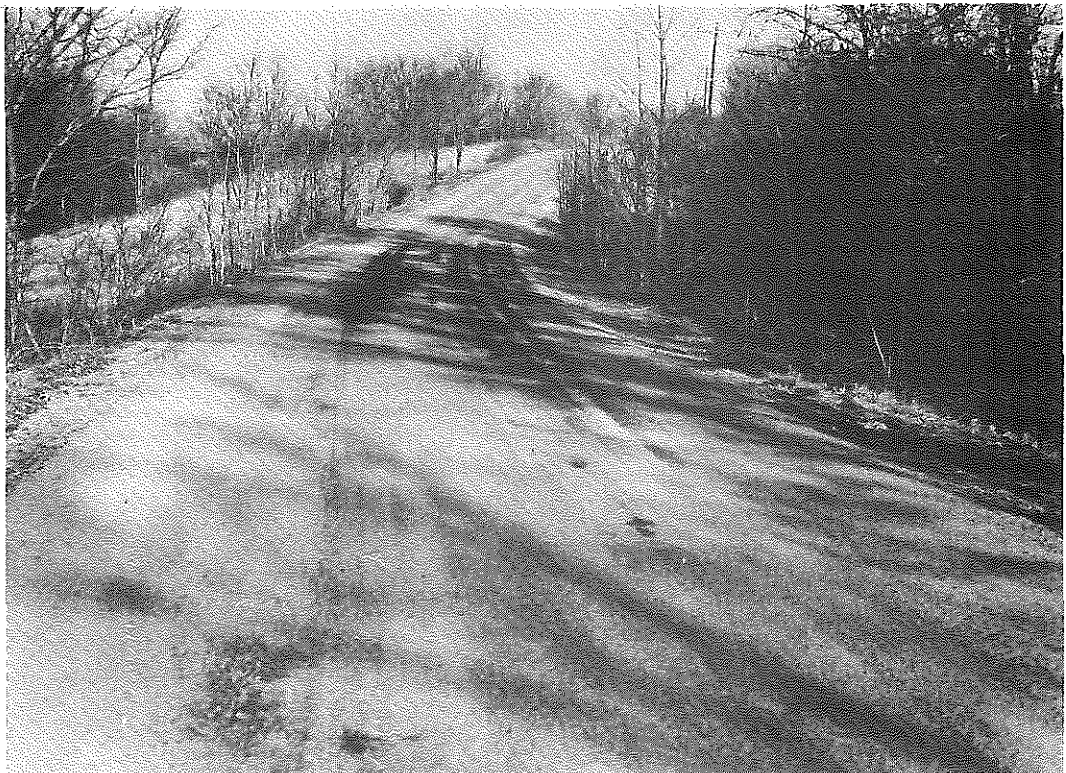
Fig. 12. RS 24-655-1. Photograph Showing Wet Area, December 19, 1962.
