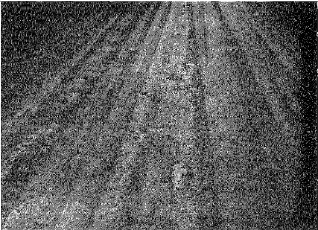
Fig. 6. RS 2-415. Potholed Condition of Compacted Roadway after a Rain Shower, July, 1962.
