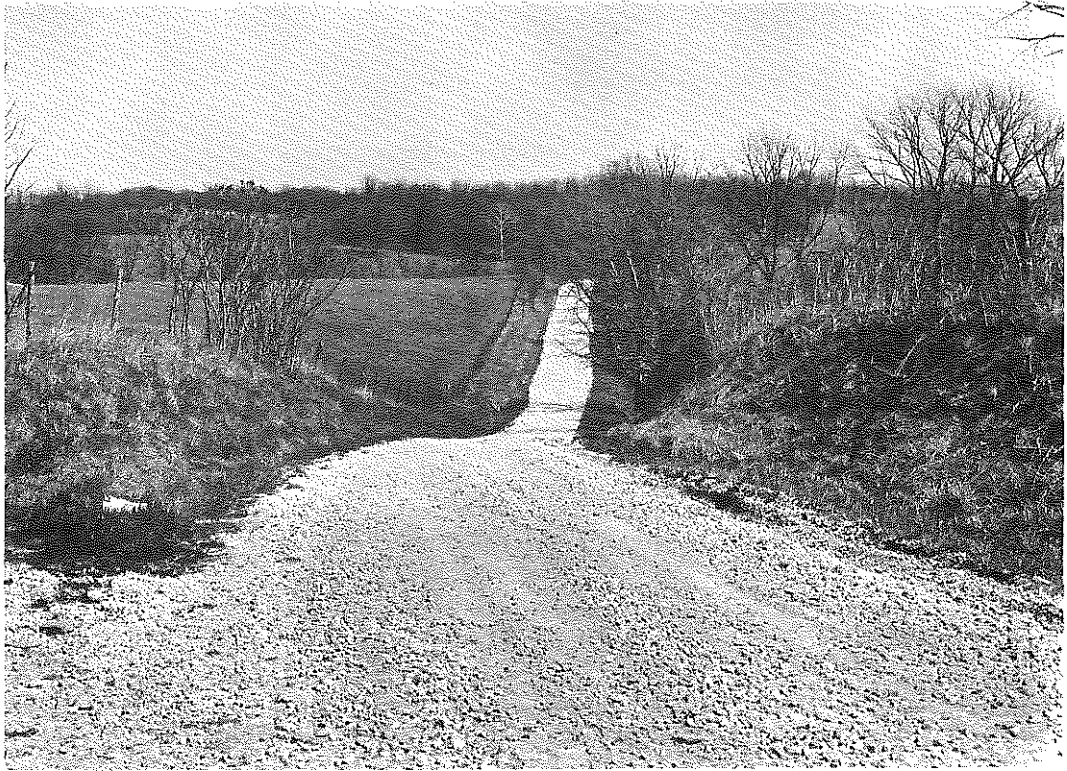
Fig. 3. MP 87-377. Northern Portion of Roadway on April 10, 1963. Note soft area on the right of the road.
