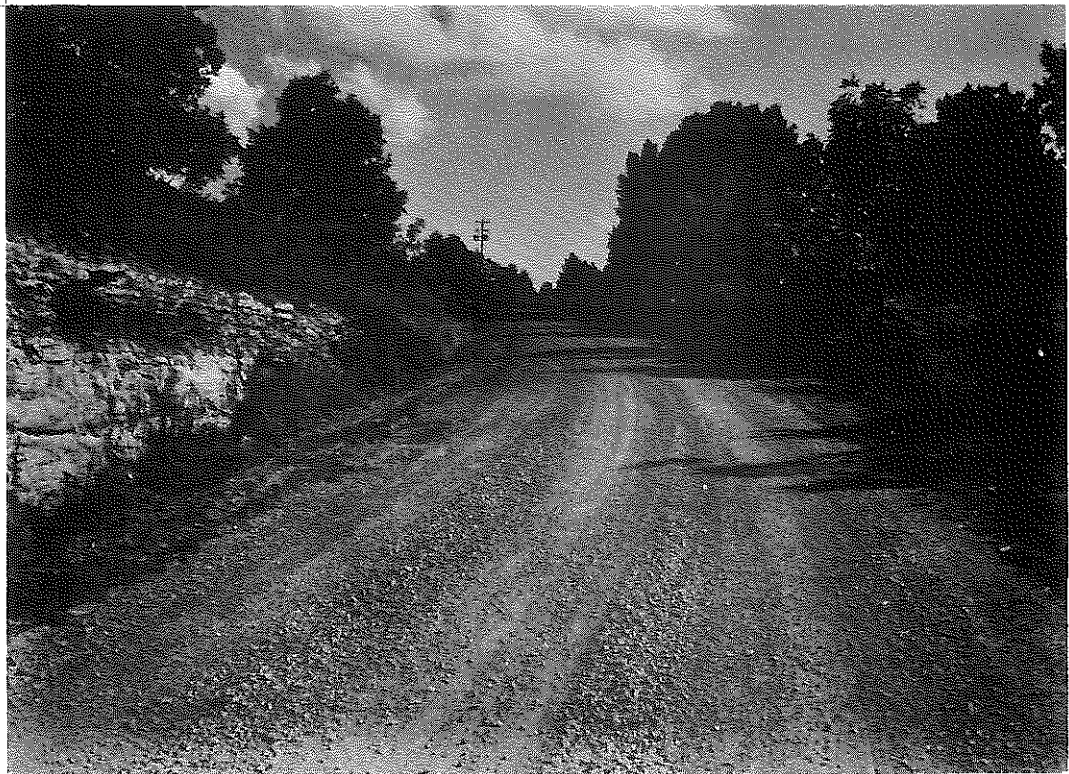
Fig. 8. RS 2-415. Photograph Showing Difference in Raveling in Treated and Untreated Base, August 8, 1962.
