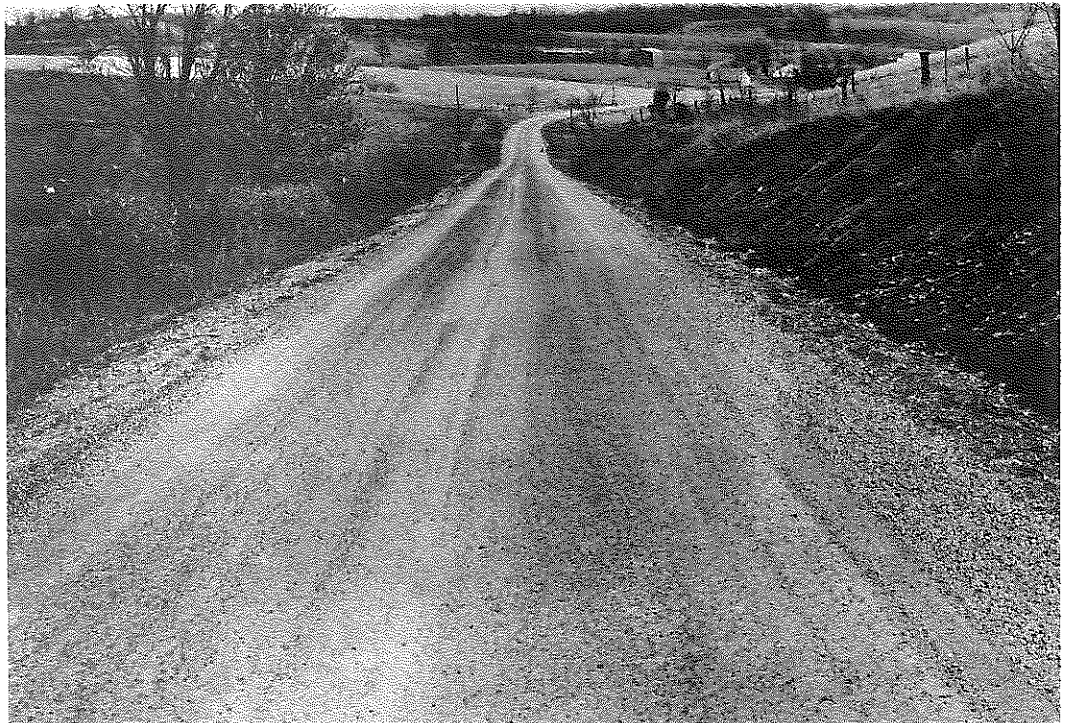
Fig. 8. RS 35-750. Condition of Roadway on April 23, 1963.
