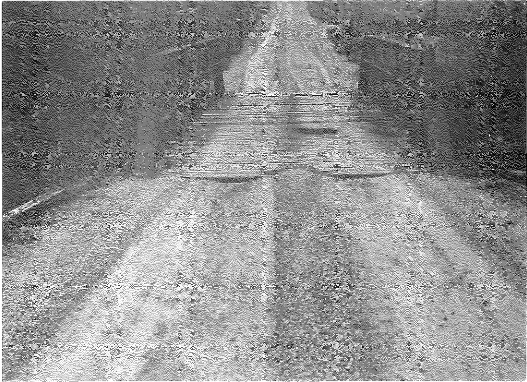
Fig. 9. RS 24-655-1. Condition of Eastern Portion of Project, September 25, 1962.
