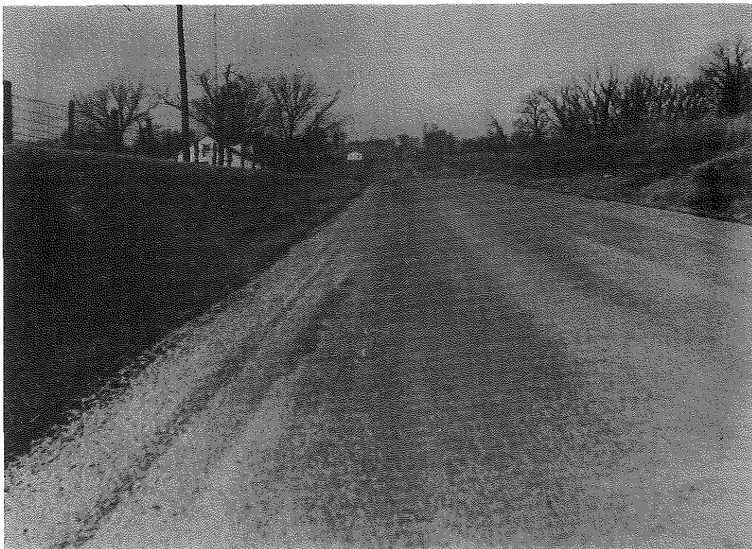
Fig. 4. RS 40-326. Condition of Roadway on December 27, 1962.
