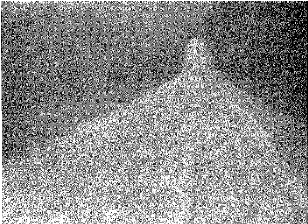
Fig. 10. RS 24-655-1. Condition of Eastern Portion of Project, September 25, 1962.
