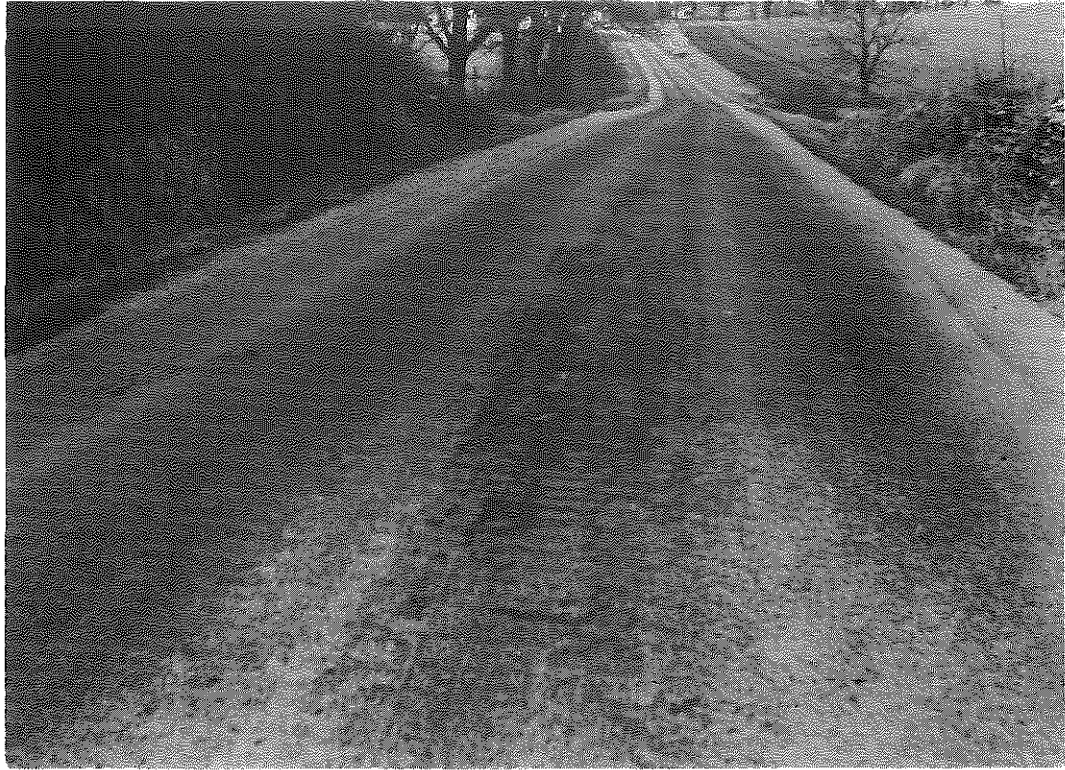
Fig. 5. RS 40-326. Distressed Area in Center of the Roadway, December 27, 1962.
