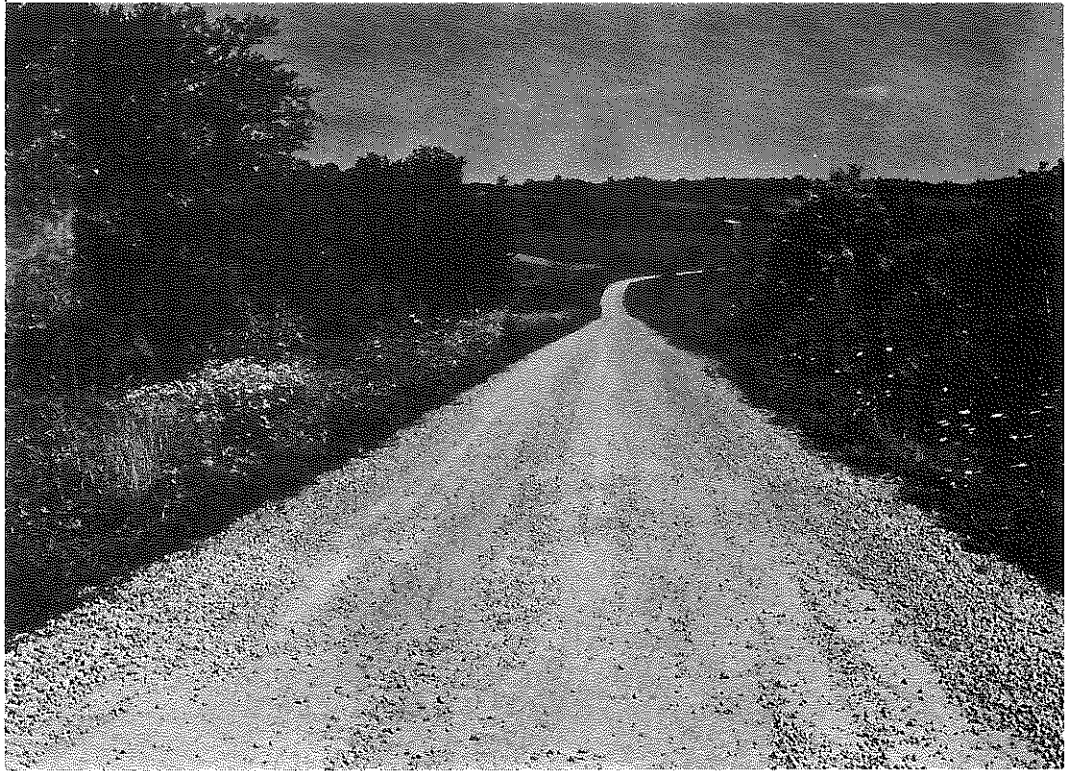
Fig. 1. RS 35-750. Condition of Roadway on July 10, 1962.
