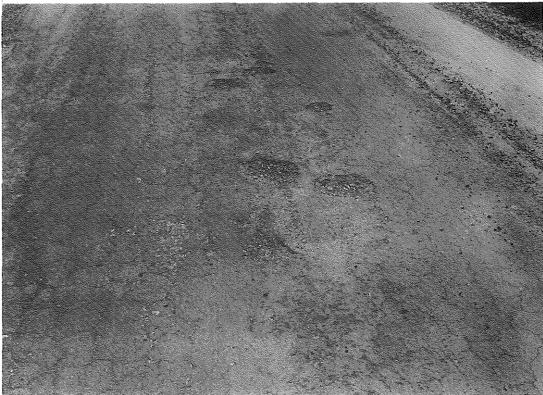
Fig. 10. RS 95-376. Potholes and Map Cracks on Roadway, April 15, 1963.
