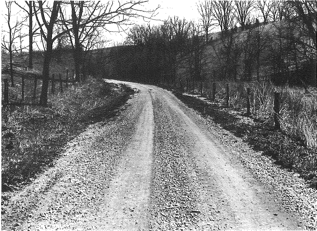
Fig. 1. MP 87-377. Poor Drainage Area on Southern Portion of Roadway, April 10, 1963.
