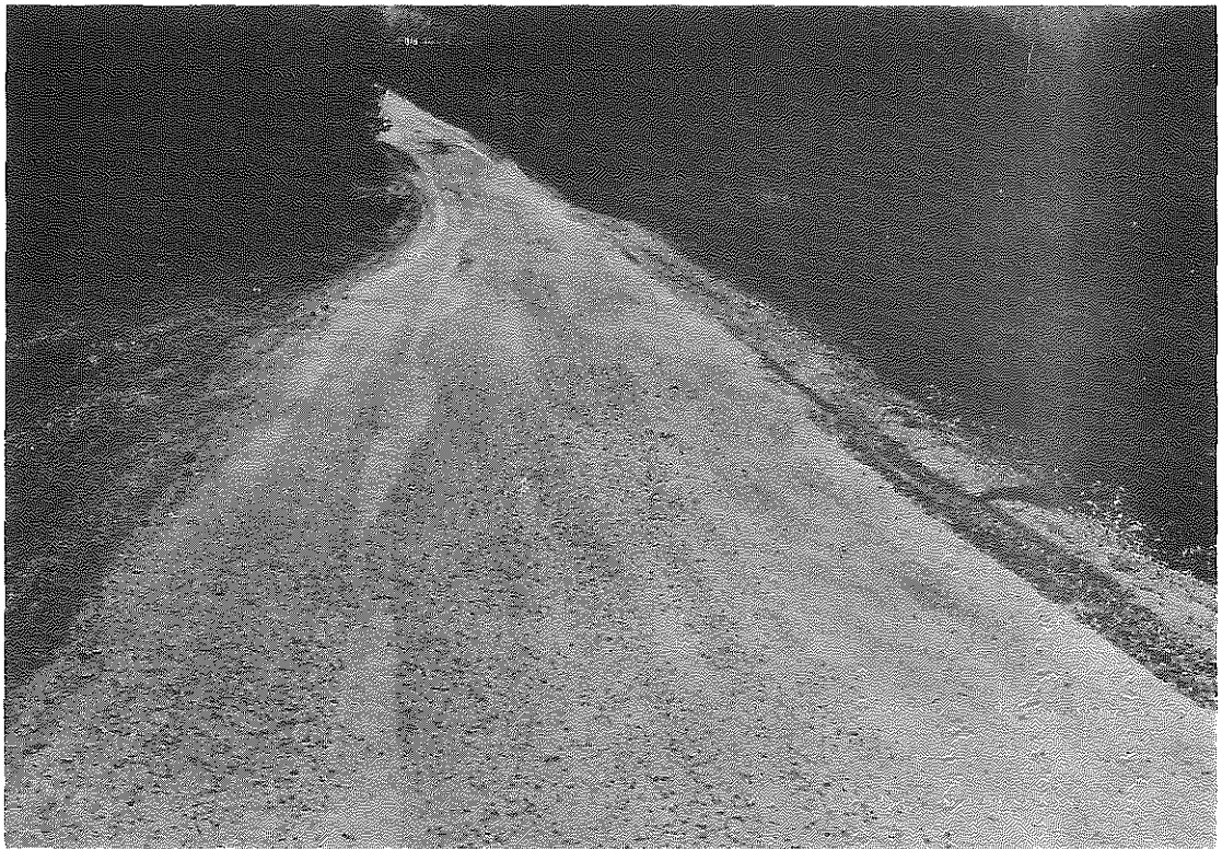
Fig. 9. RS 32-189. Condition of Roadway After Blading, April 23, 1963.
