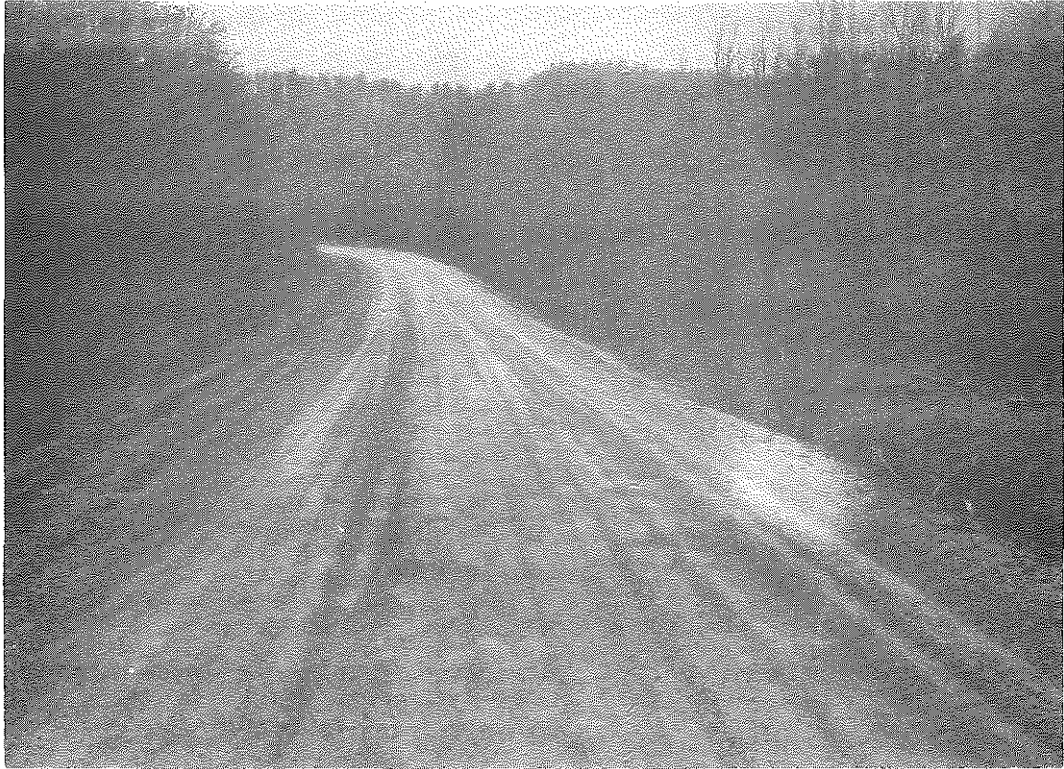
Fig. 5. RS 65-549. Condition of Roadway on April 15, 1963.
