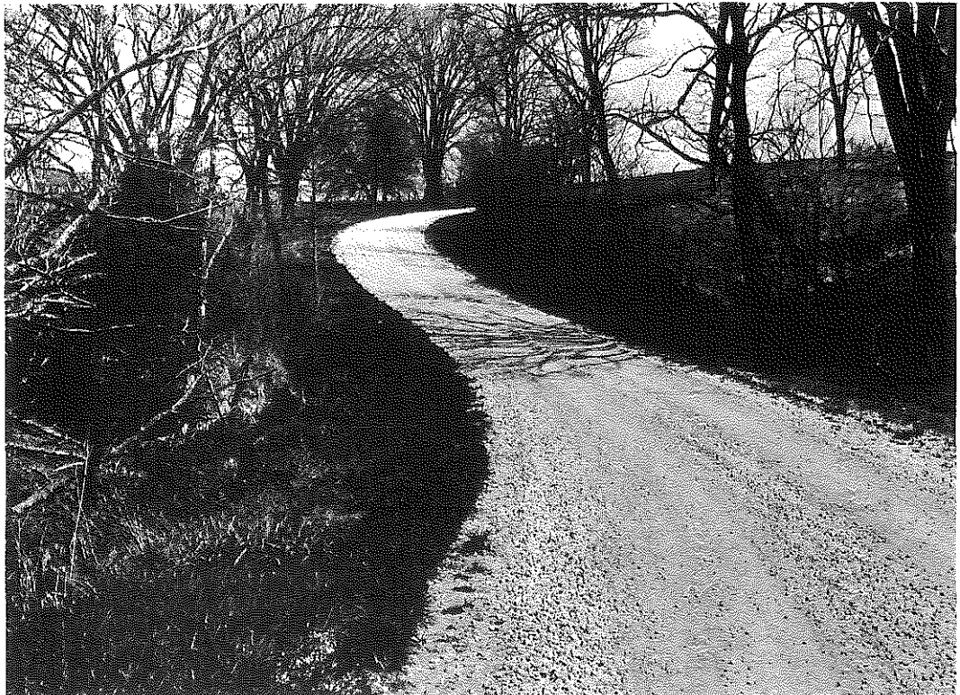
Fig. 4. MP 87-377. Condition of Southern Portion of Roadway on April 10, 1963.
