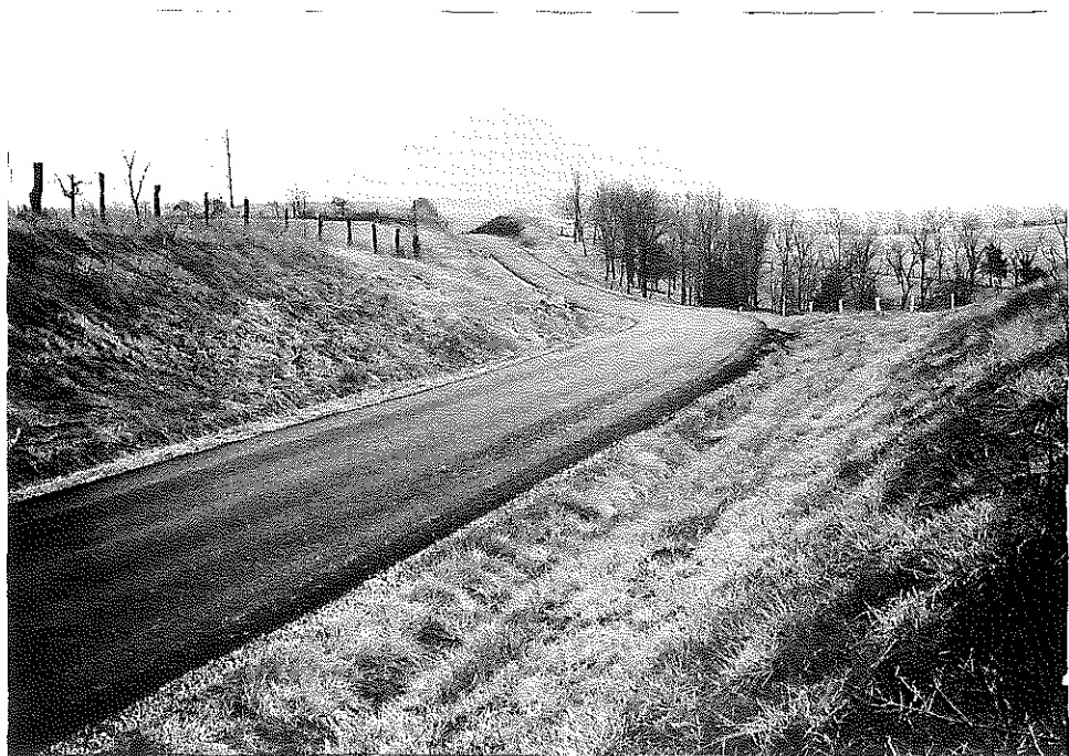
Fig. 2. RS 40-326. Area of Distress in Outside Wheel Track of Roadway, February 13, 1962.
