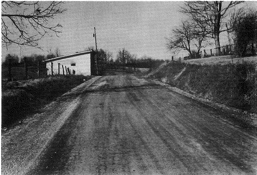
Fig. 8. RS 95-376. Roadway Condition at South End of Project on February 6, 1963.
