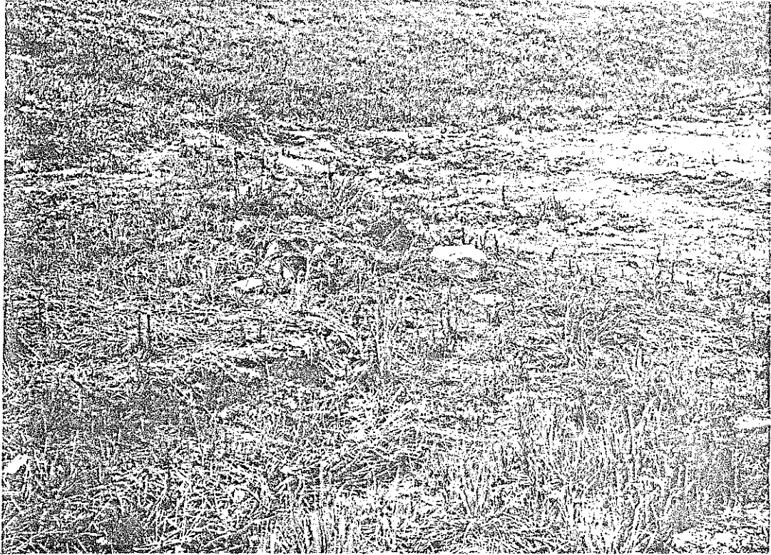
Fig. 24. Wet Area at Toe of Embankment Showing Slight Soil Flow, April 25, 1963.
