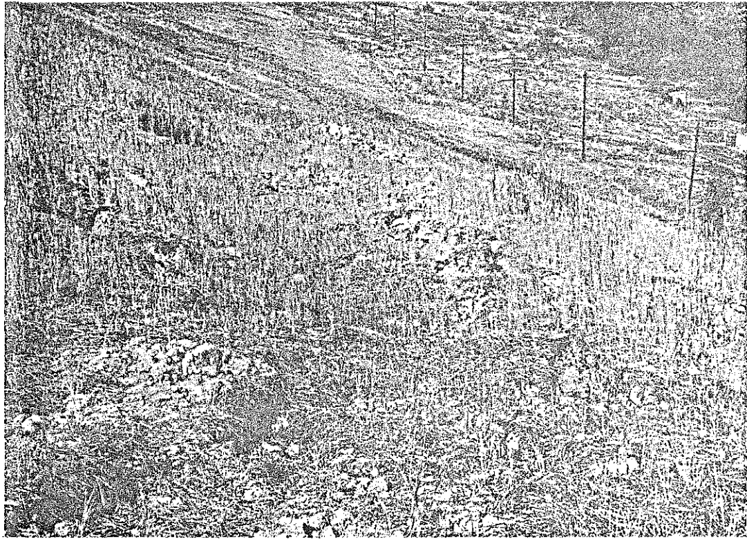
Fig. 38. Transverse Cracks and Ridges on Embankment Slope, May 10, 1963 (Looking North).
