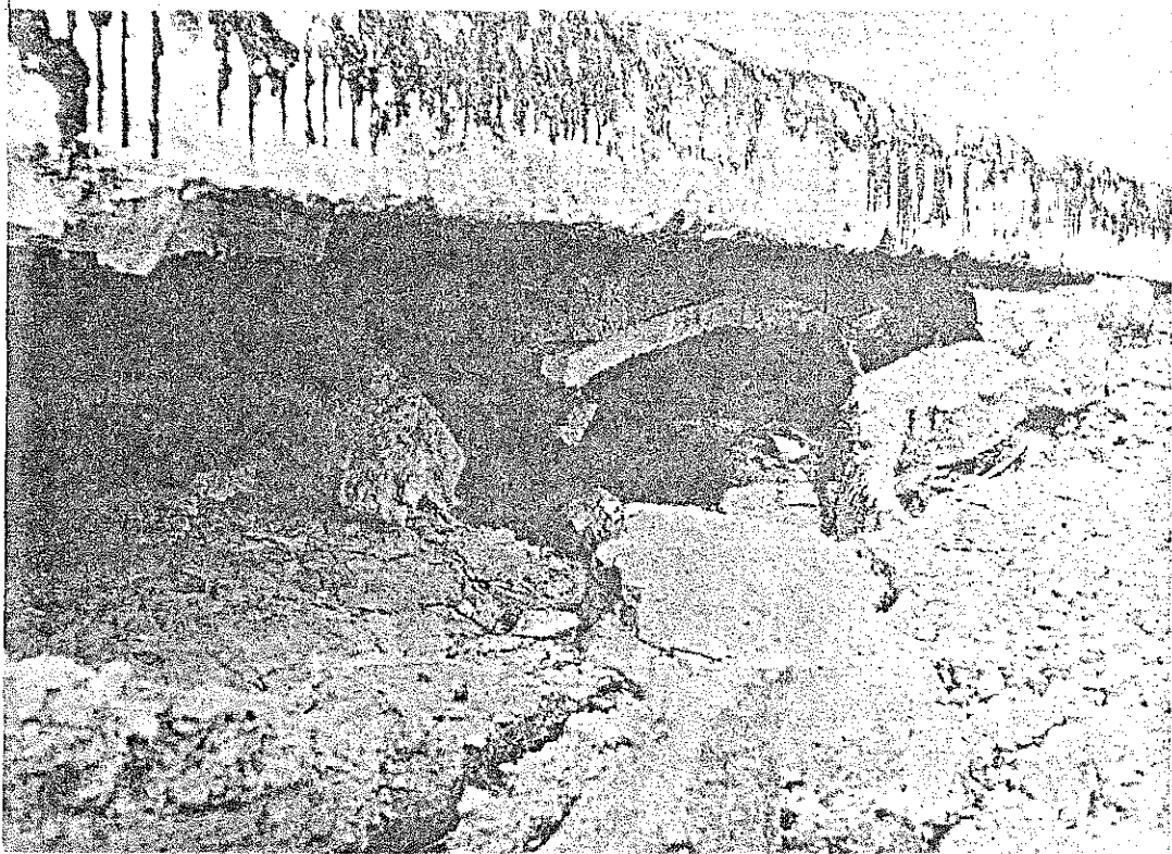
Fig. 33. Layers of Old Cement Grout and Mudjacking Material, May 10, 1963.
