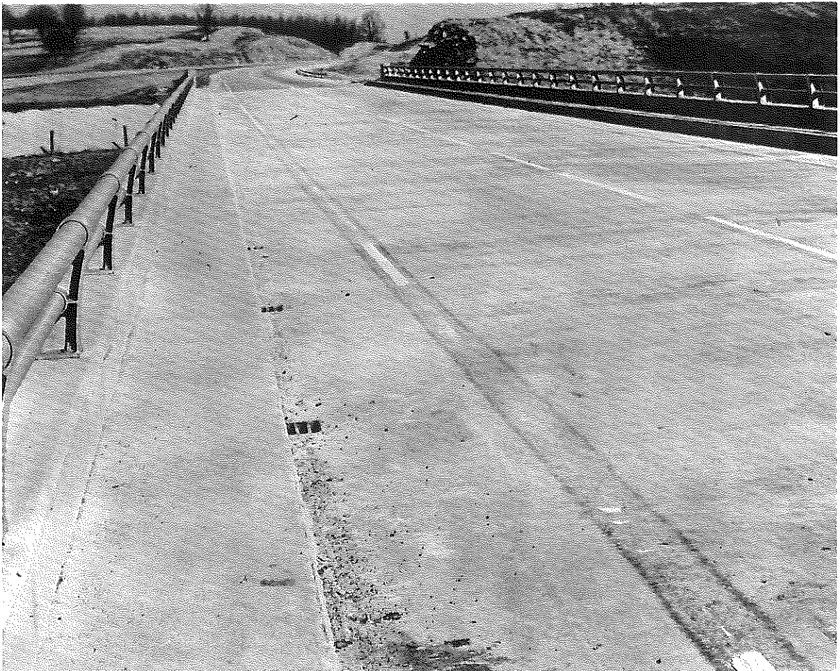
Figure 13: View of Concrete Bridge Deck, I 64, Clark - Montgomery Counties, Showing Spalled and Missing Portions of Plastic Edge-line (Catatherm Subsection). The darkened portion along the edge-line in the foreground indicates a heavy application of bonding primer. This line was placed in November 1962, and the photograph was taken in February 1963.
